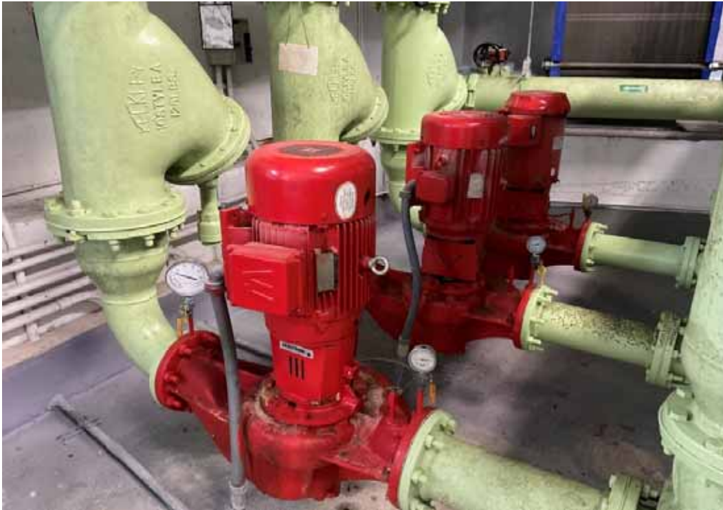
A/C Condensing Pumps - Open Loop
