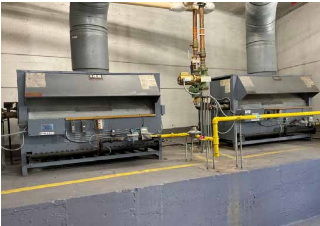
Boilers - Domestic Water
