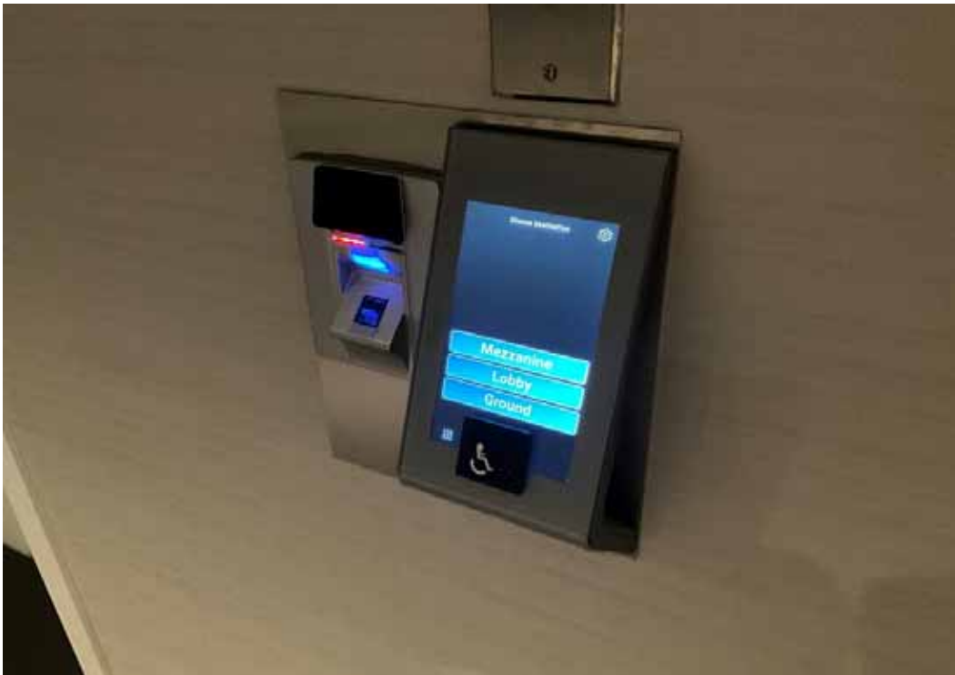
Card & Biometric Reader - Elevator Lobby
