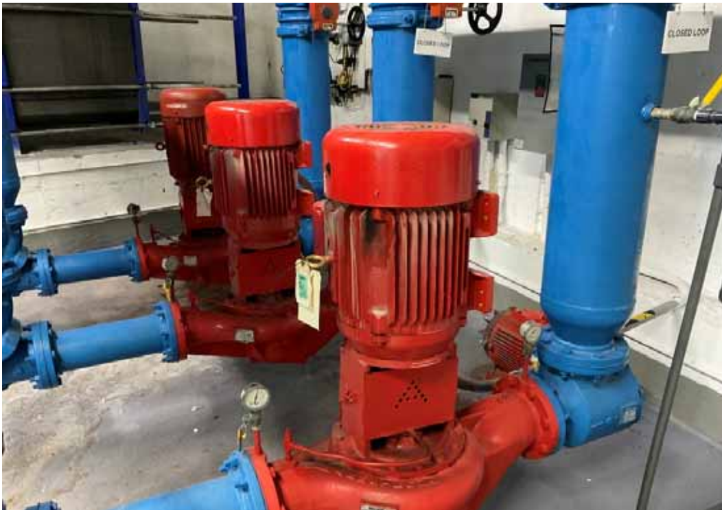
A/C Condensing Pumps - Closed Loop
