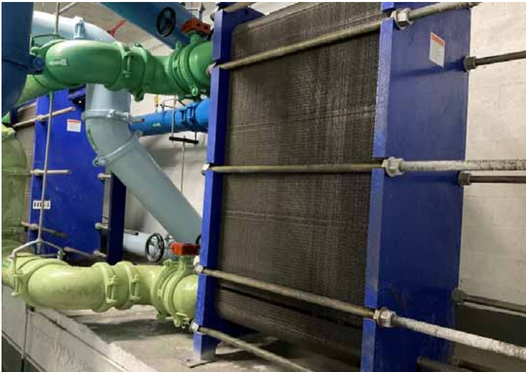
A/C Heat Exchangers
