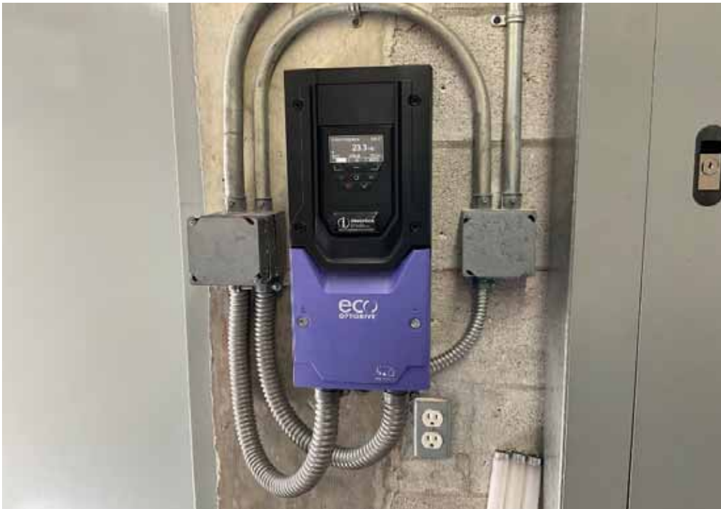
Var Freq Drive - Supply Fan
