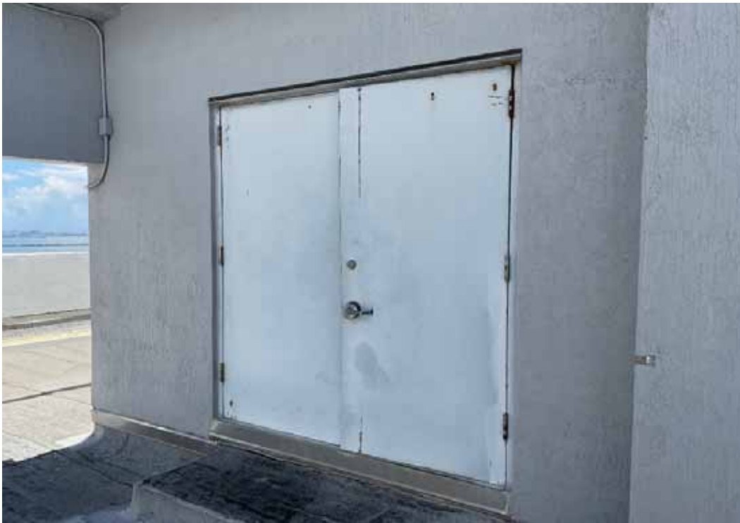
Doors - Roof Communication Room
