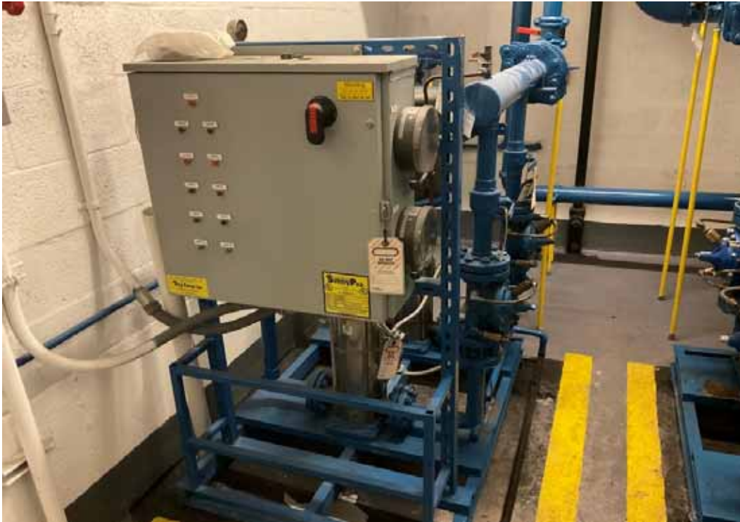
A/C Cooling Tower Drain Pump System
