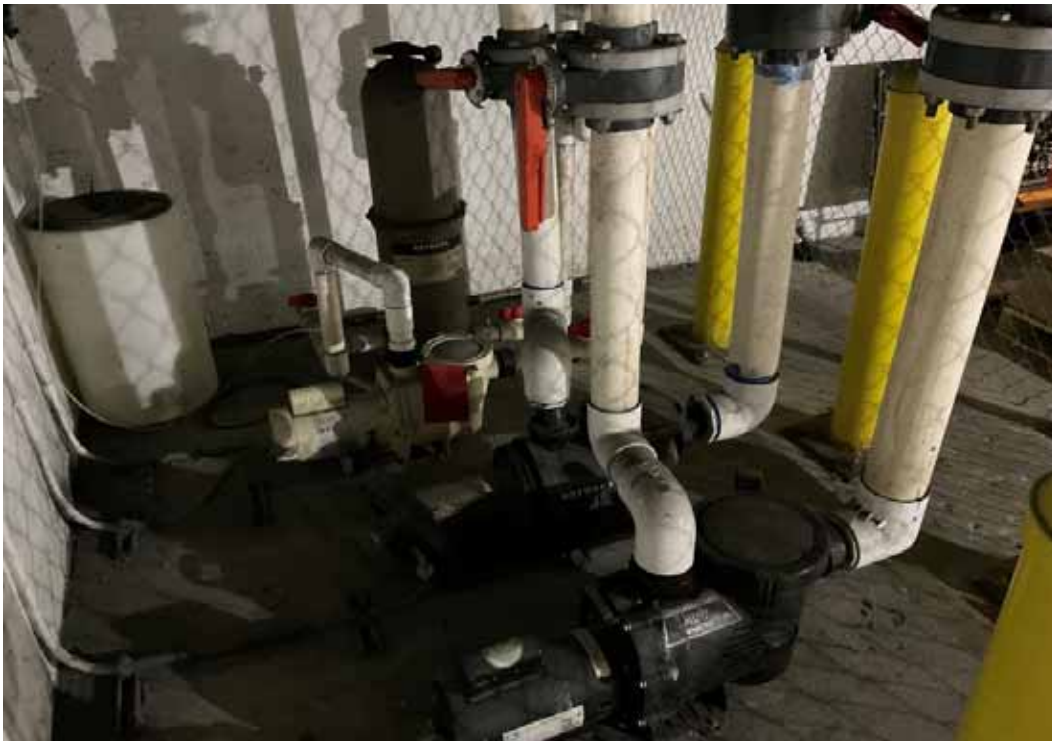
Lobby Fountain Equipment
