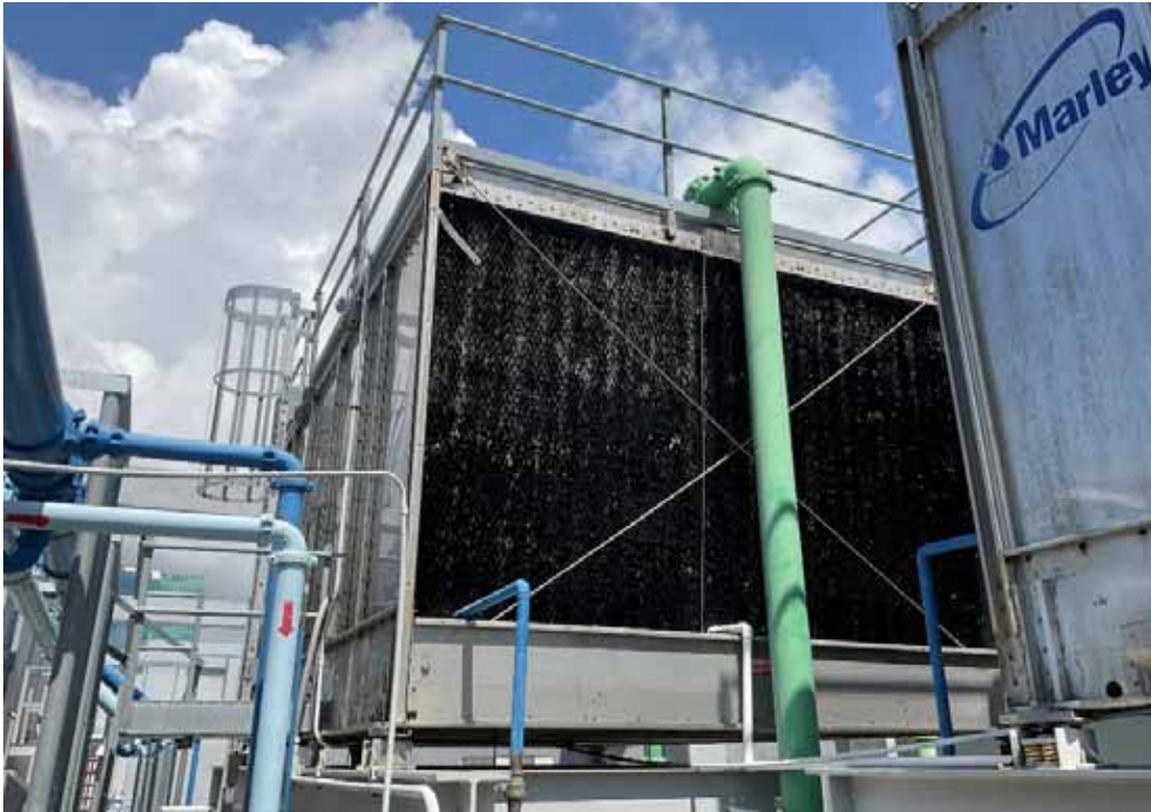
A/C Cooling Tower #2
