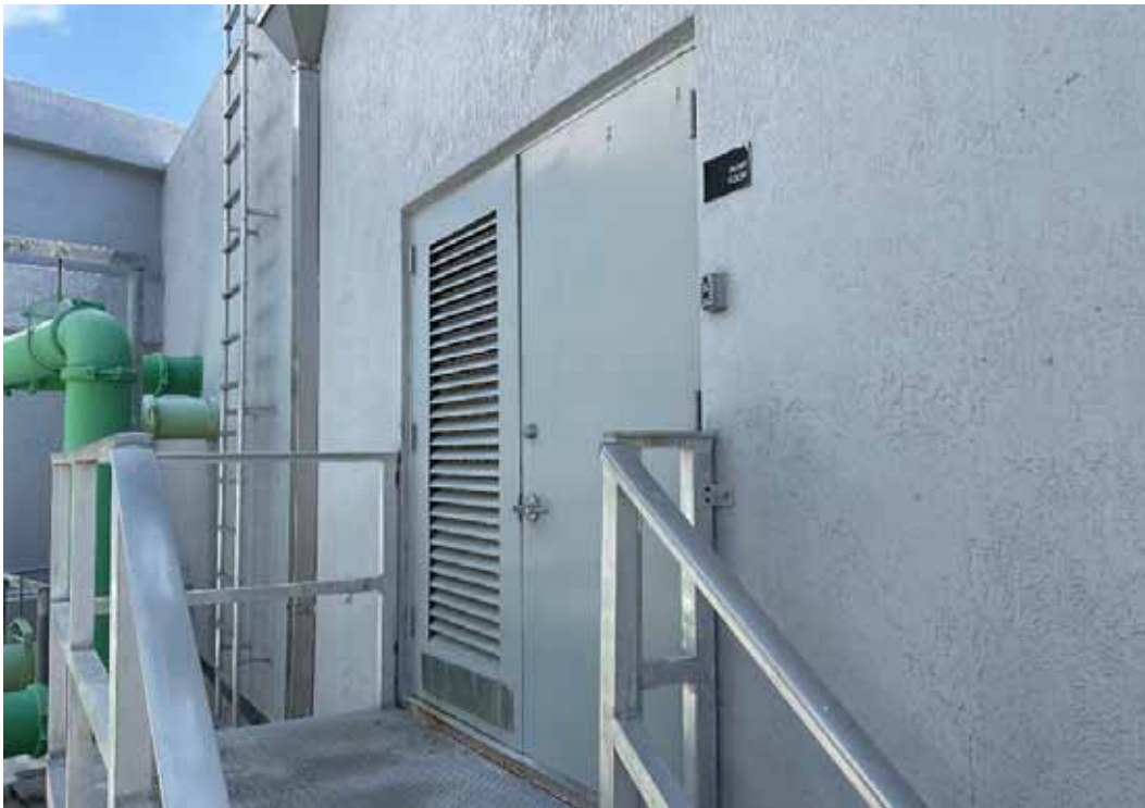
Doors - Roof Pump Room
