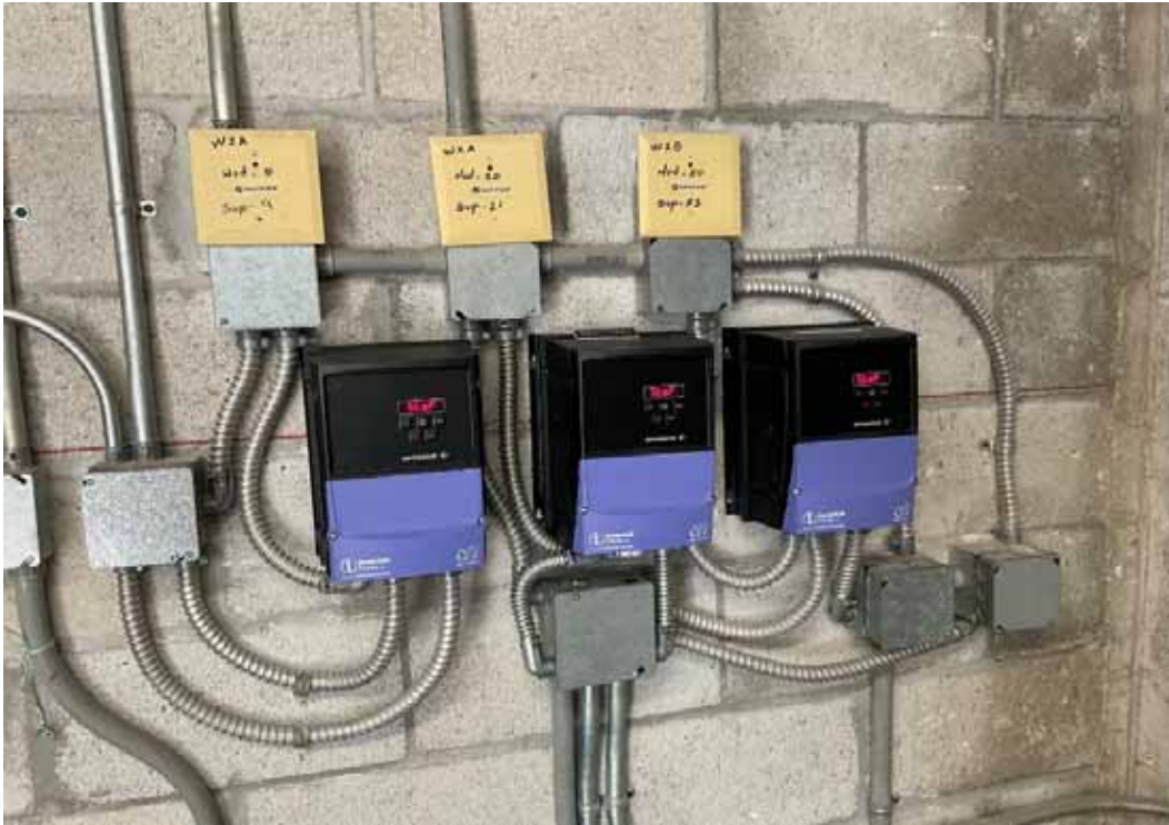
Var Freq Drives - Supply Fans
