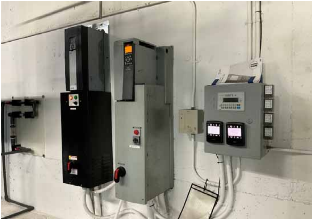
Var Freq Drives - A/C Cooling Towers
