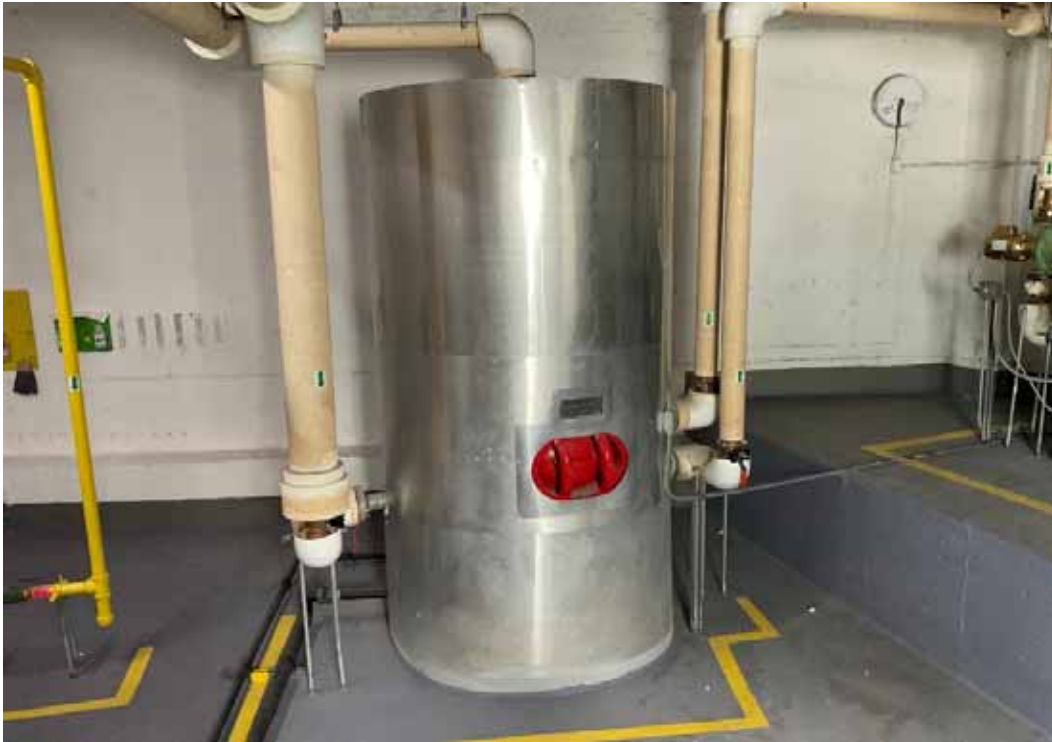
Boiler Storage Tank
