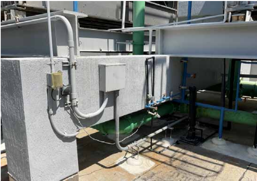
A/C Cooling Tower Supports
