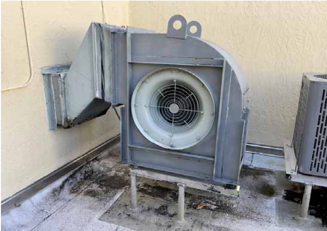
Pressurization Fan - North Tower
