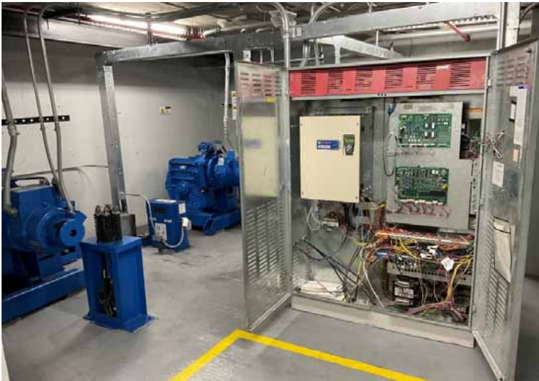
Elevator Equipment - South Tower
