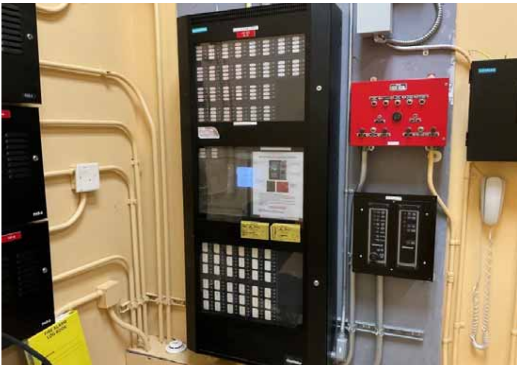
Fire Alarm Panel
