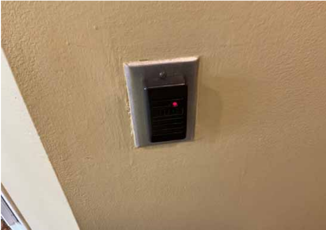
Access Control - FOB Reader
