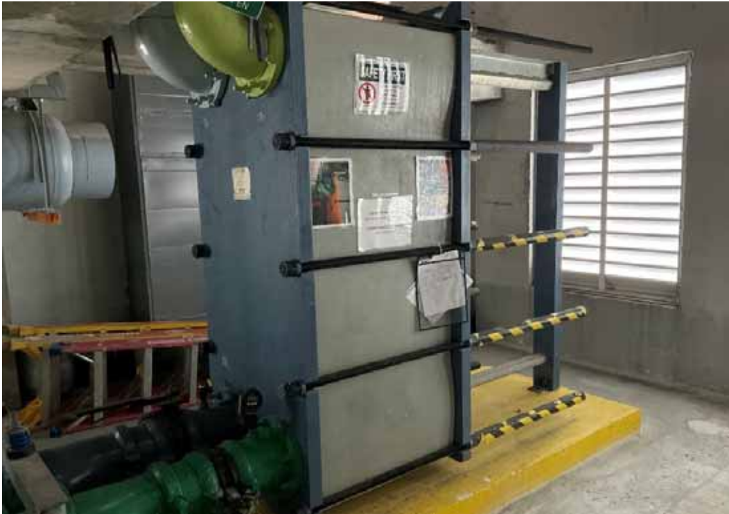
A/C Heat Exchanger
