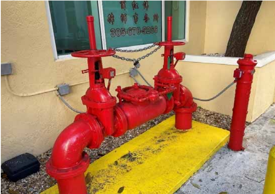
Backflow Preventer - Fire
