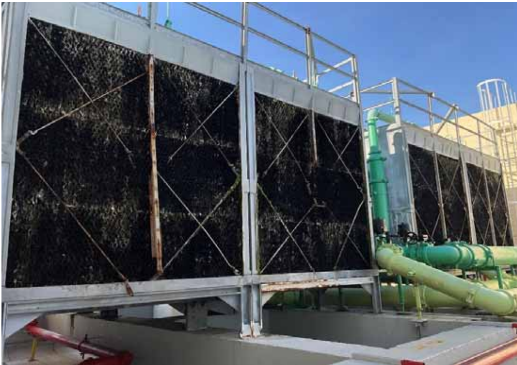
A/C Cooling Towers
