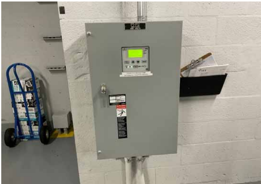
Domestic Water System Automatic Transfer Switch
