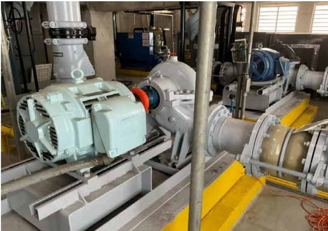
A/C Condensing Pumps - Closed Loop
