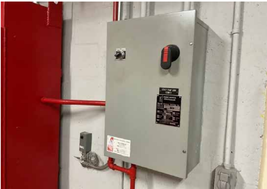
Fire Jockey Pump Controller
