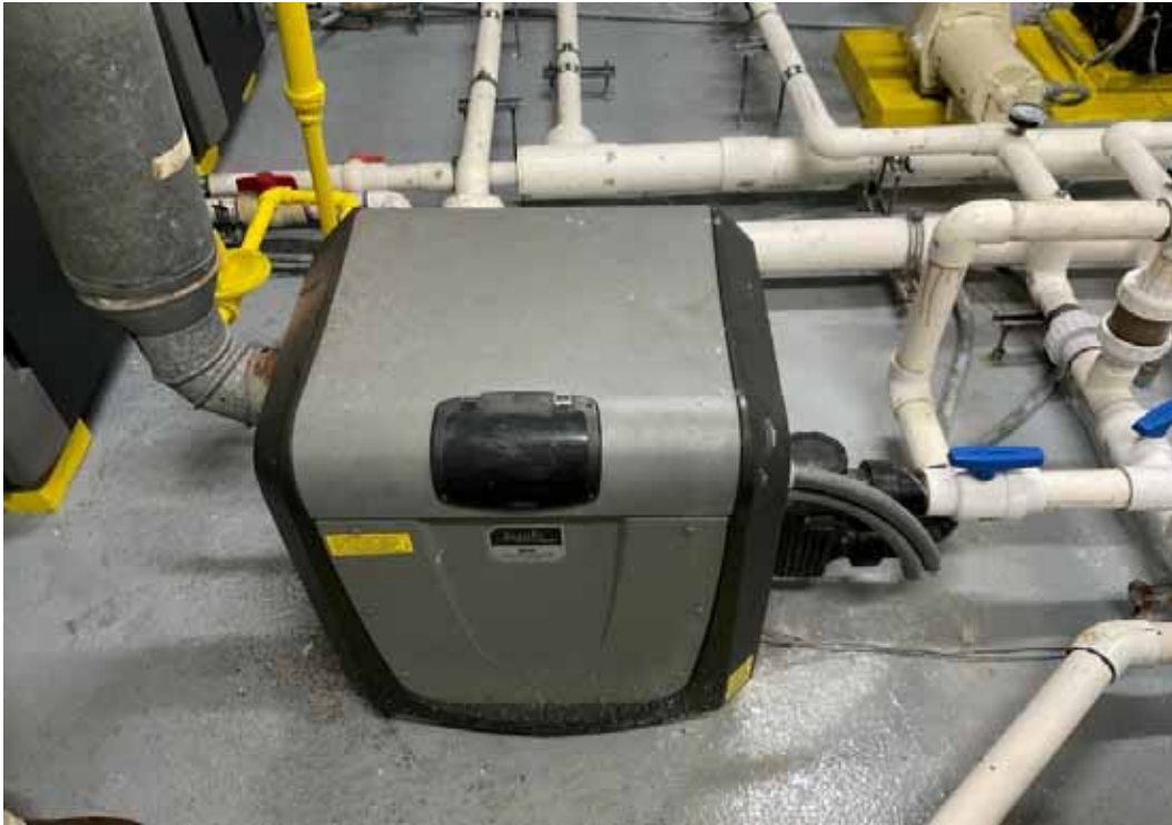
Spa Equipment, Heater
