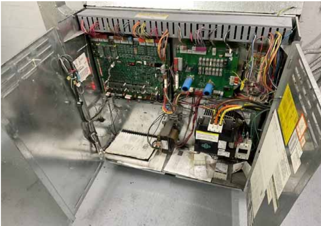
Elevator Equipment - Garage
