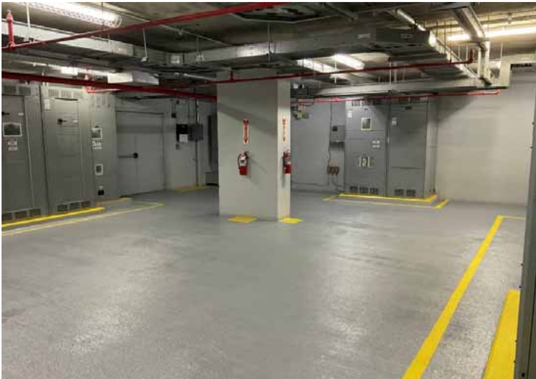
Main Electrical Room
