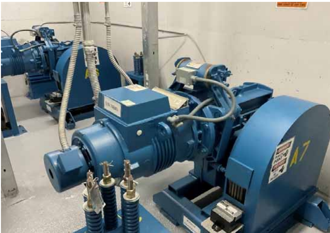
Elevator Equipment - North Tower
