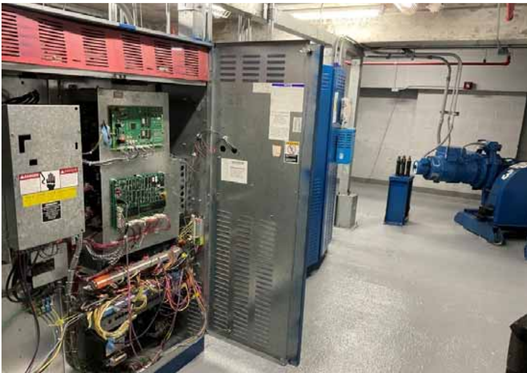
Elevator Equipment - South Tower
