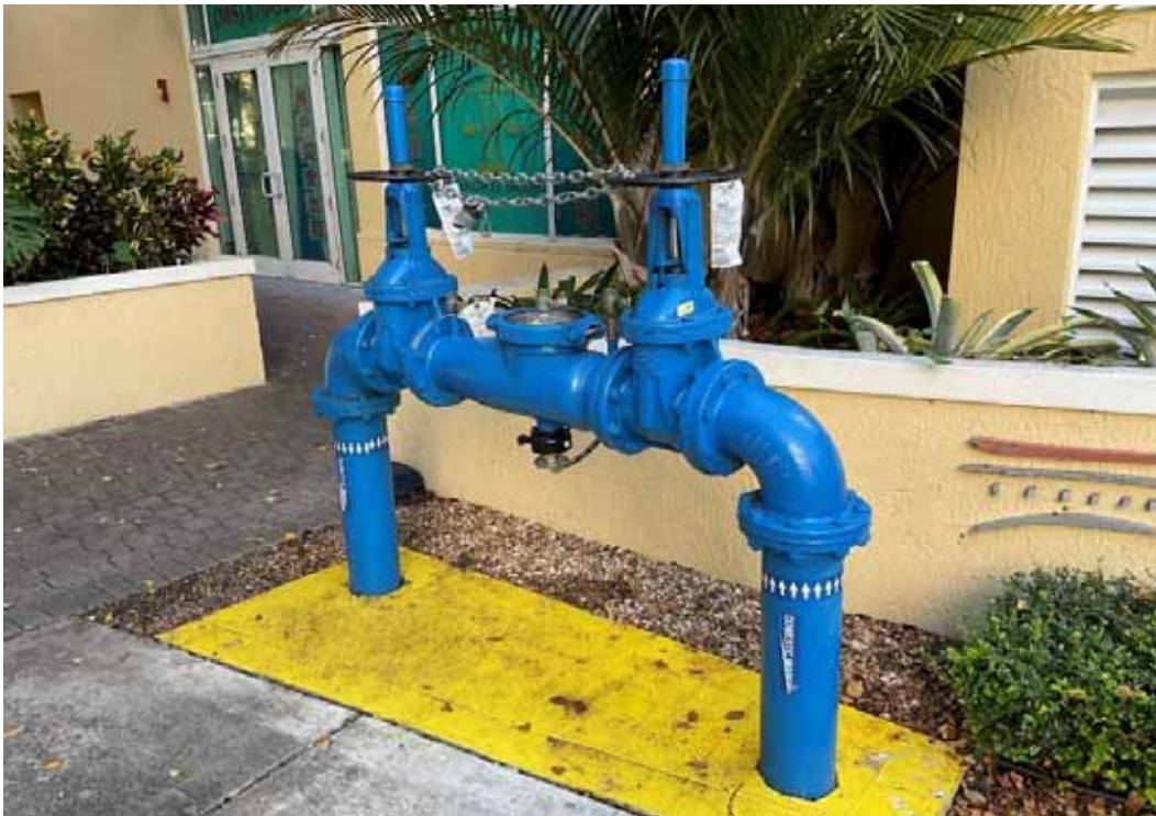
Backflow Preventer - Domestic Water
