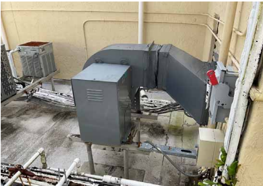
Pressurization Fan - North Tower
