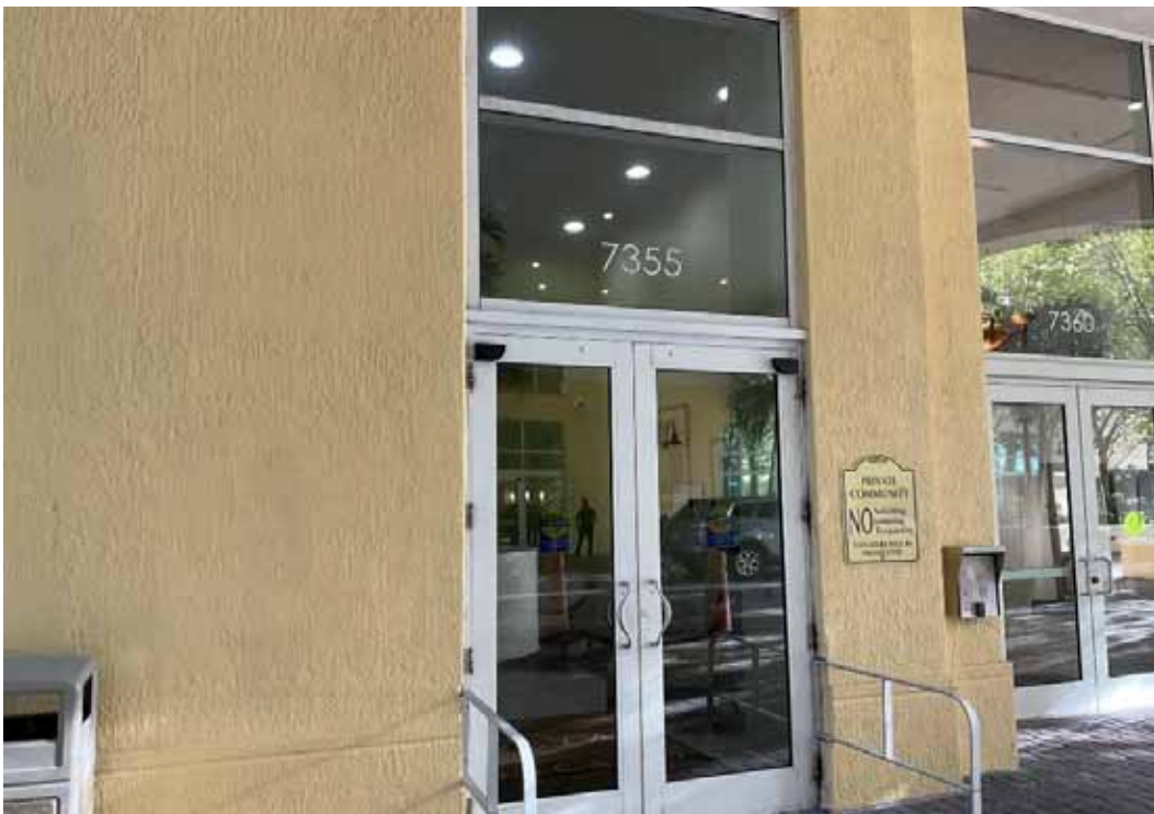
Windows & Doors - North Tower Elevator Lobby
