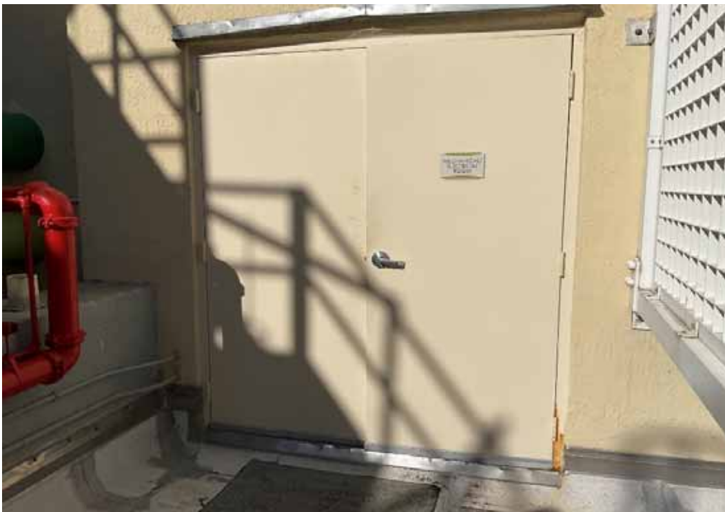
Doors - South Tower Roof Mech/Elec Room
