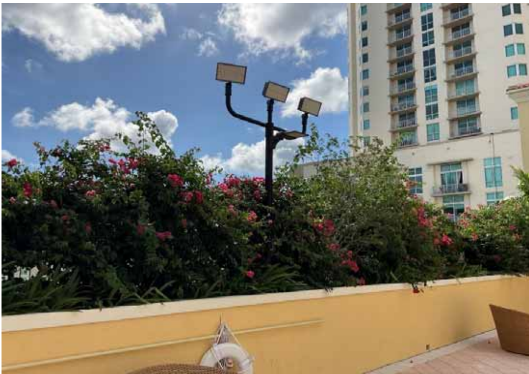
Light Pole & Fixtures - Recreation Deck
