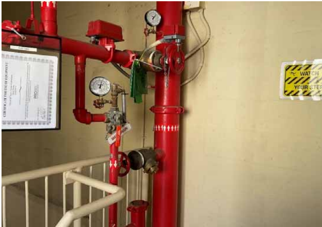
Fire Standpipe - North Tower
