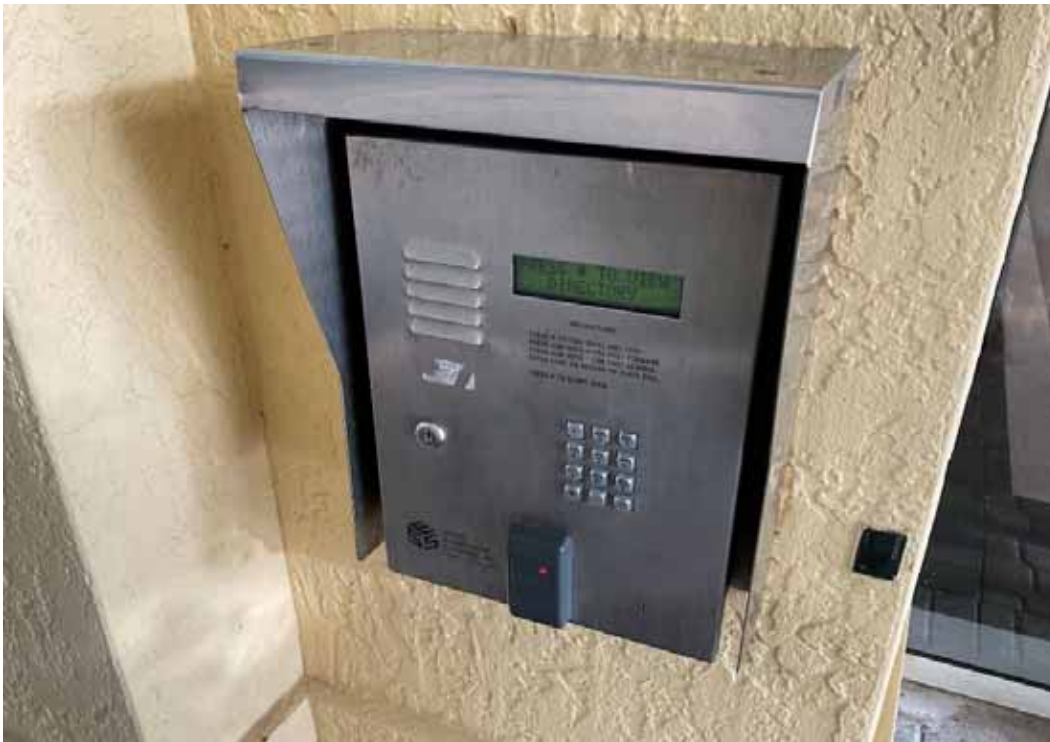
Enterphone - North Tower
