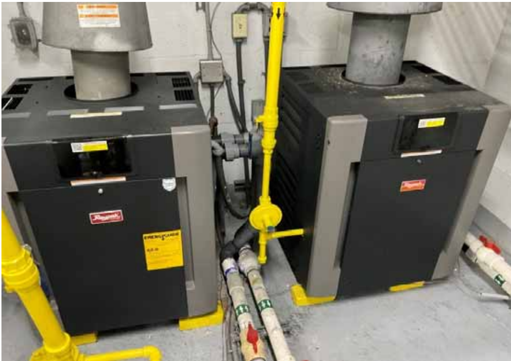
Pool Equipment, Heaters
