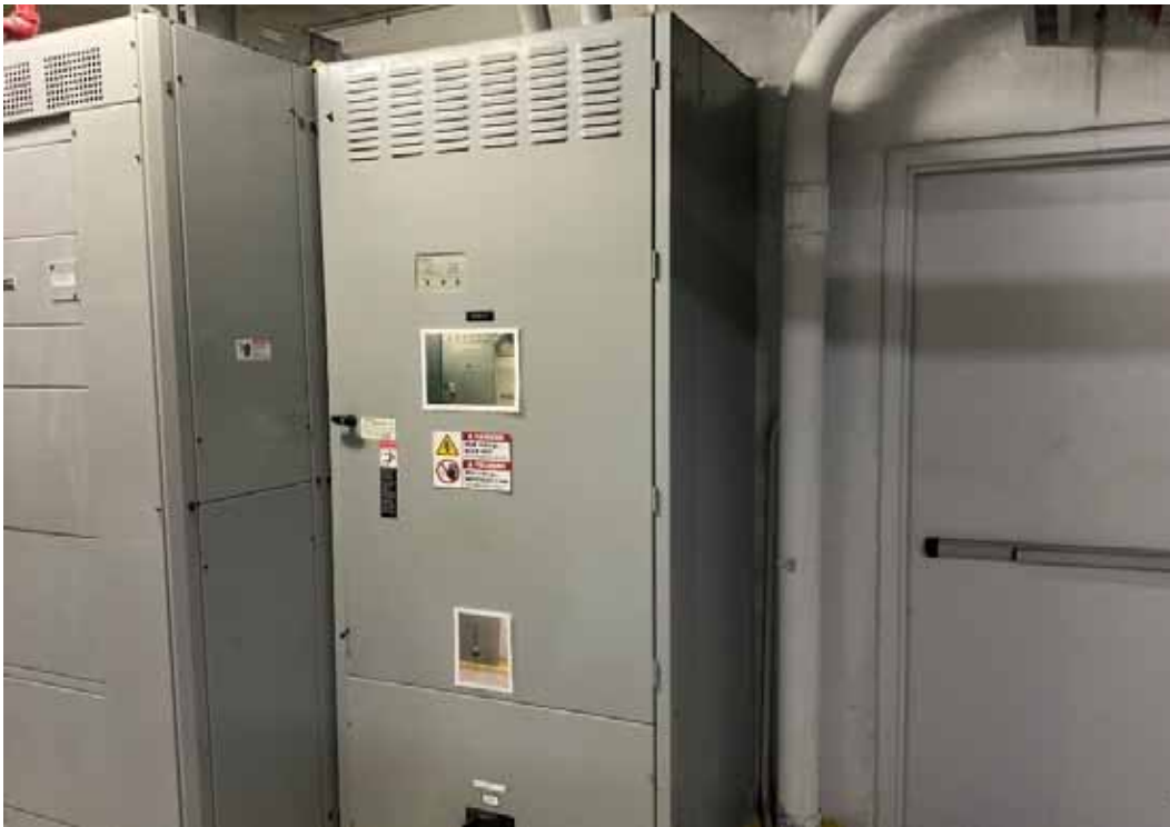
Generator Automatic Transfer Switch #1
