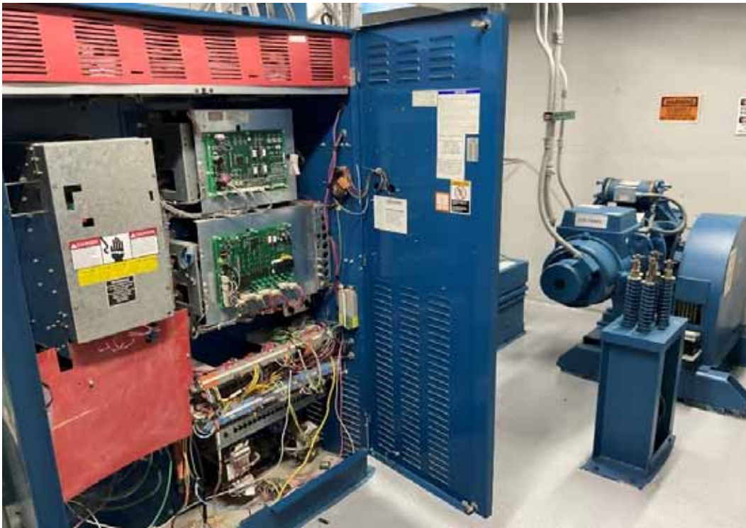
Elevator Equipment - North Tower
