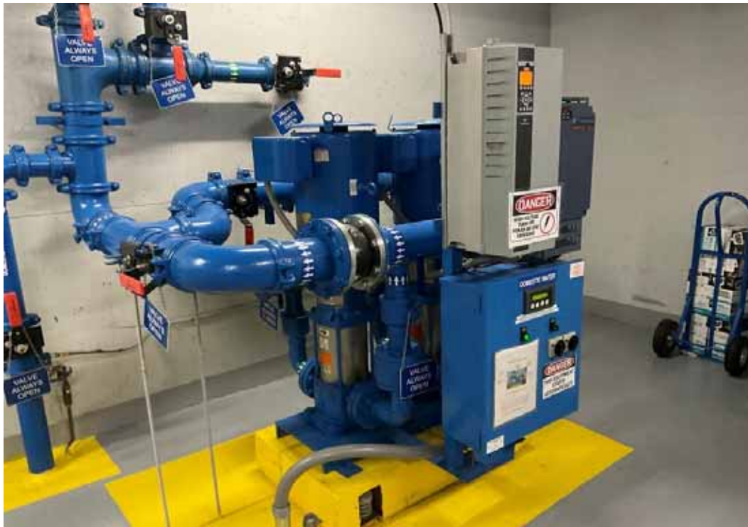
Domestic Water Booster Pump System
