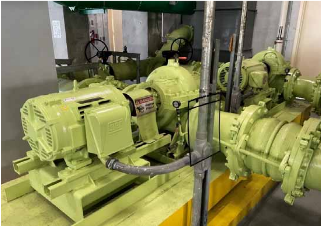
A/C Condensing Pumps - Open Loop
