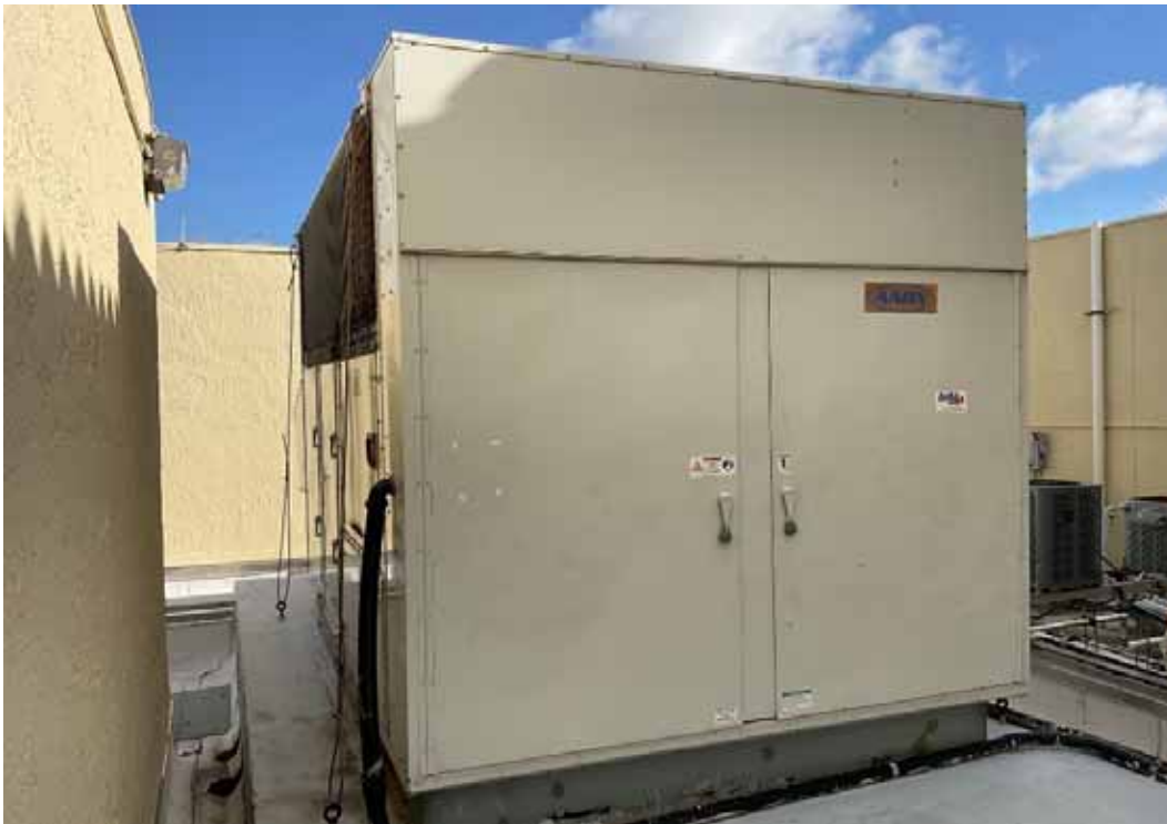
A/C RTU - North Tower Hallways
