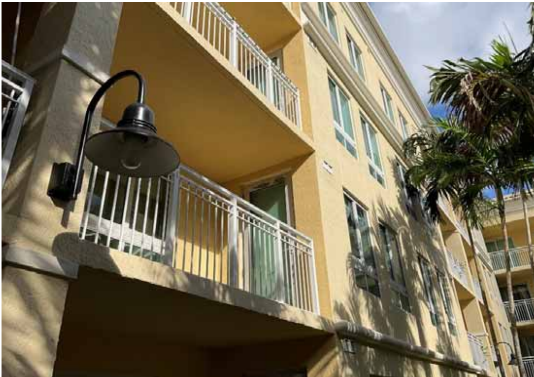
Balcony Railings - North Tower
