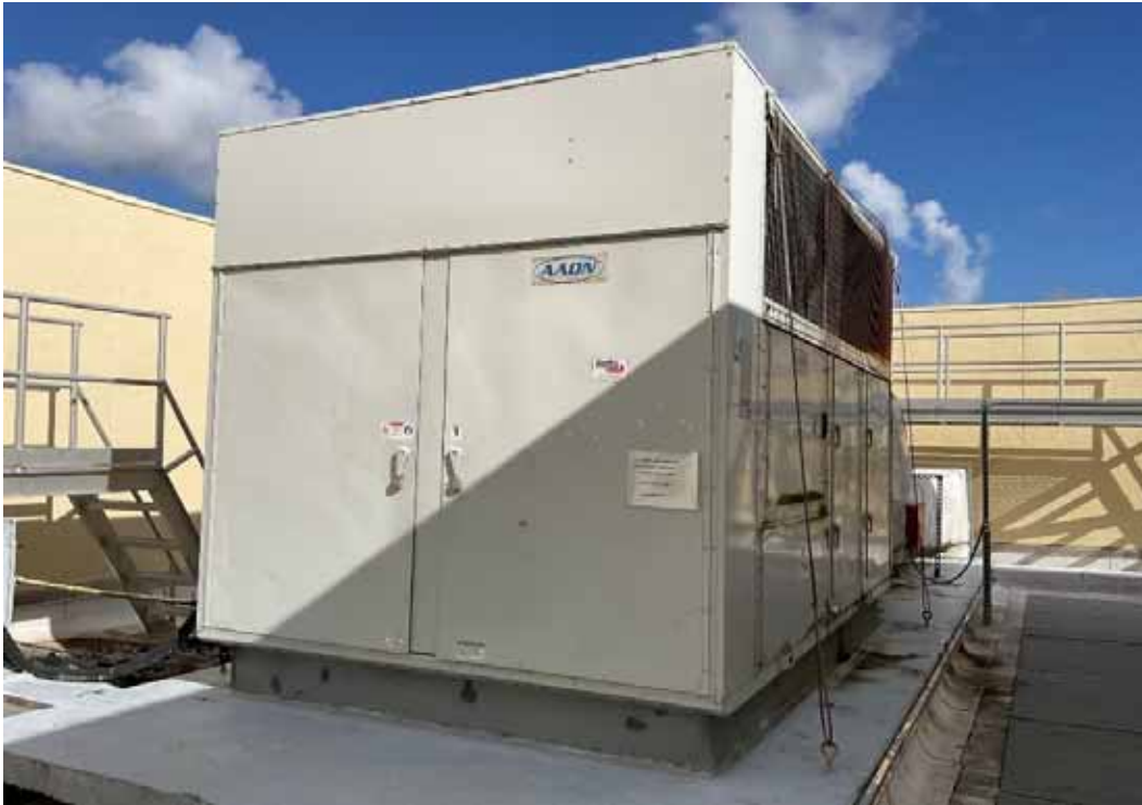
A/C RTU - North Tower Hallways
