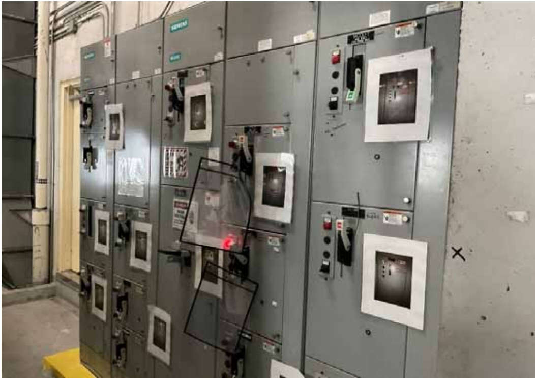
Electrical Panels - South Tower Roof Mech Room
