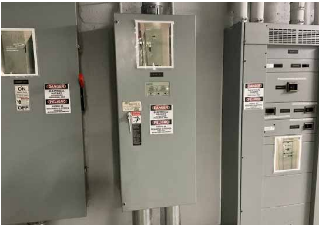
Generator Automatic Transfer Switch #3
