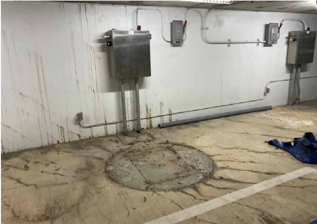
Lift Station - Sanitary Sewer
