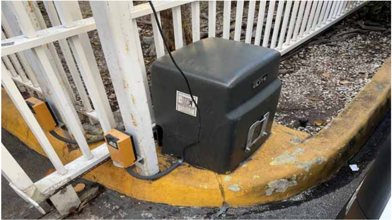
Gate Operator - Contractor Parking
