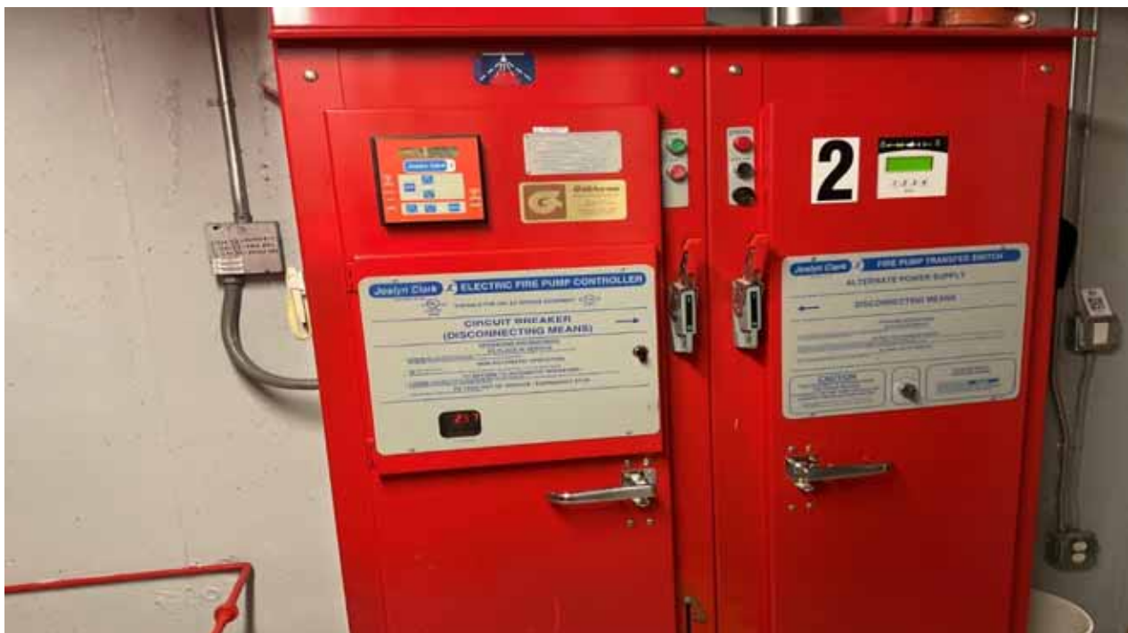
Fire Pump Controller - High Zone
