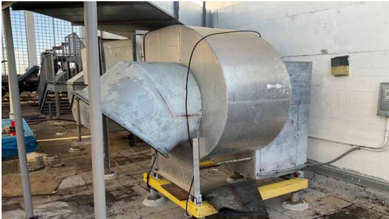
Stairwell Pressurization Fan - West
