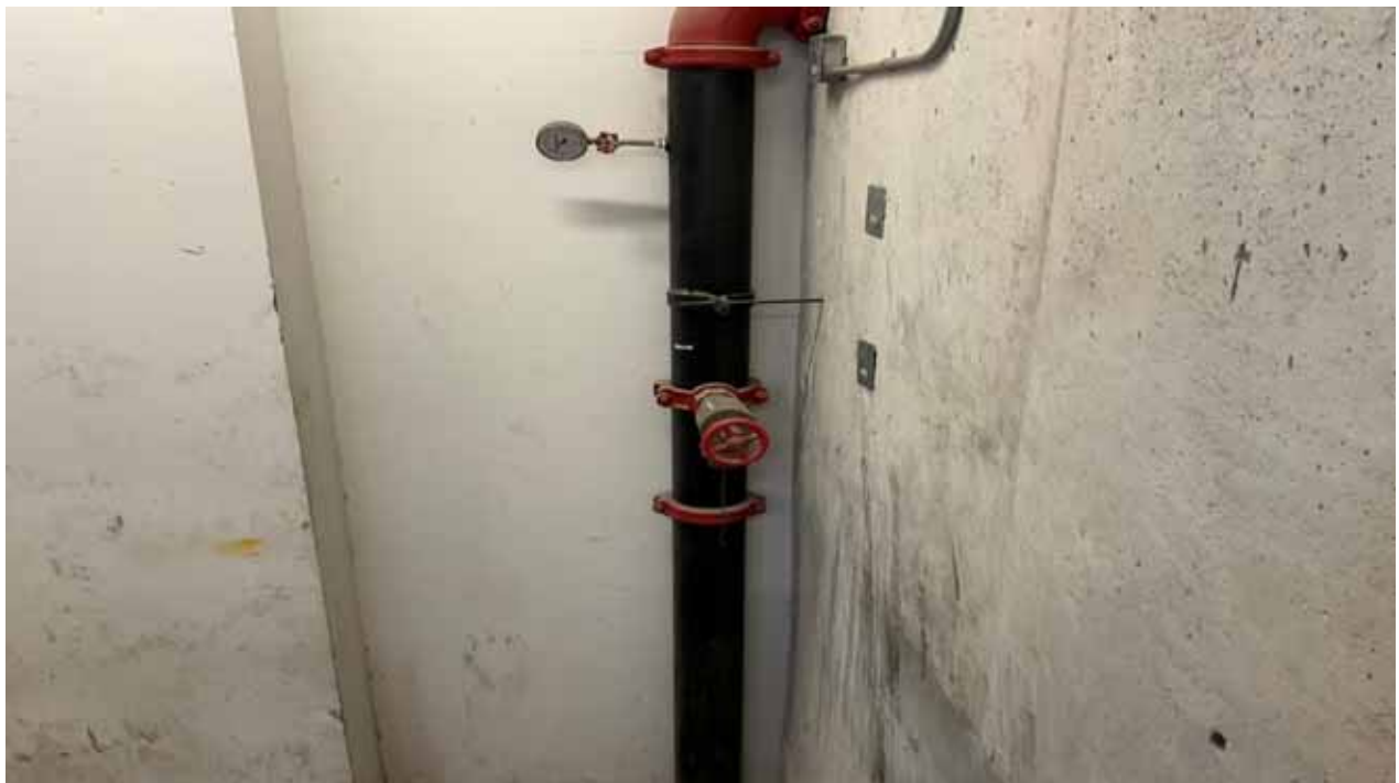
Fire Standpipe - West
