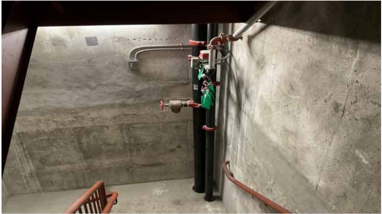
Fire Standpipe - East
