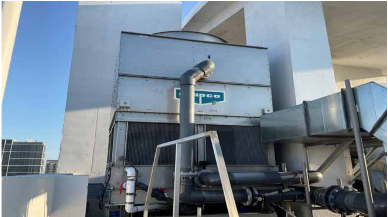
A/C Cooling Tower #4
