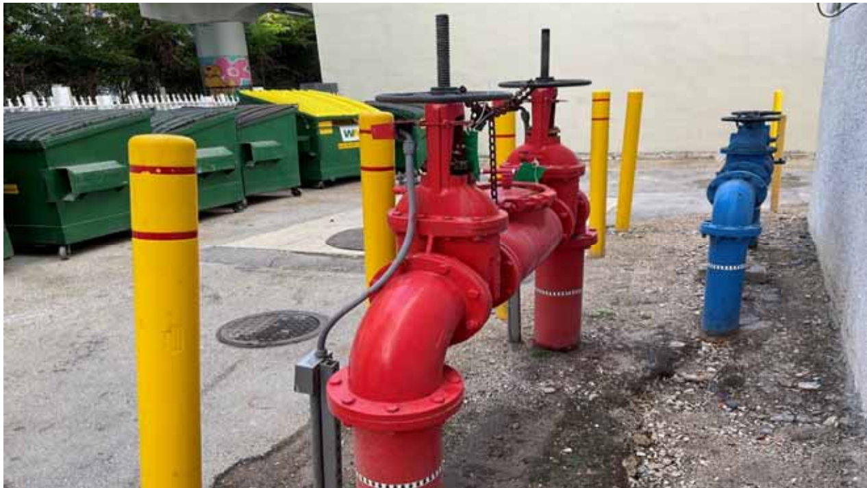
Backflow Preventer - Fire
