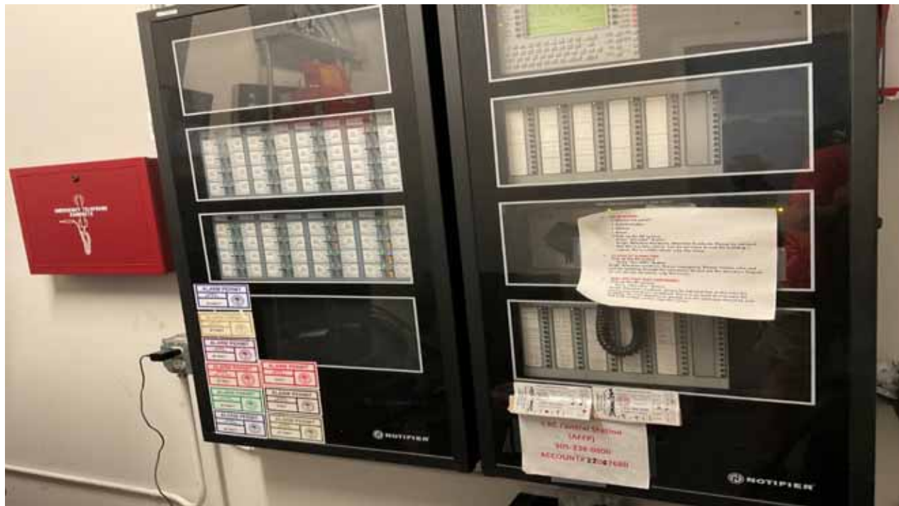
Fire Alarm Panel
