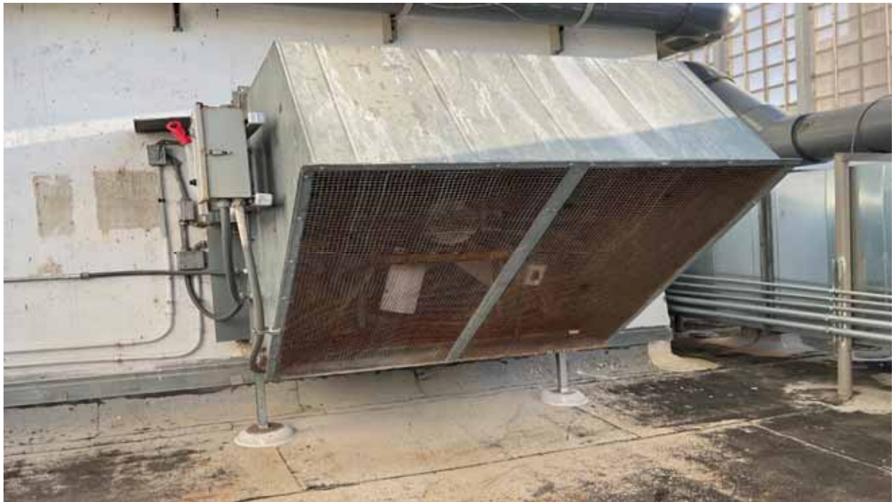
Elevator Pressurization Fan - West
