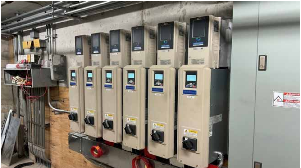
A/C Cooling Towers - Var Freq Drives
