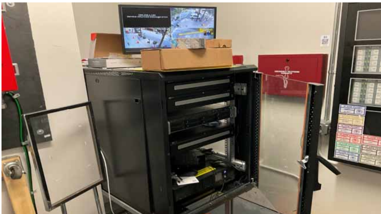
Video Surveillance System Equipment
