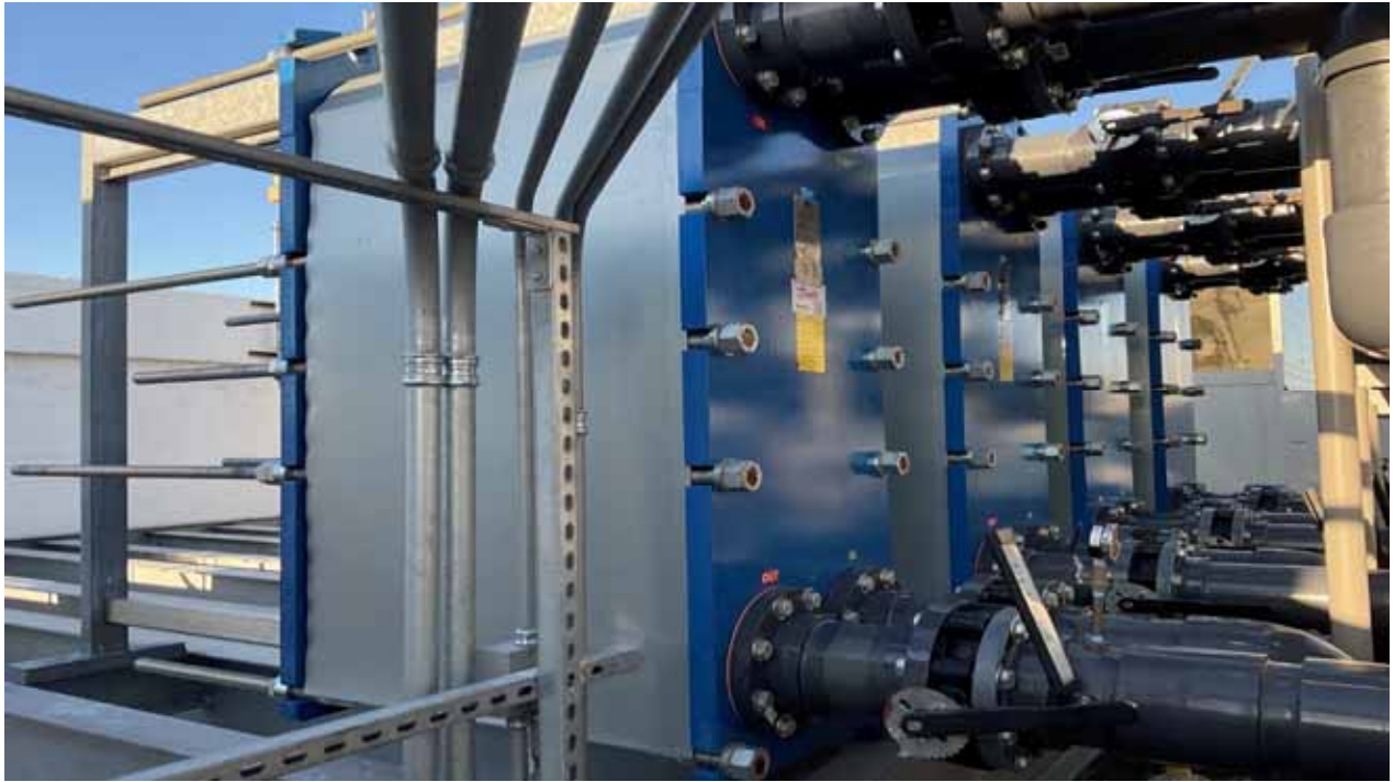
A/C Heat Exchangers
