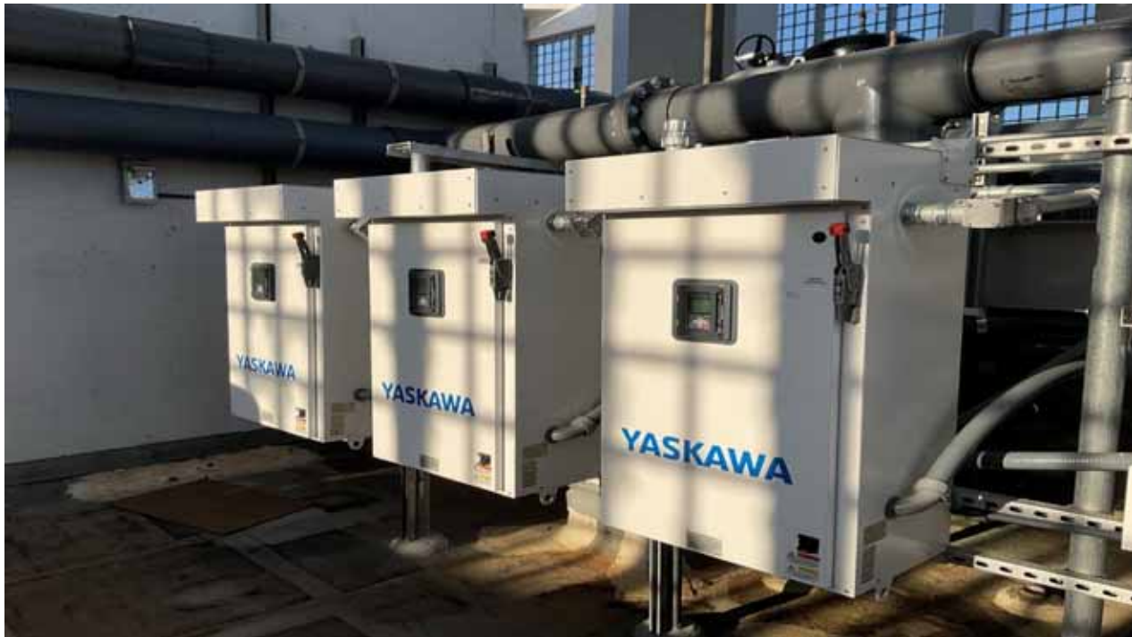
A/C Condensing Pump VFD's - Closed Loop
