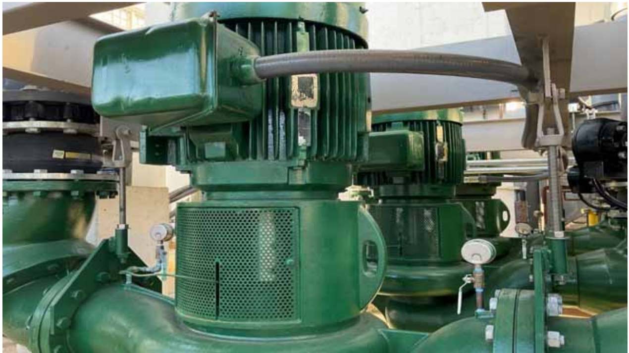
A/C Condensing Pumps - Closed Loop
