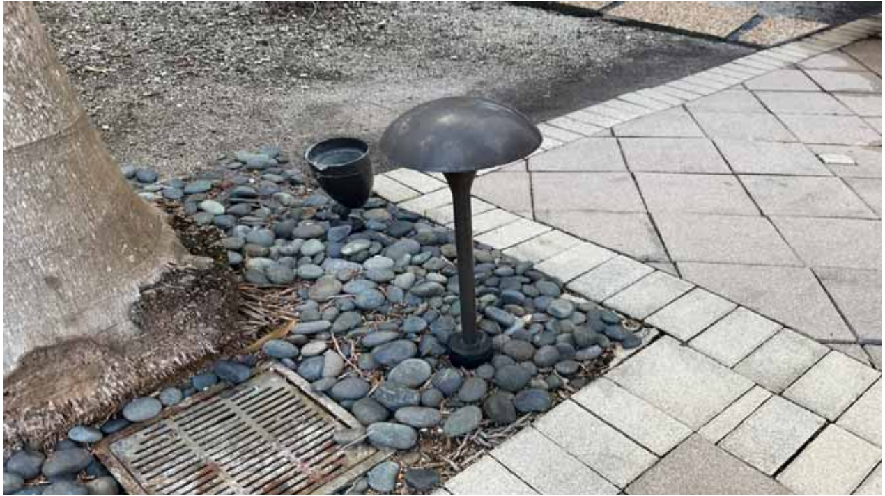
Light Fixture - Ground Level Pool Deck
