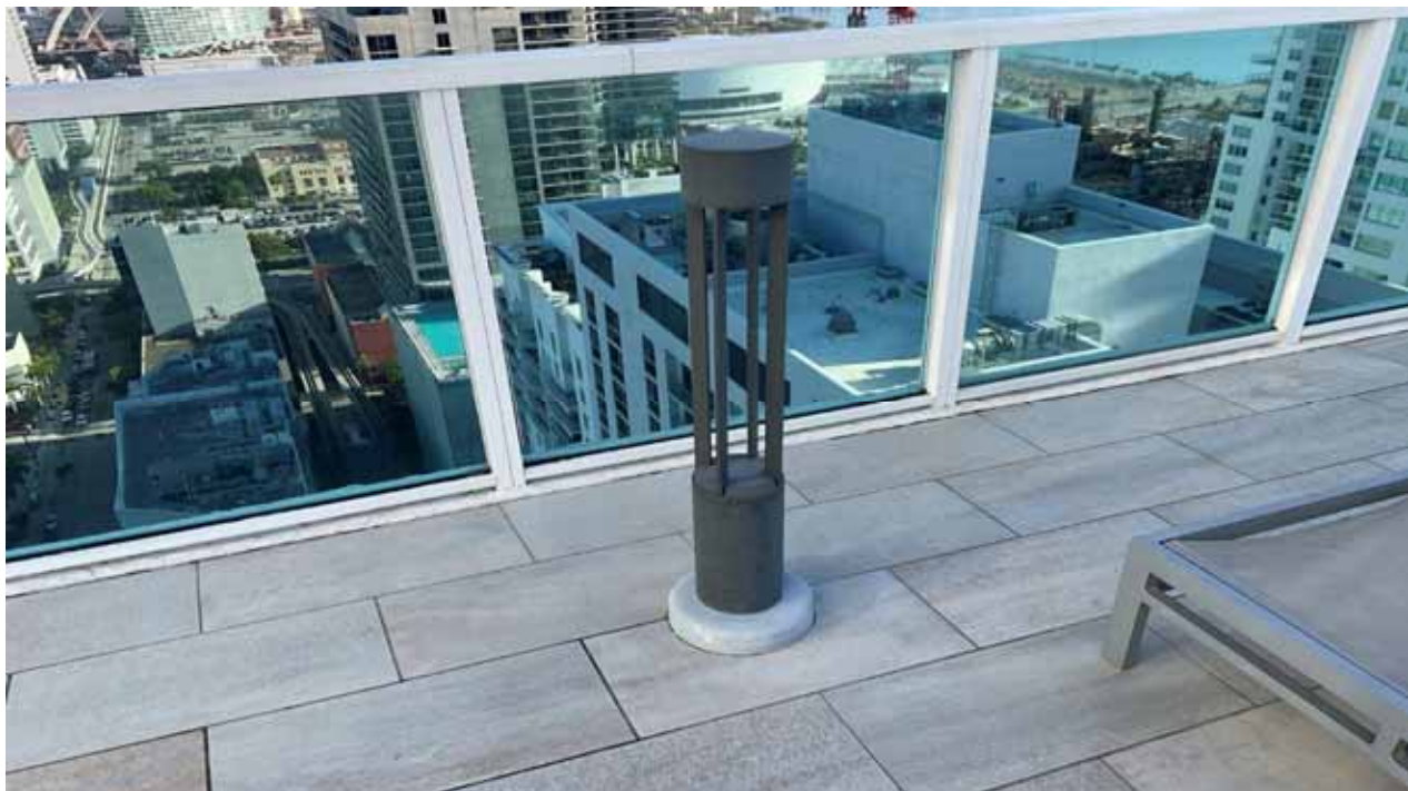
Light Bollard - Pool Deck
