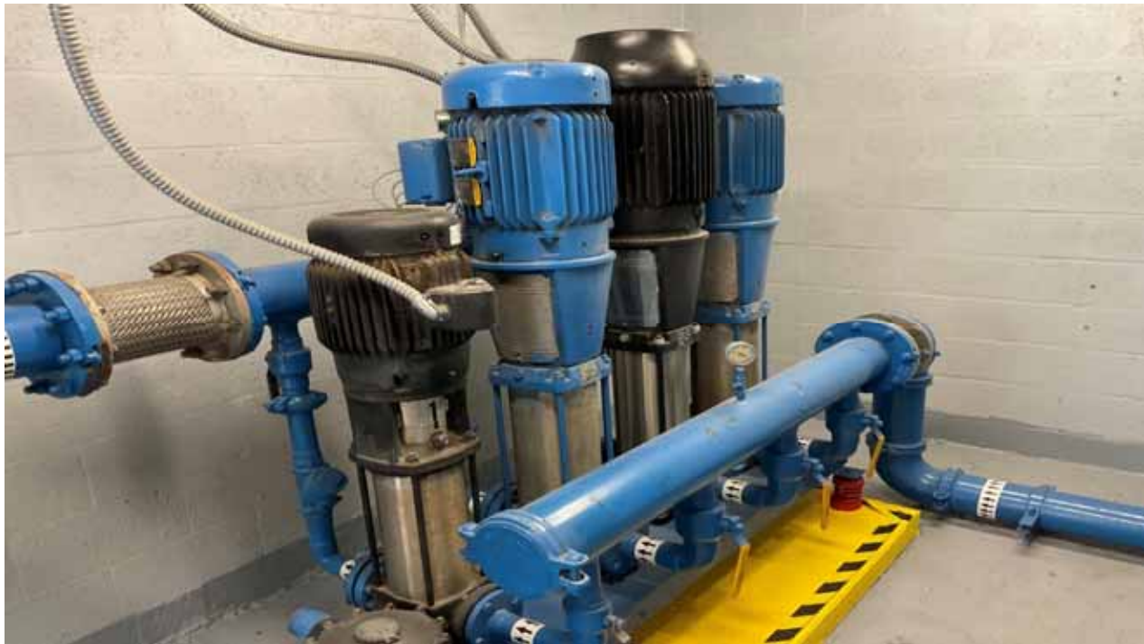
Domestic Water Booster Pumps
