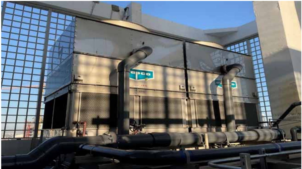
A/C Cooling Towers #2 & 5
