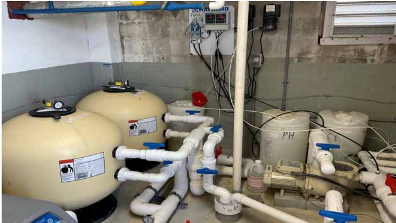
Rooftop Pool Equipment
