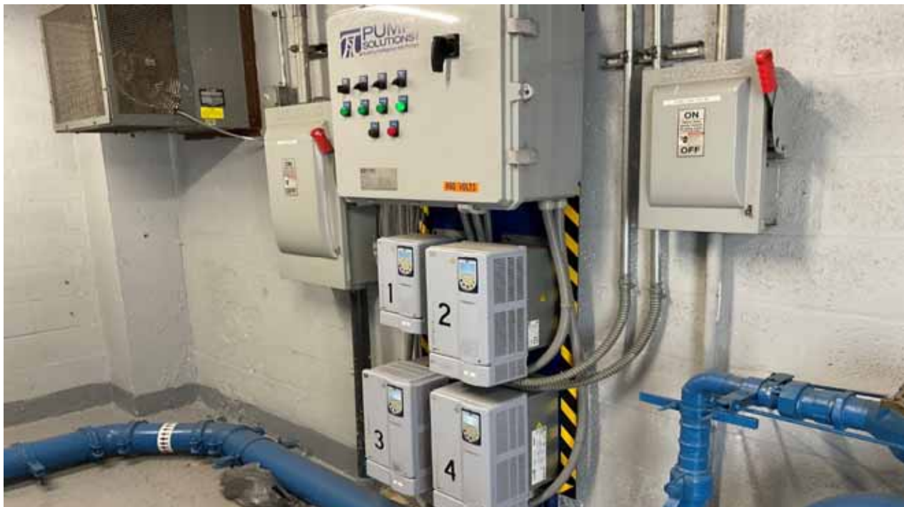
Domestic Water Control Panel & VFD's
