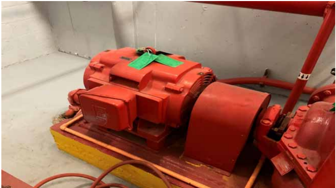
Fire Pump - Low Zone
