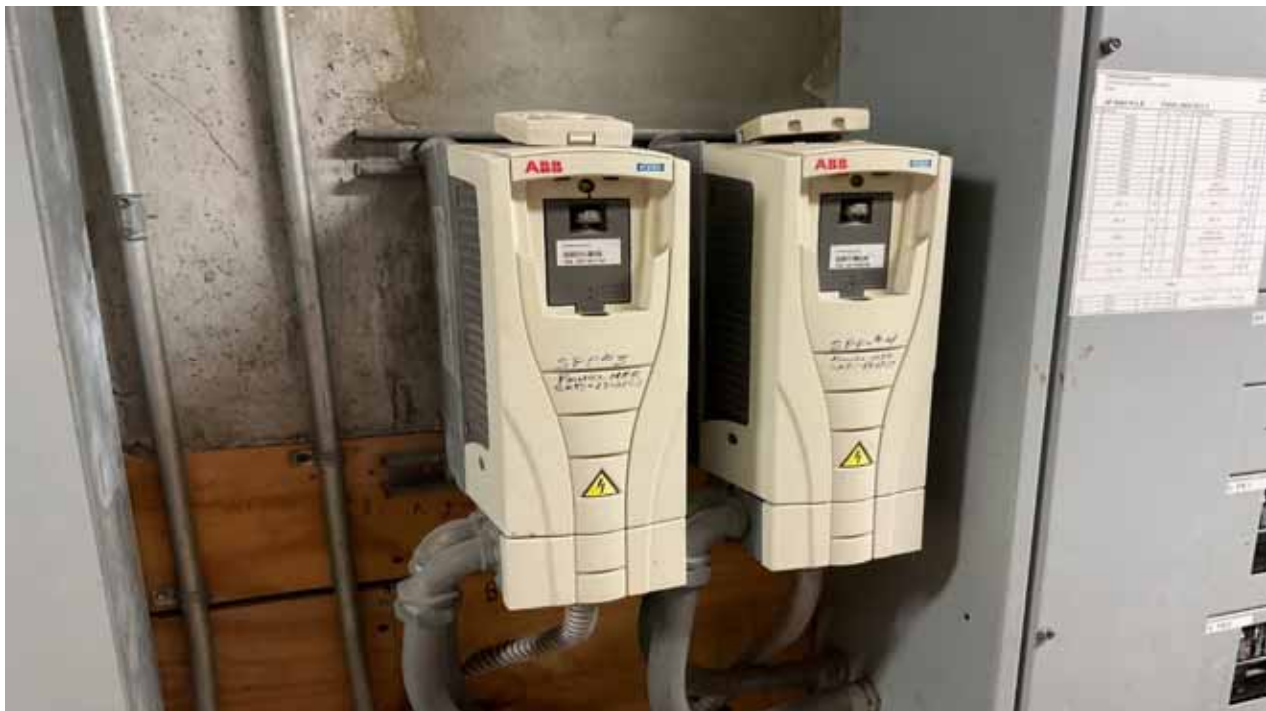
Stairwell Pressurization Fans - Var Freq Drives
