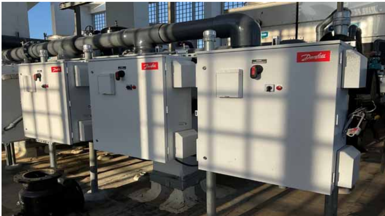
A/C Condensing Pump VFD's - Open Loop
