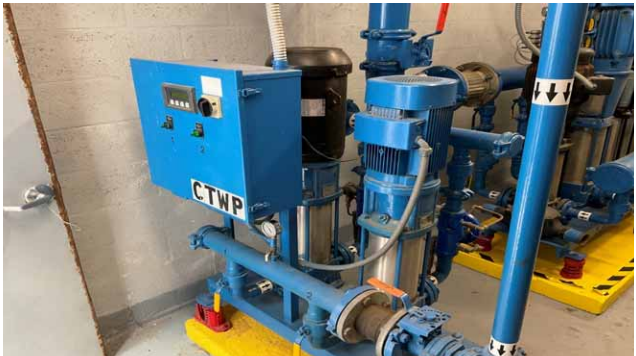
A/C Cooling Tower Drain Pump System
