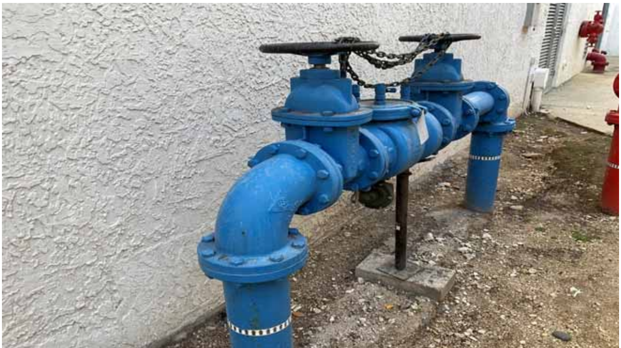
Backflow Preventer - Domestic Water
