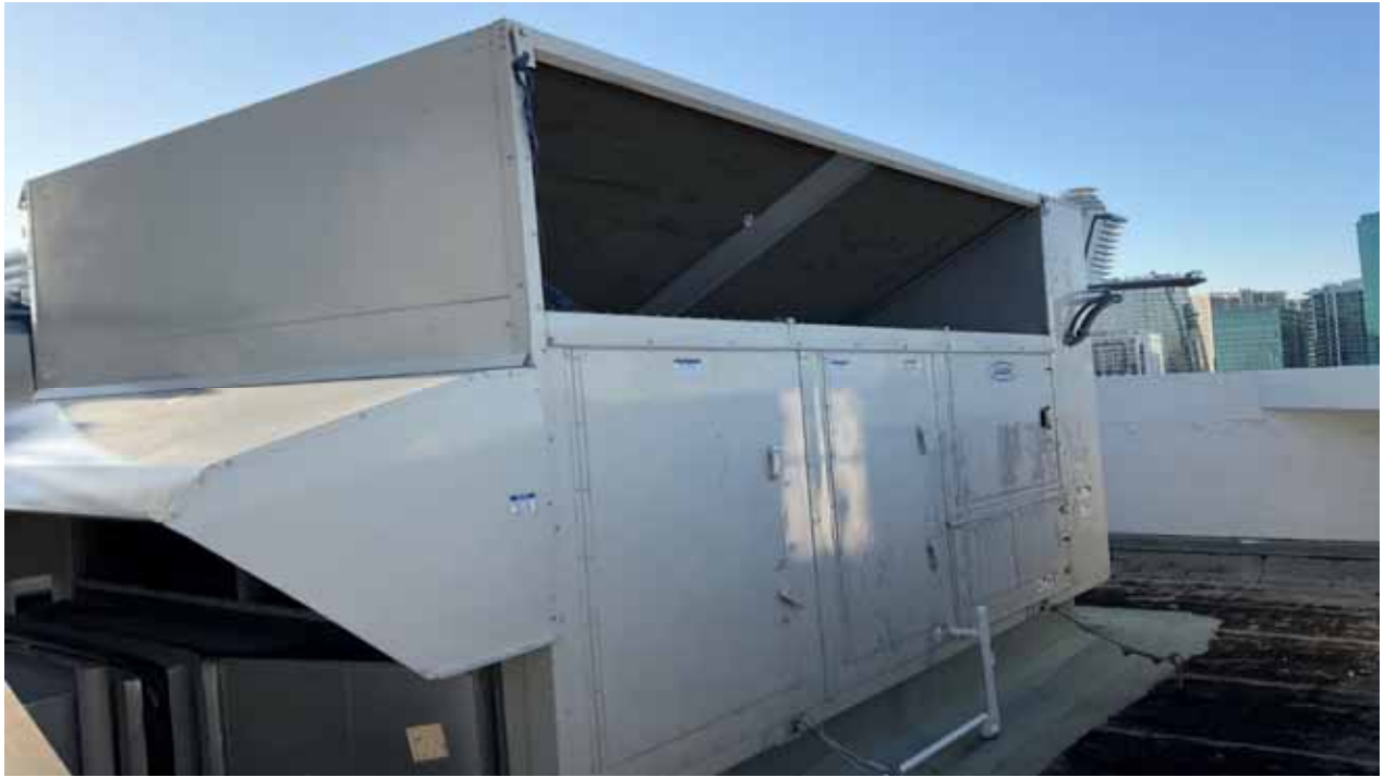
A/C Outside Air Unit #1 - Hallways West
