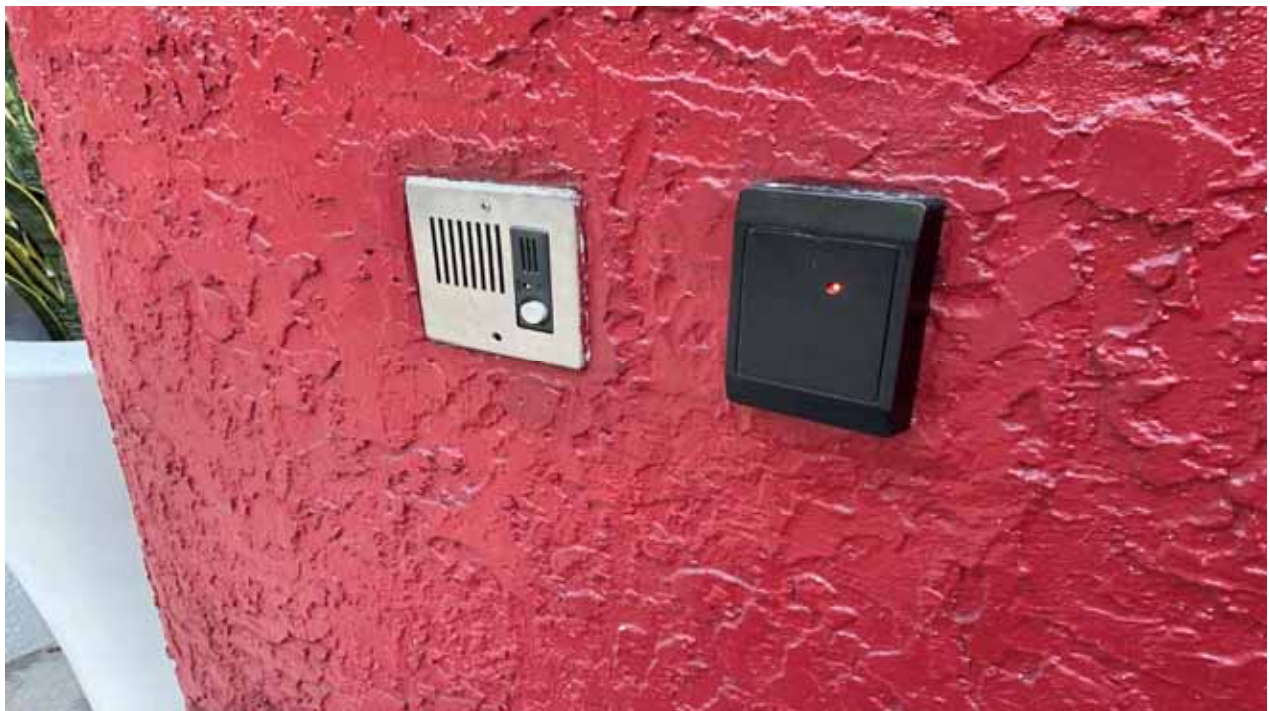
Access Control - FOB Reader & Intercom
