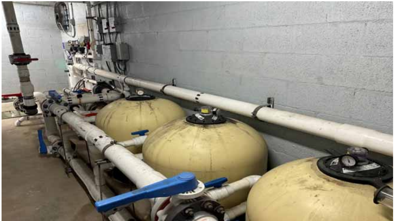
Ground Level Pool Equipment
