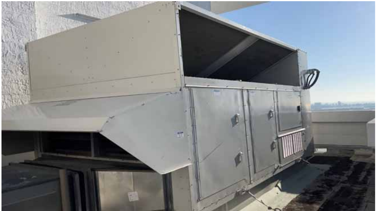
A/C Outside Air Unit #3 - Hallways East
