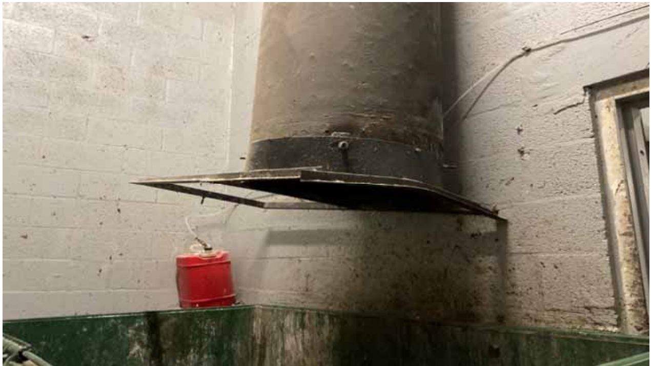
Trash Chute Guillotine - East
