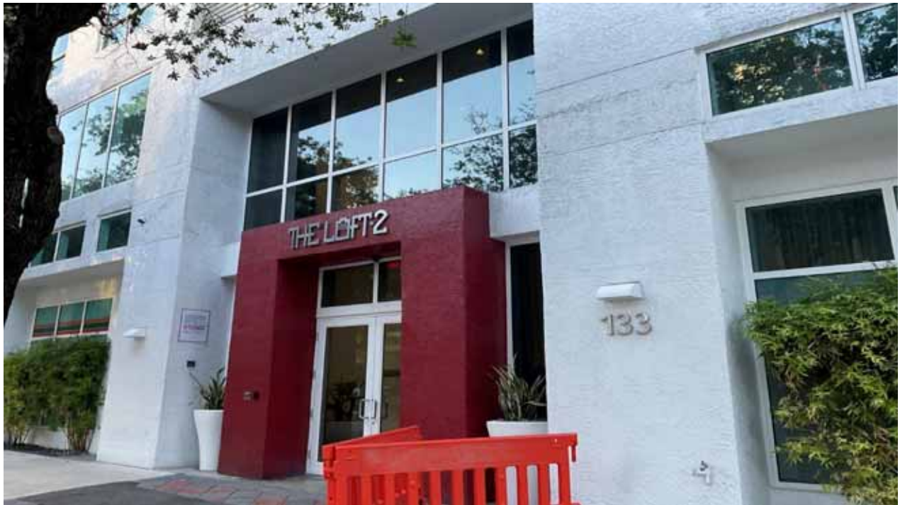
Windows & Doors - Main Lobby West
