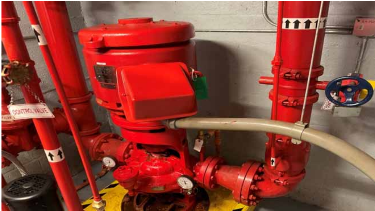
Fire Pump - High Zone
