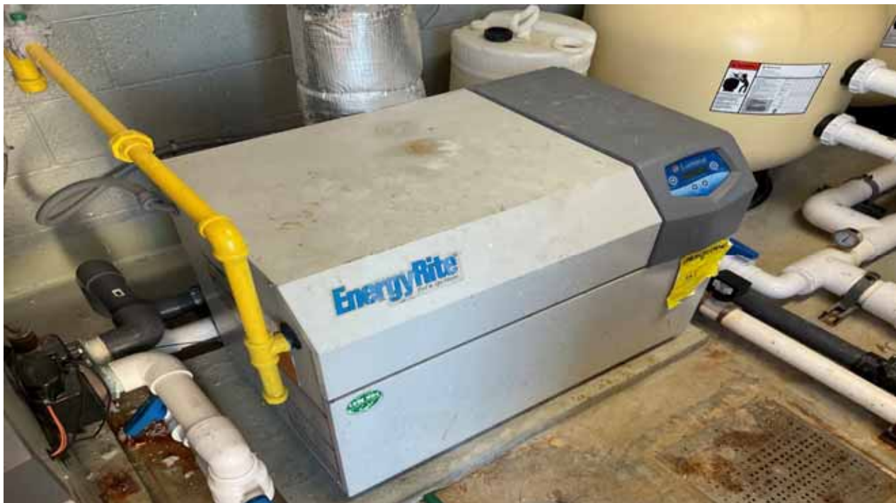
Rooftop Pool Equipment, Heater
