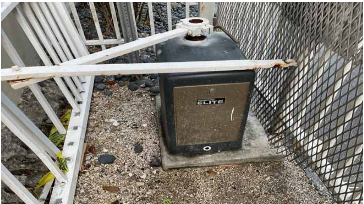
Gate Operator - Receiving Area
