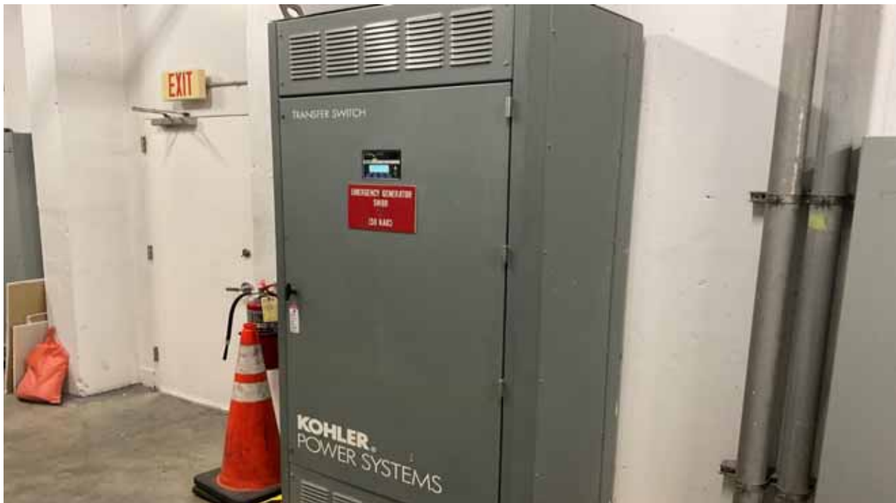
Generator Transfer Switch
