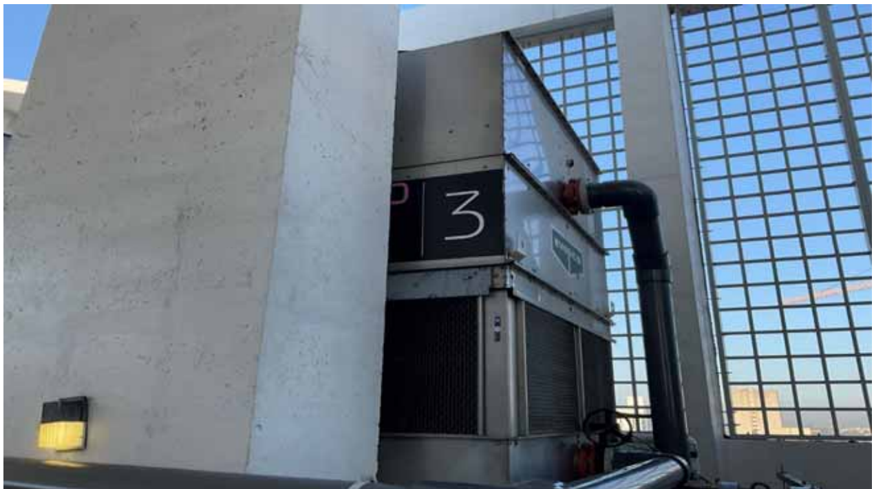
A/C Cooling Tower #1
