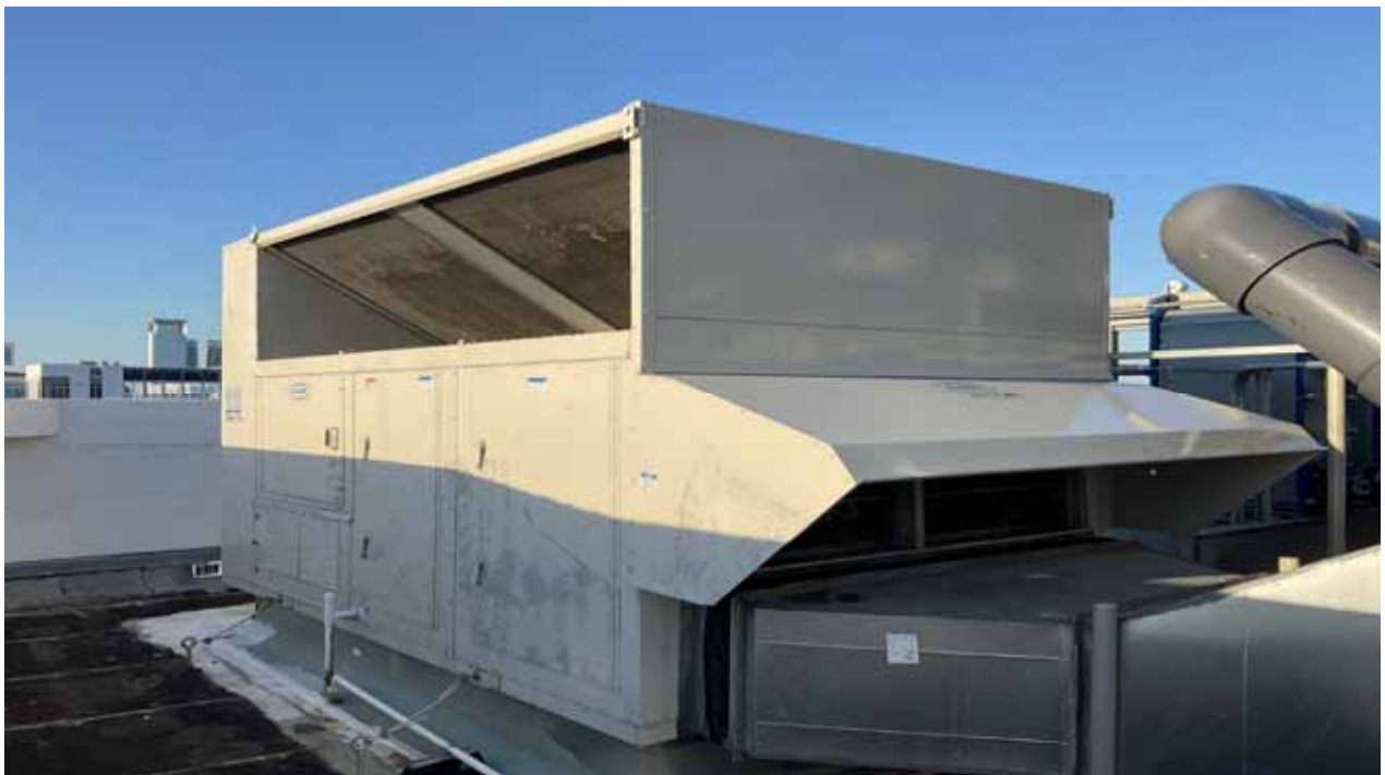
A/C Outside Air Unit #2 - Hallways West
