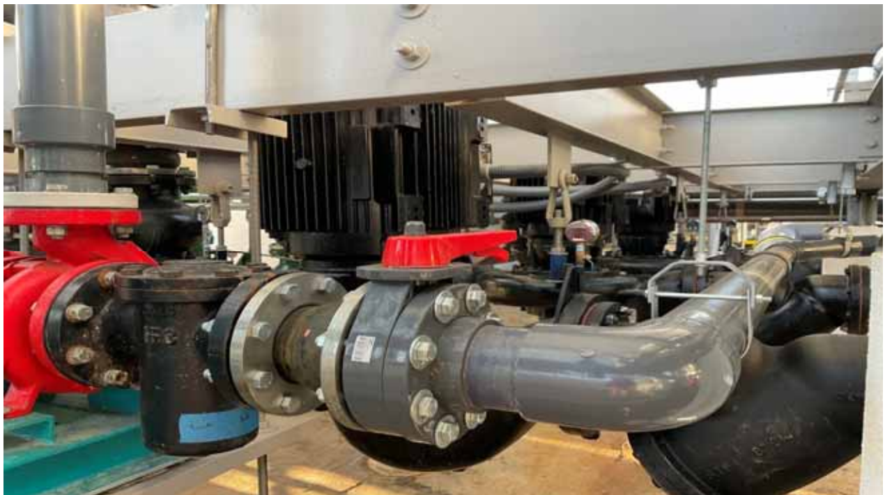
A/C Condensing Pumps - Open Loop
