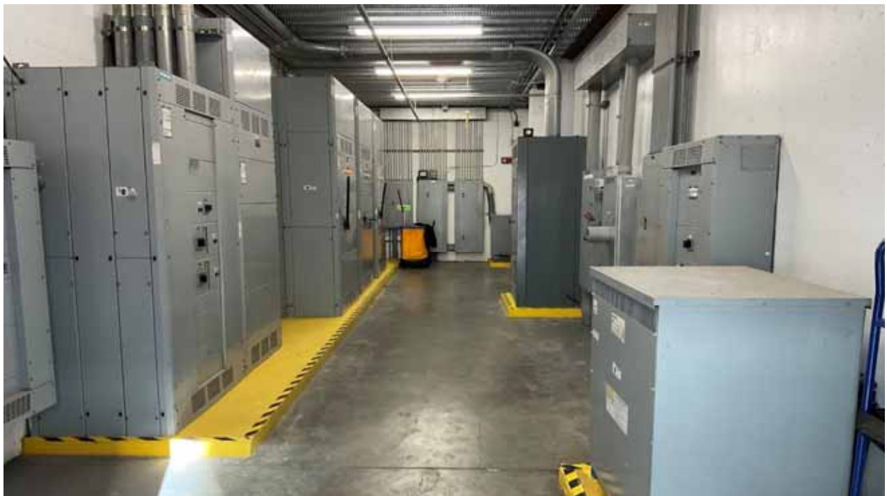
Main Electrical Room
