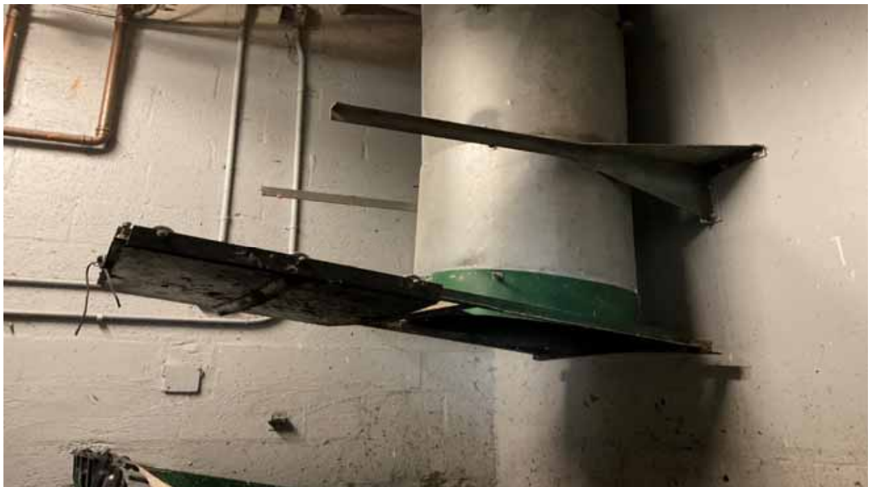
Trash Chute Guillotine - West
