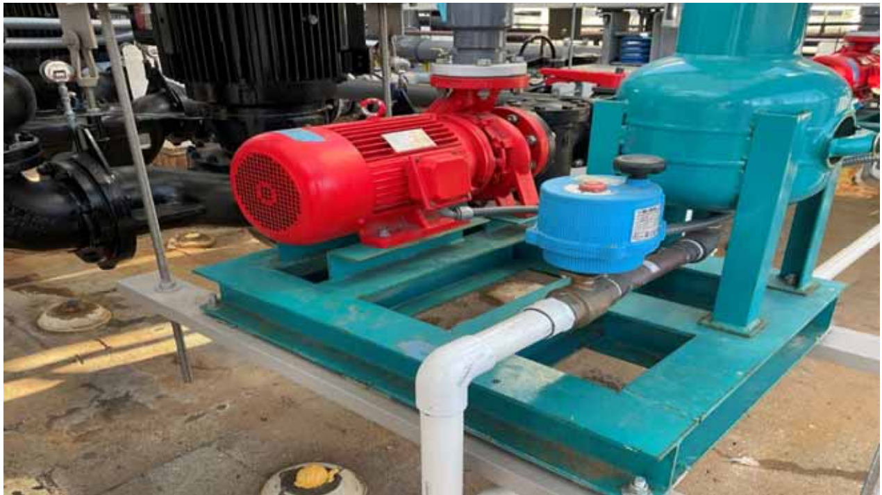
A/C Cooling Tower Filtration System (1 of 2)
