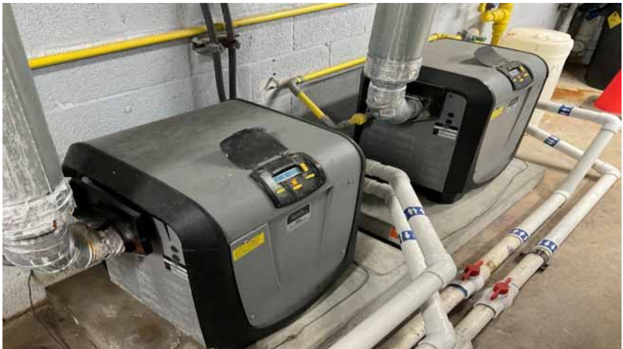
Ground Level Pool Equipment, Heaters
