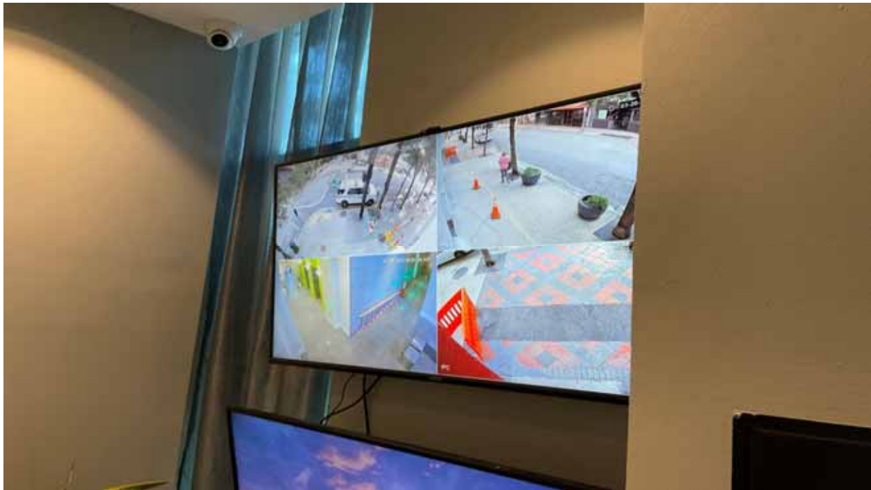
Video Surveillance System Equipment
