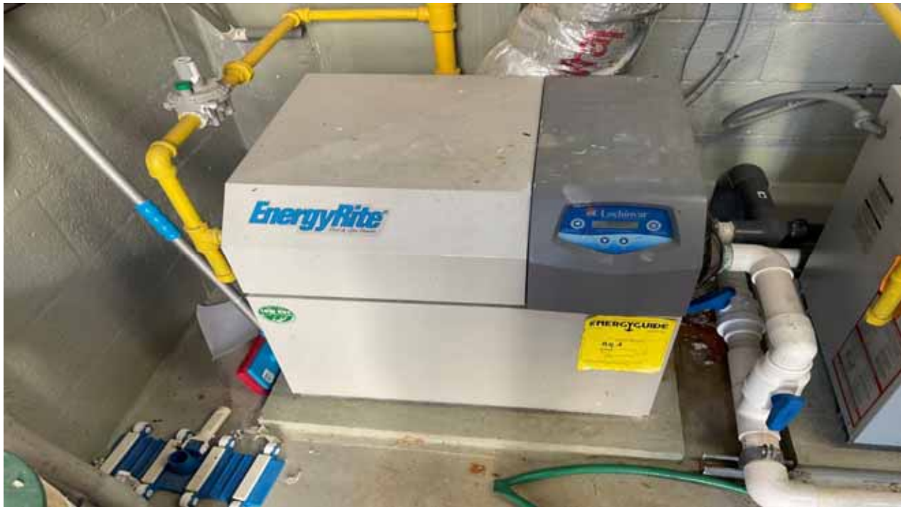
Spa Equipment, Heater
