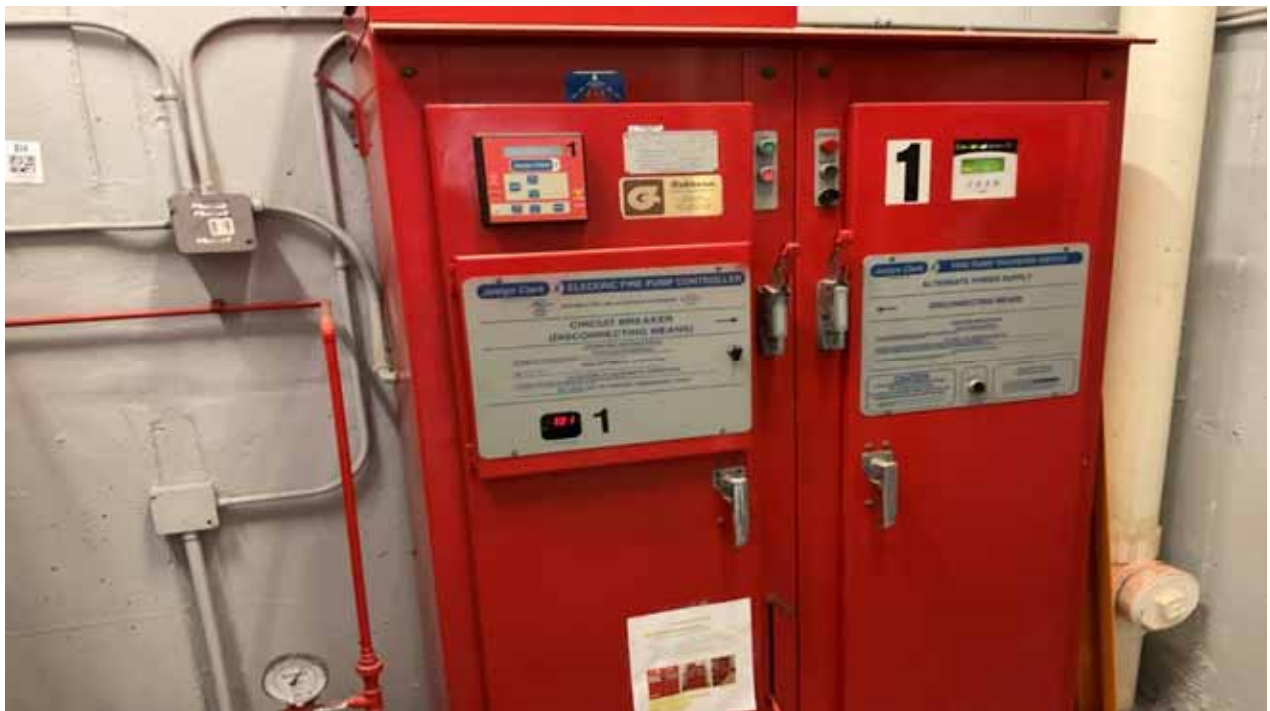
Fire Pump Controller - Low Zone
