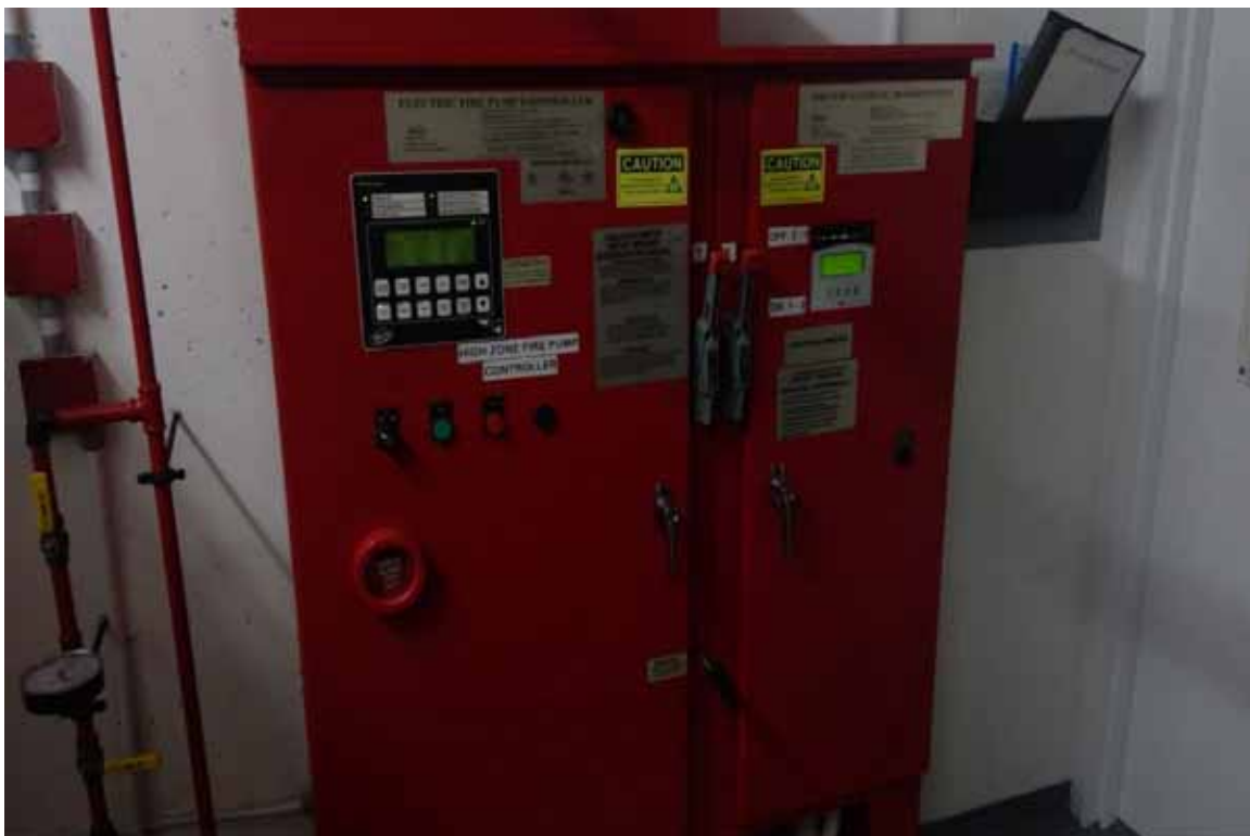
Fire Pump Controller - High Zone
