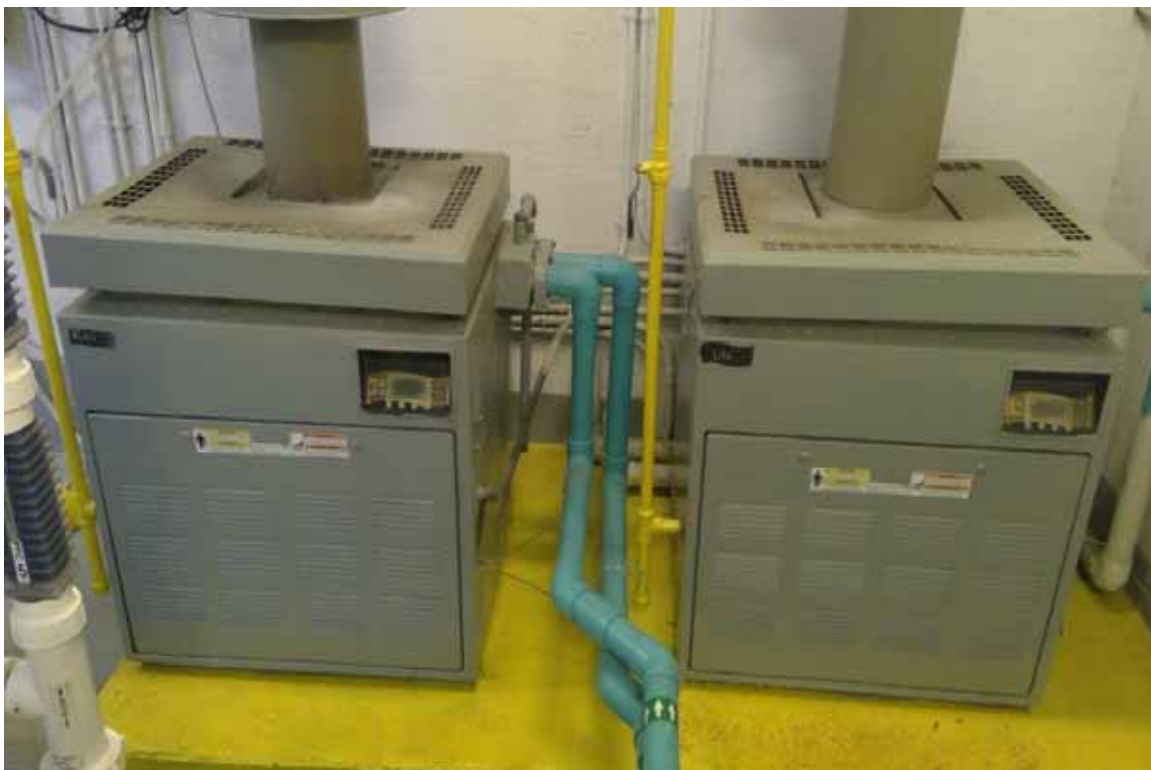
West Pool Equipment, Heaters
