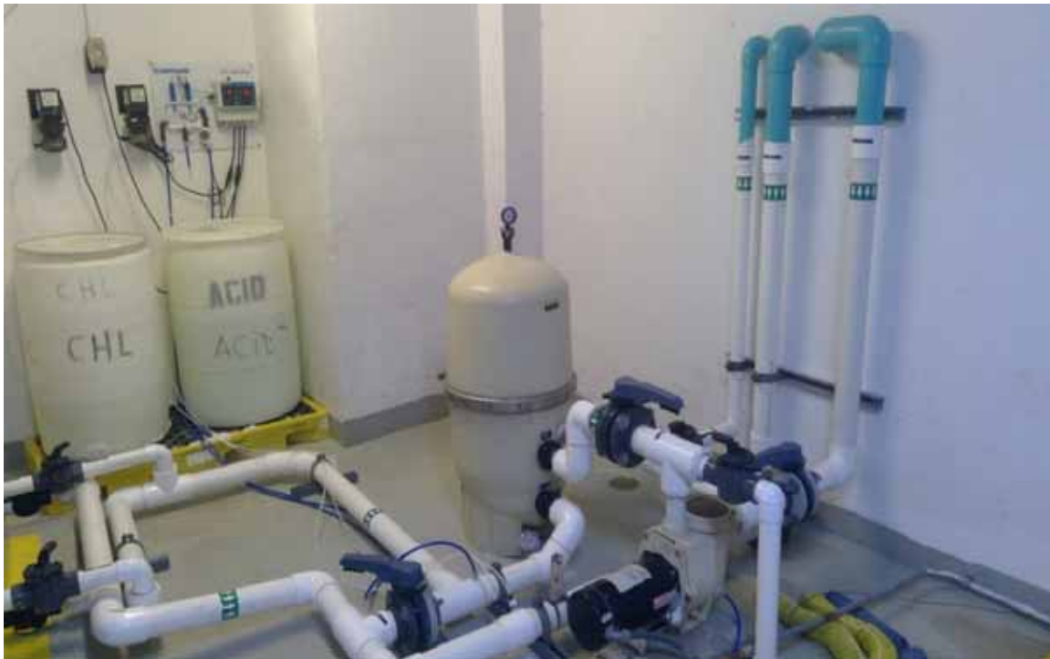
East Pool Equipment
