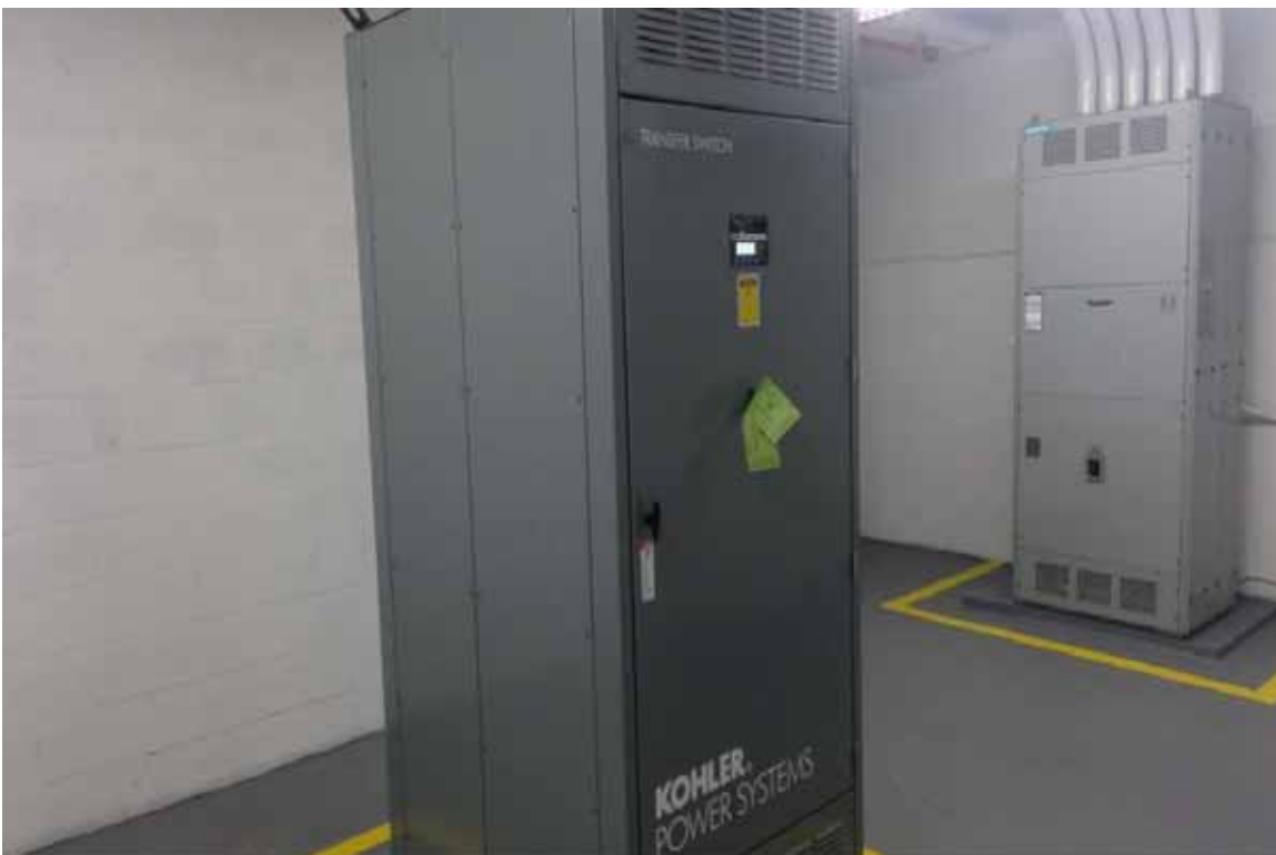
Generator Automatic Transfer Switch
