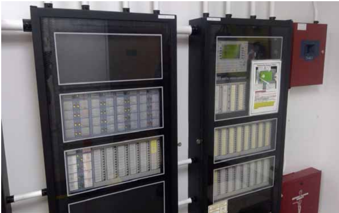
Fire Alarm Panel
