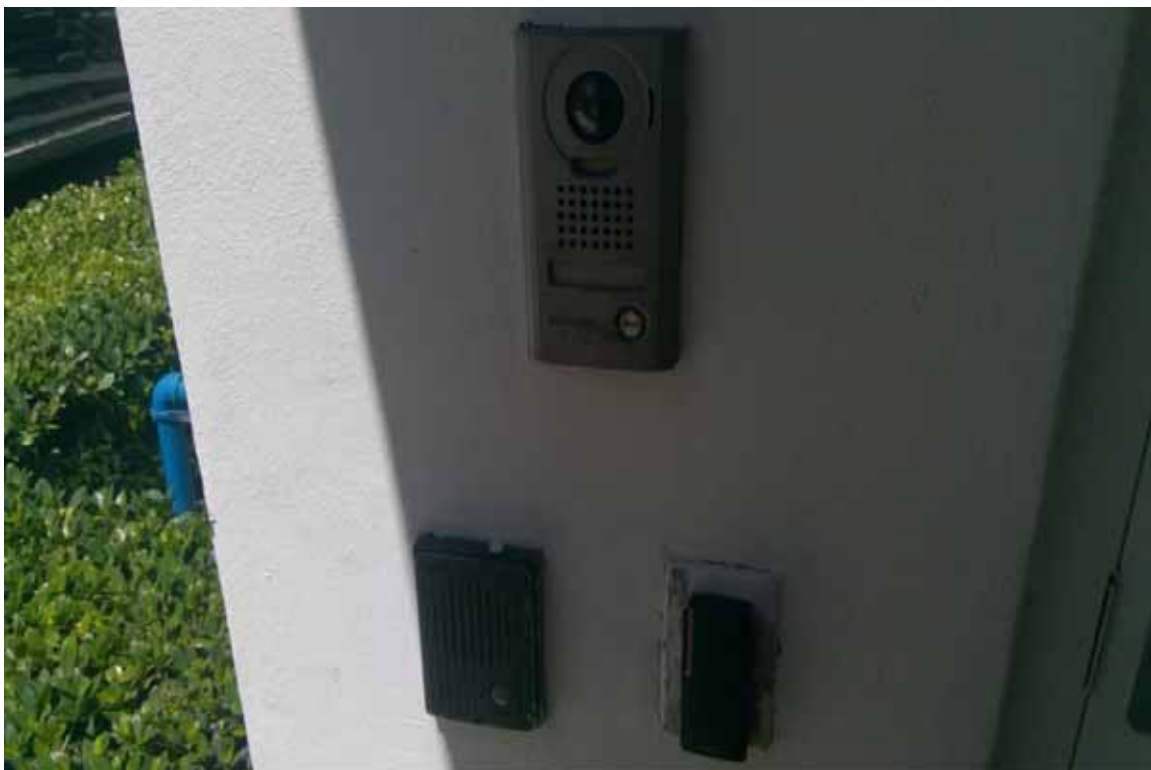
Access Control - FOB Reader & Intercom
