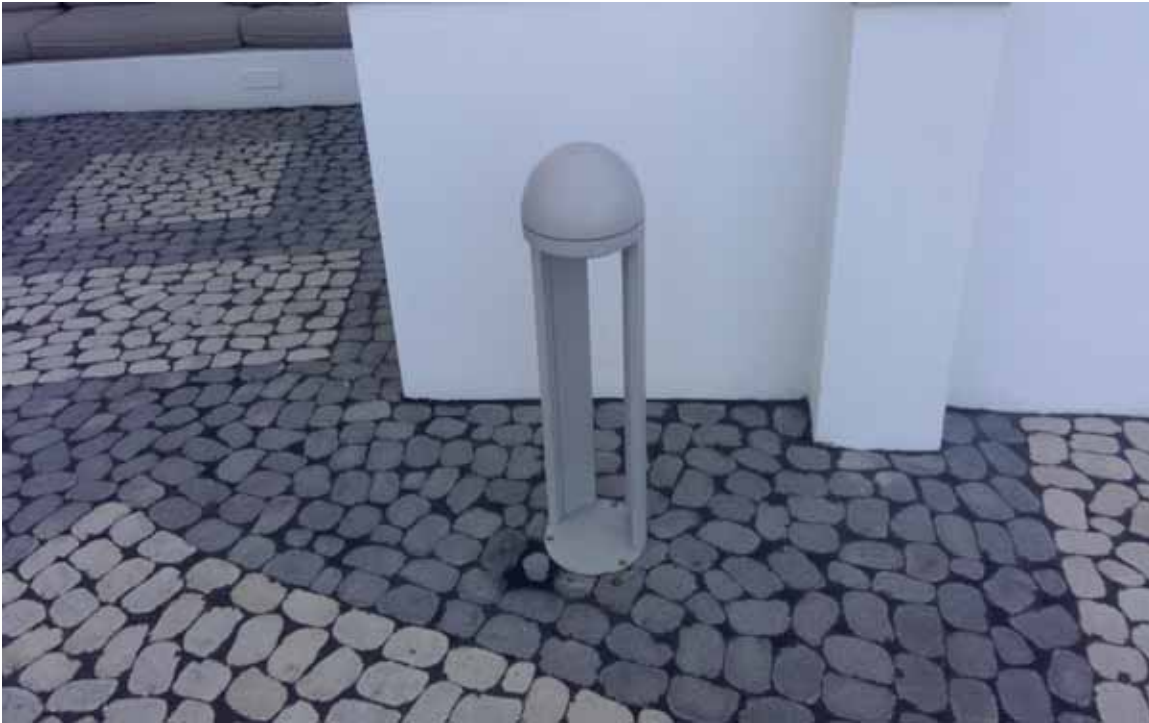
Light Bollard - West Pool Deck
