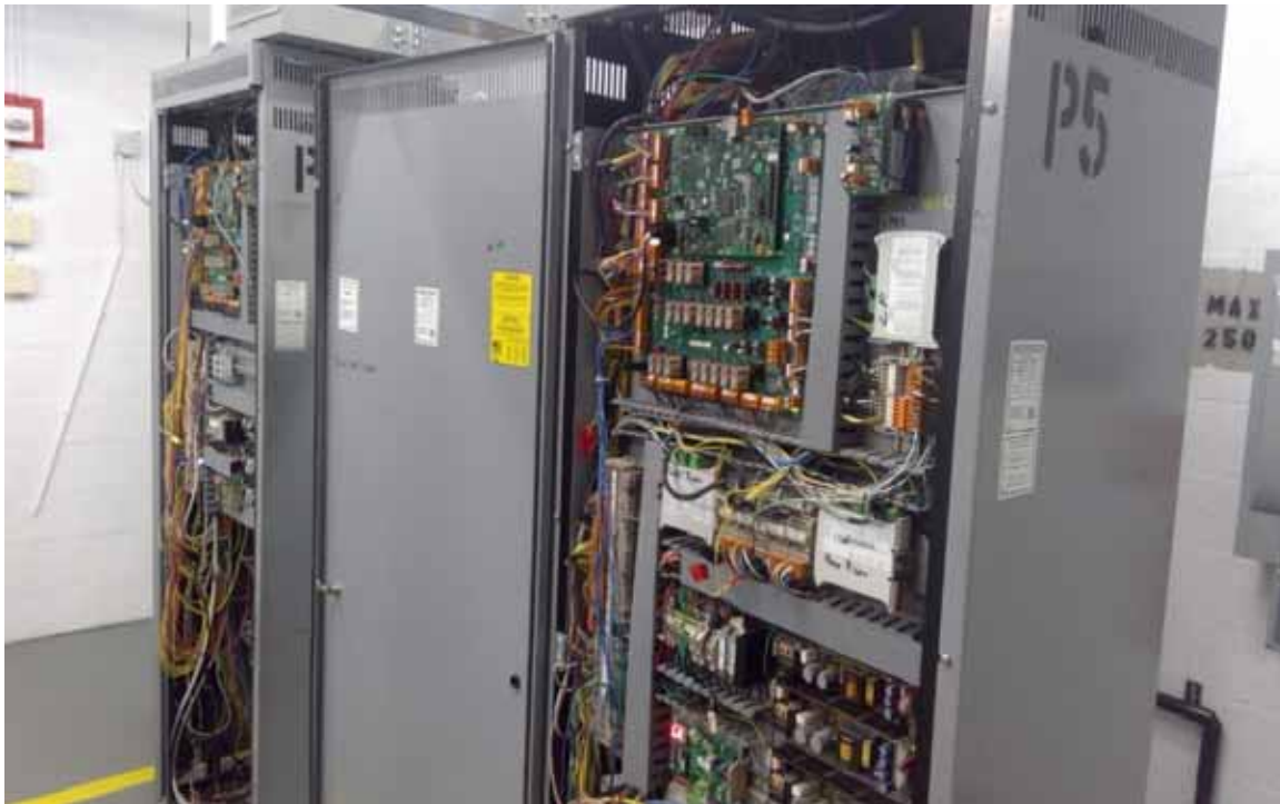
Elevator Equipment P5 & P6
