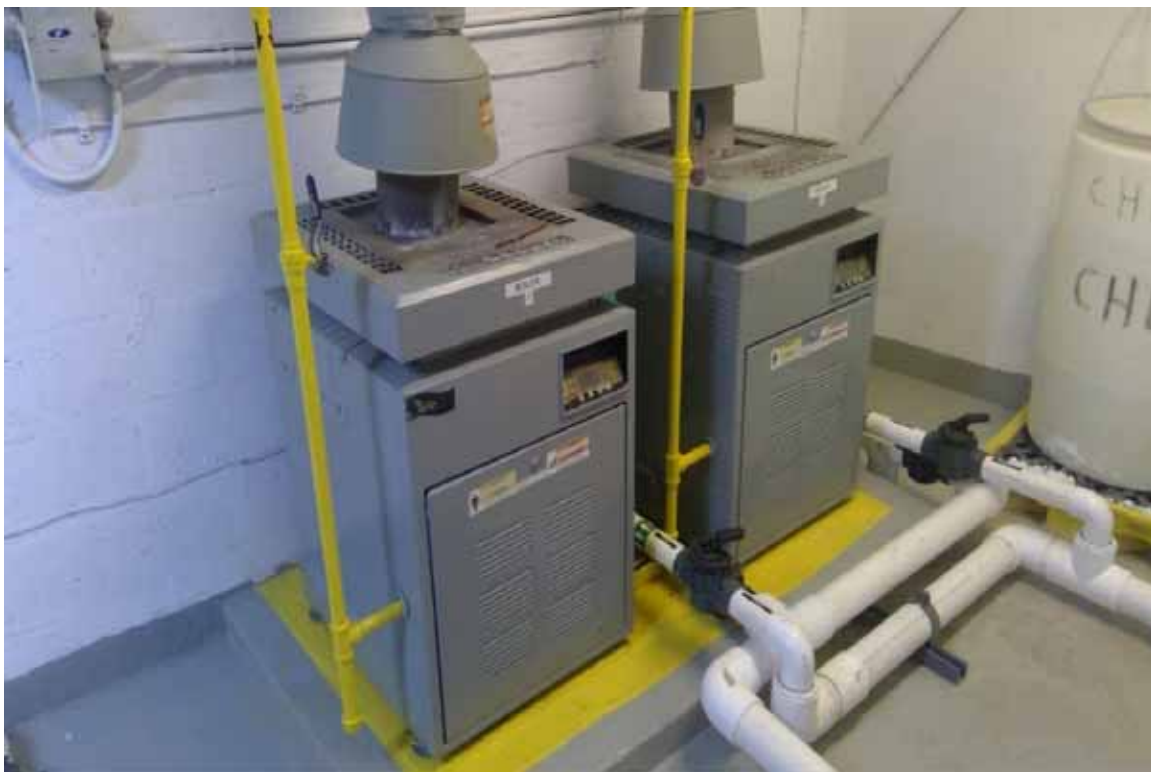
East Pool Equipment, Heaters
