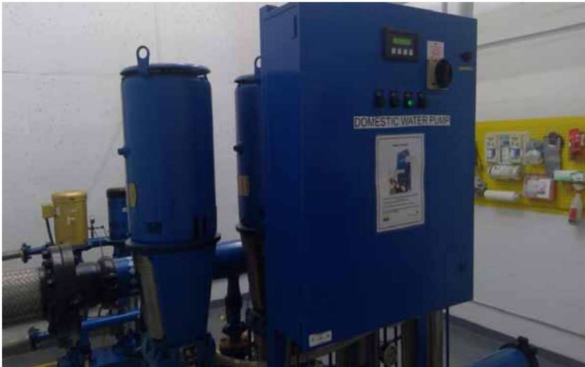
Domestic Water Booster Pump System
