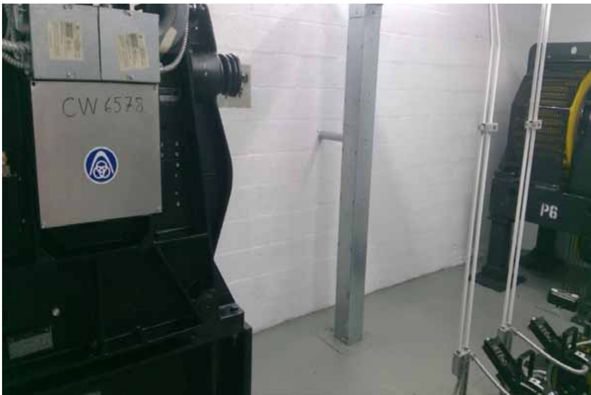
Elevator Equipment P5 & P6
