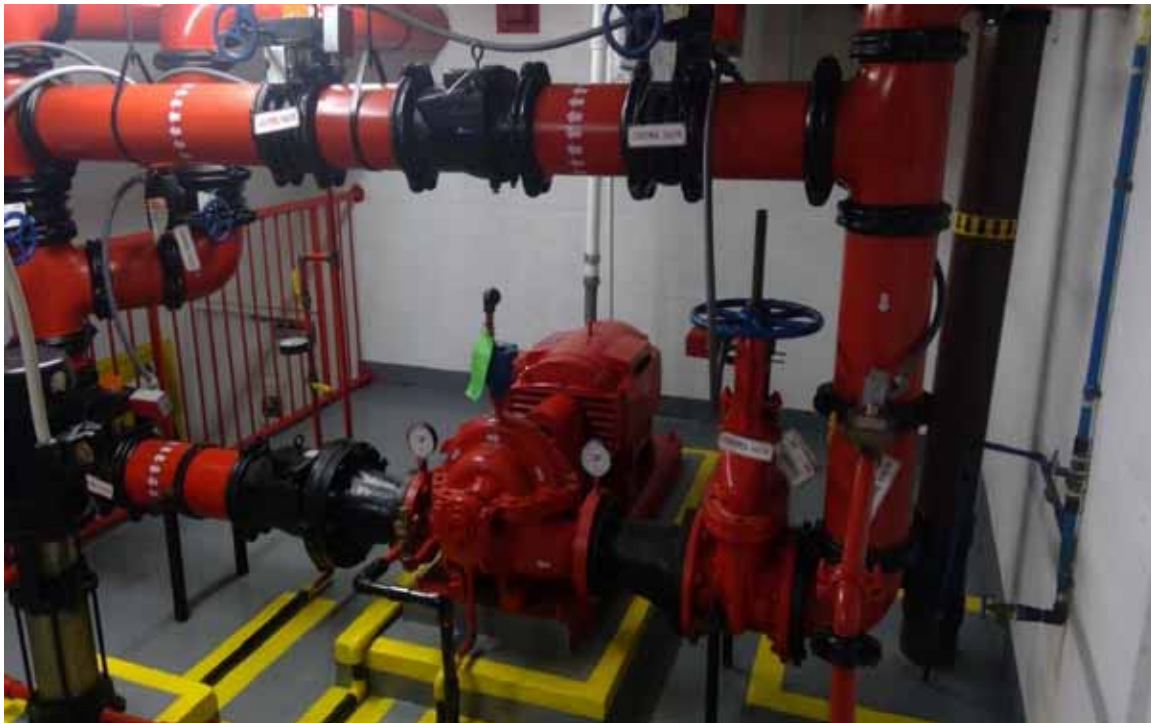
Fire Pump - Low Zone
