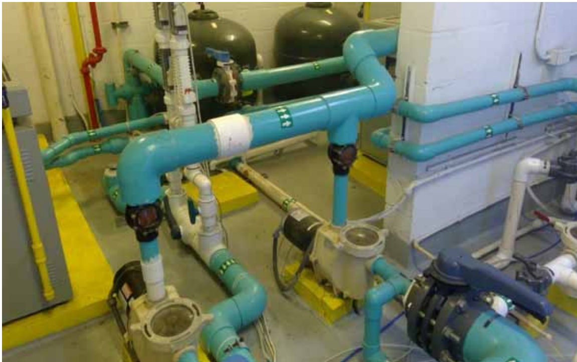
West Pool Equipment
