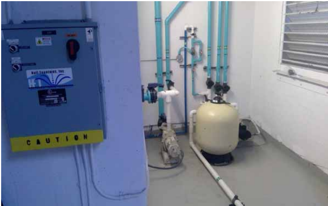
Fountain Equipment - East Pool
