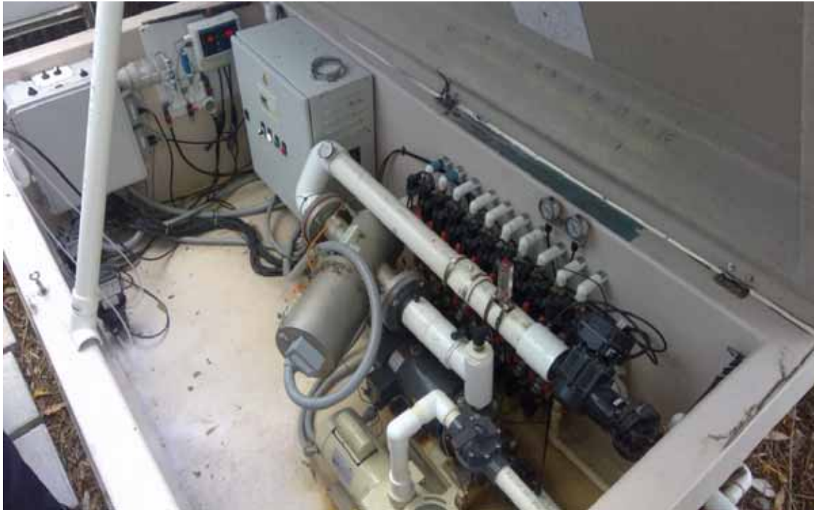
Splash Pad Equipment
