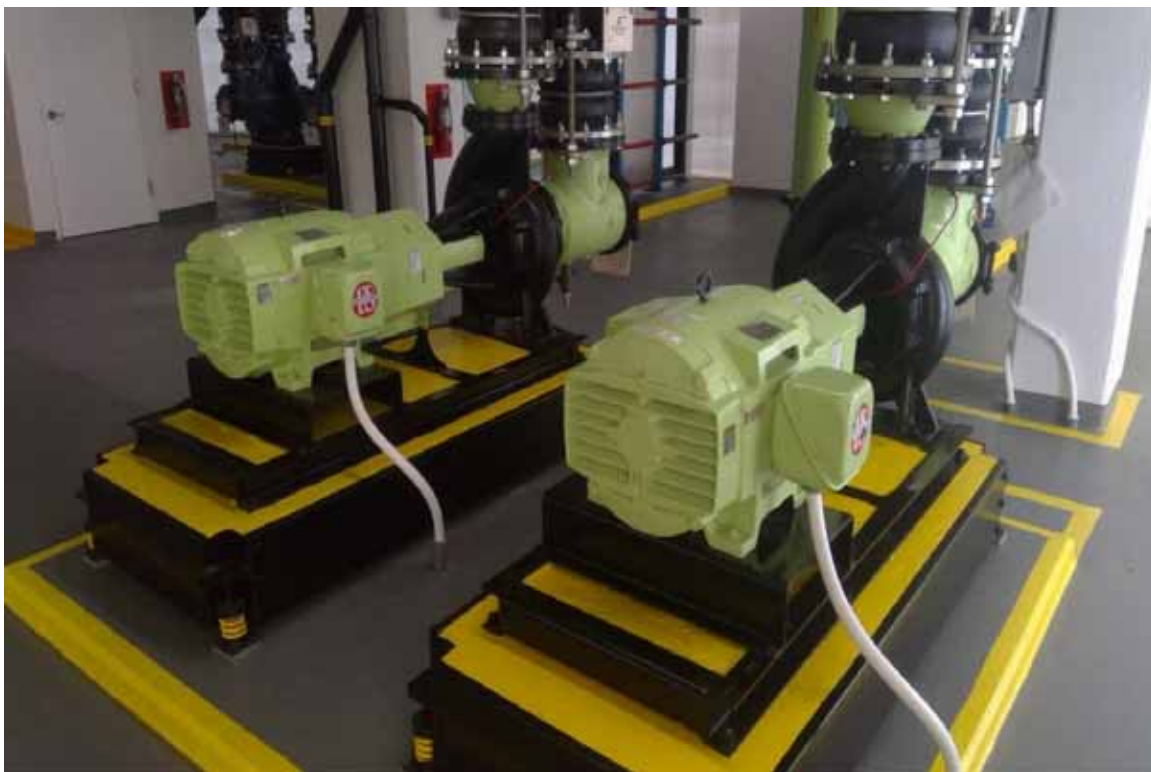
A/C Condensing Pumps - Open Loop
