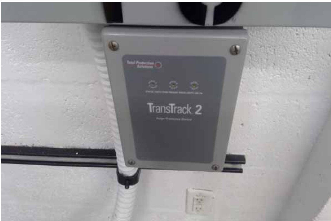
Surge Protective Device - Elevator System
