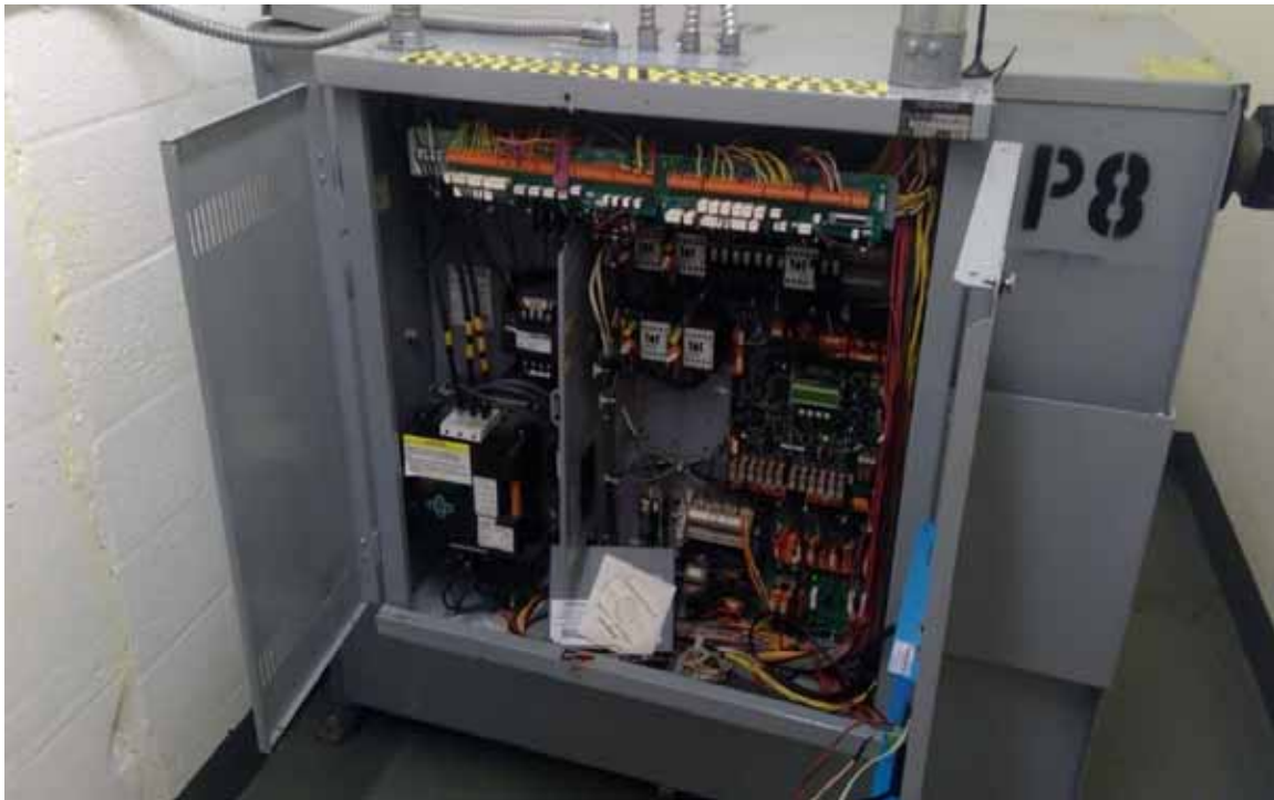
Elevator Equipment P8
