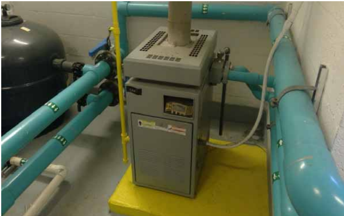
Spa Equipment, Heater
