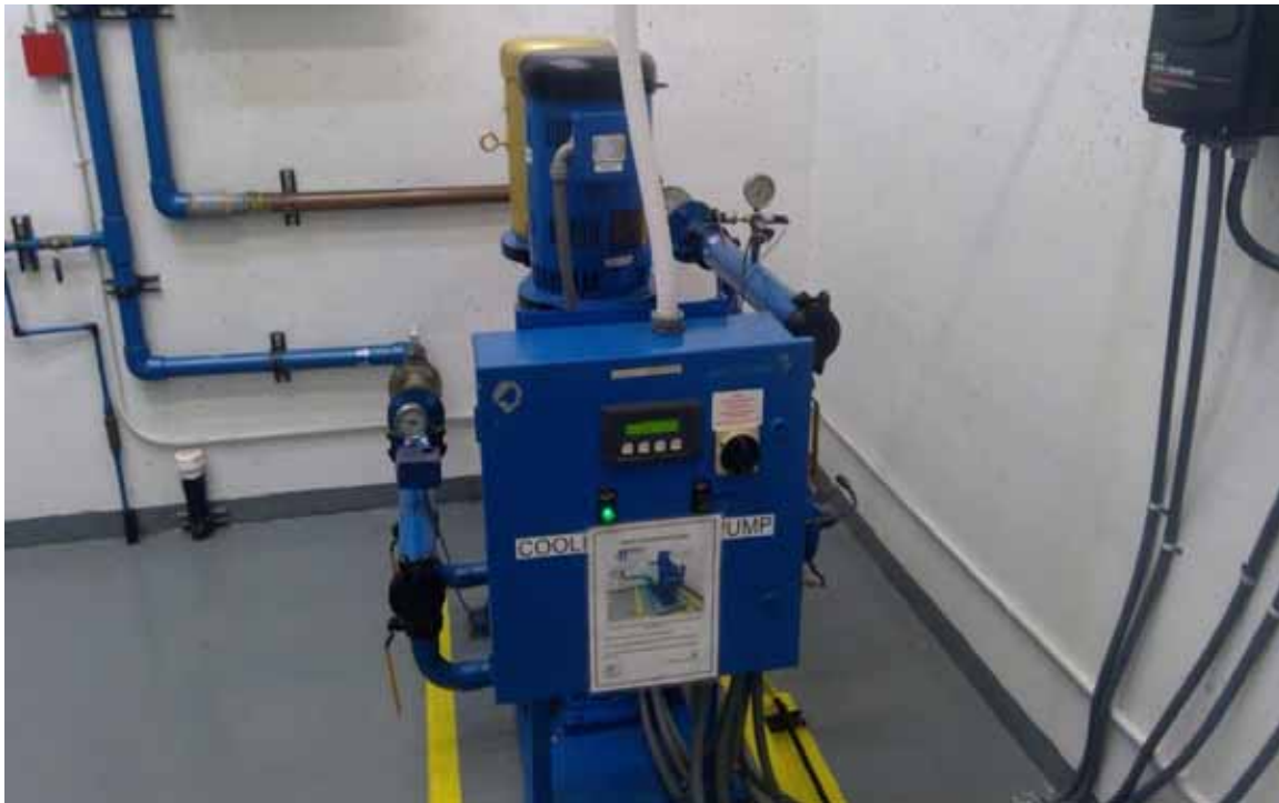
A/C Cooling Tower Makeup Pump System
