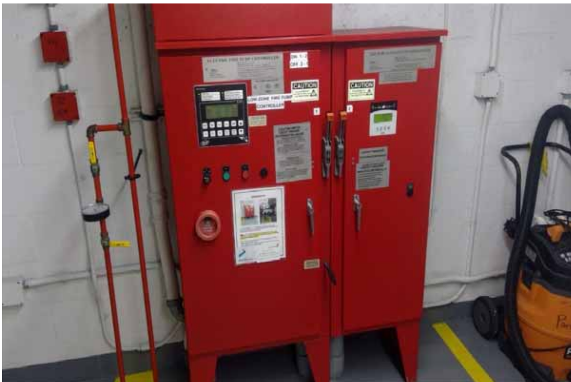
Fire Pump Controller - Low Zone
