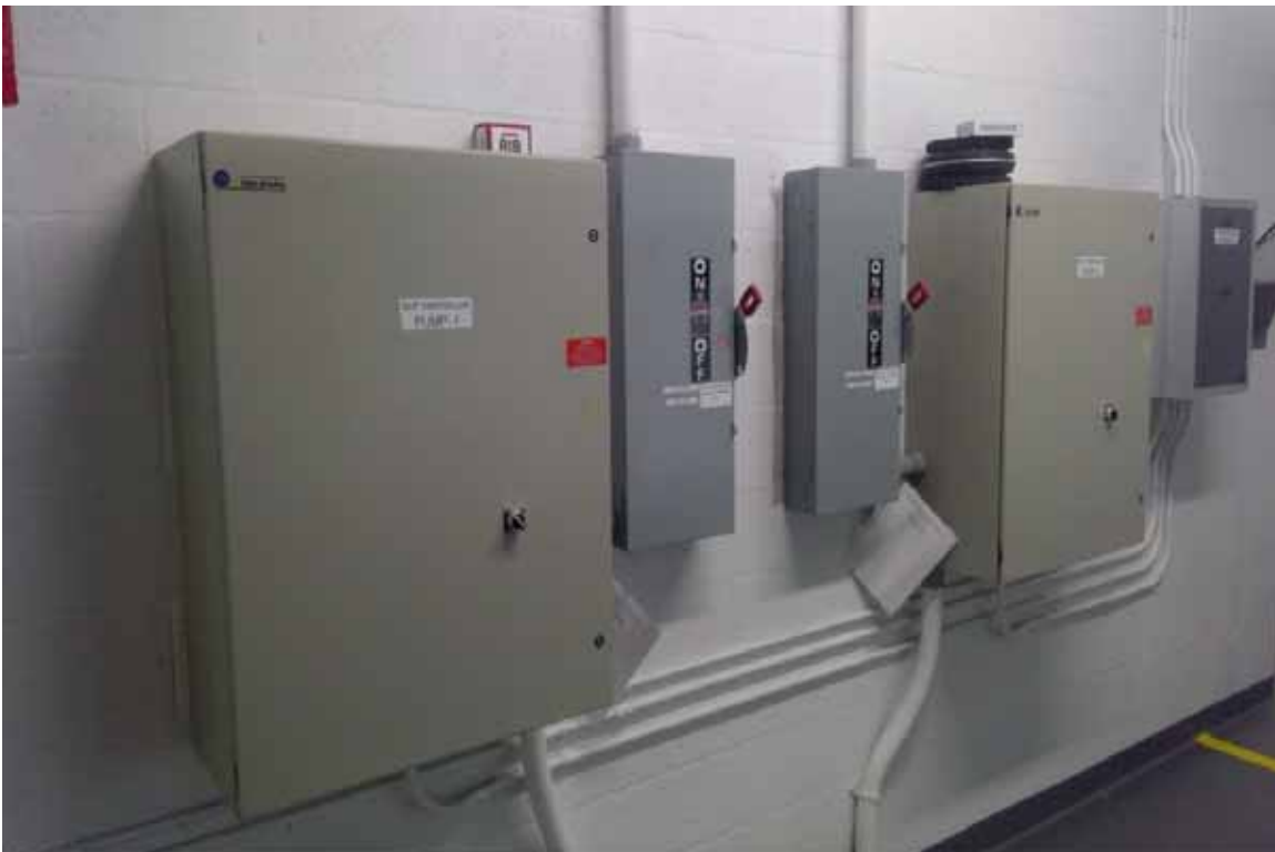
Variable Frequency Drives - Closed Loop Pumps
