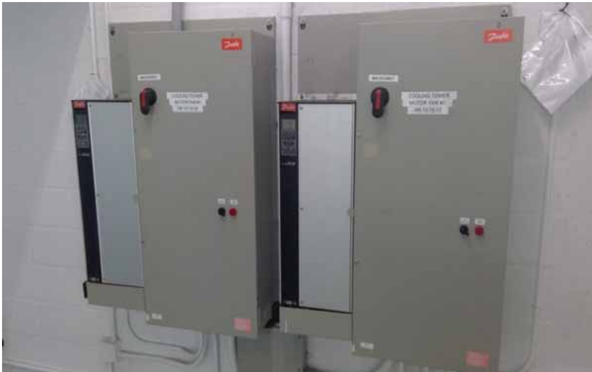
Variable Frequency Drives - A/C Cooling Tower
