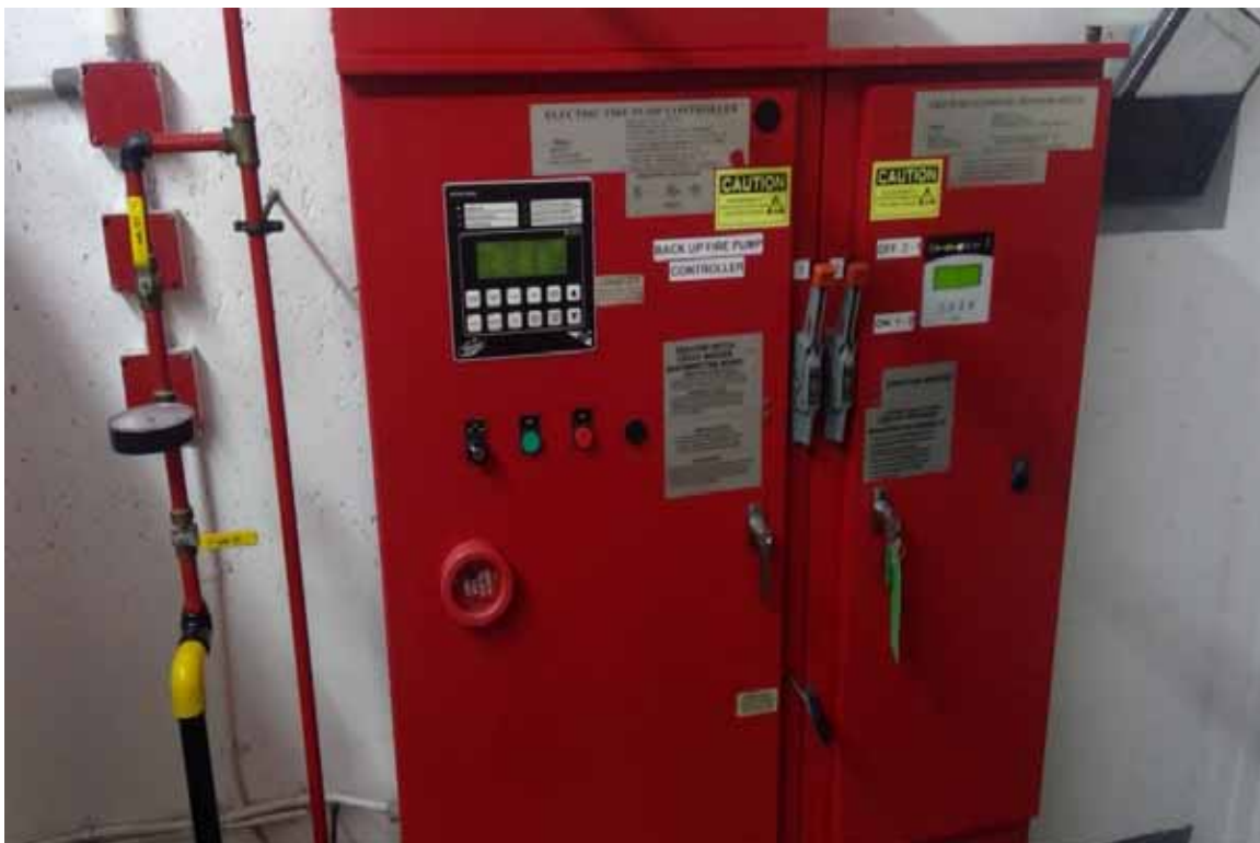
Fire Pump Controller - Back Up
