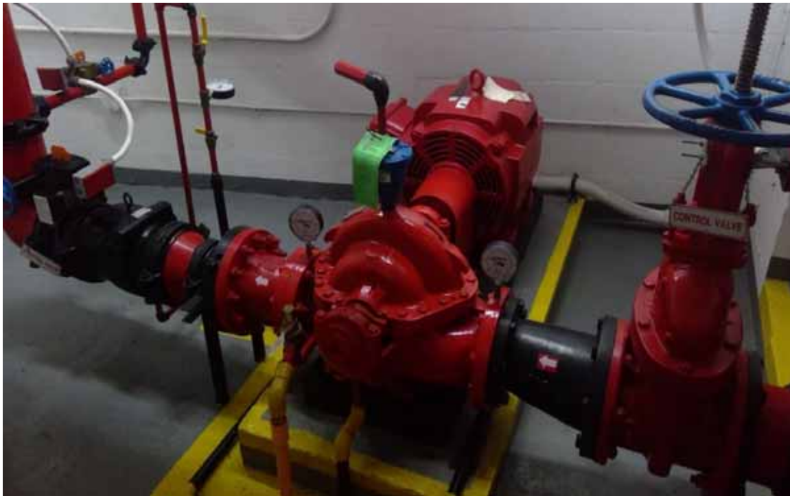
Fire Pump - High Zone
