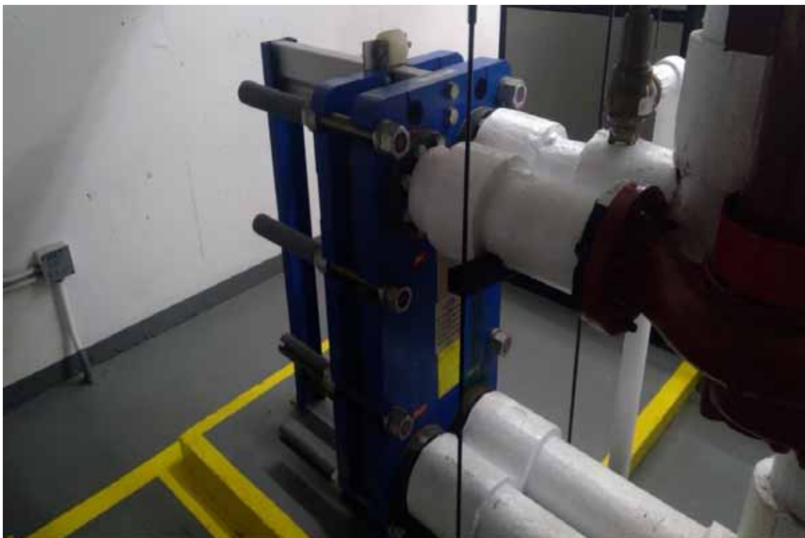
Heat Exchanger - Hot Water
