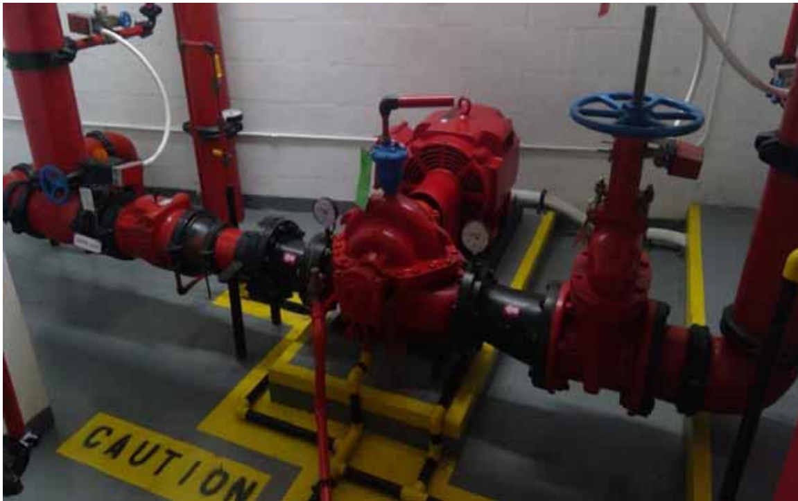
Fire Pump - Back Up
