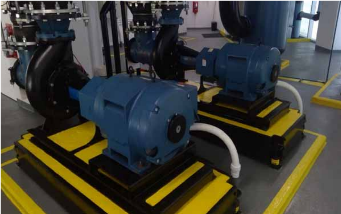
A/C Condensing Pumps - Closed Loop
