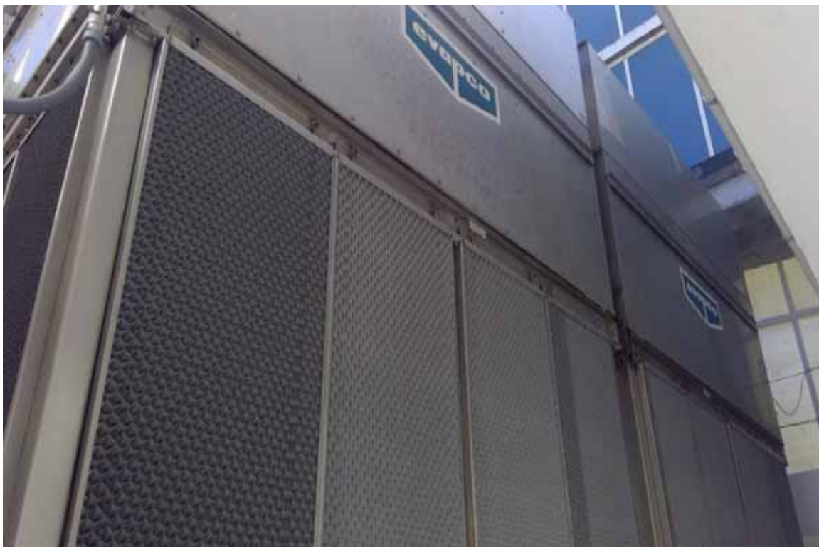
A/C Cooling Towers
