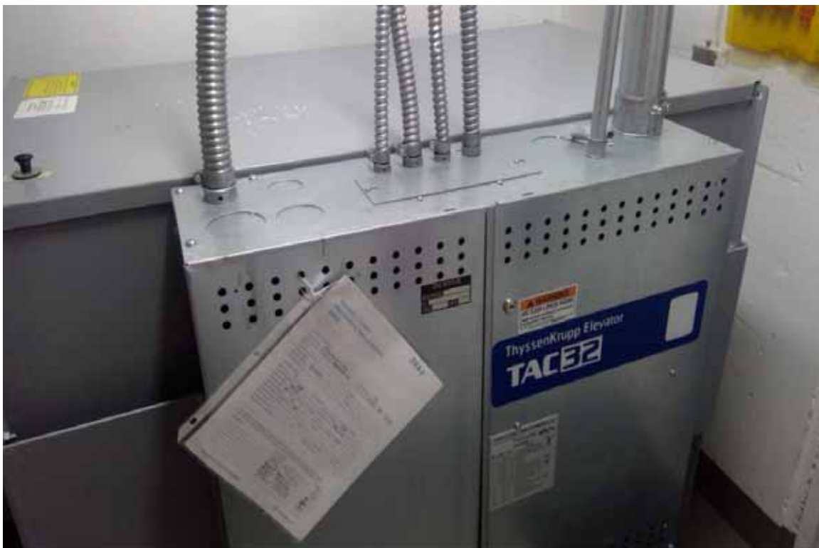
Elevator Equipment P7
