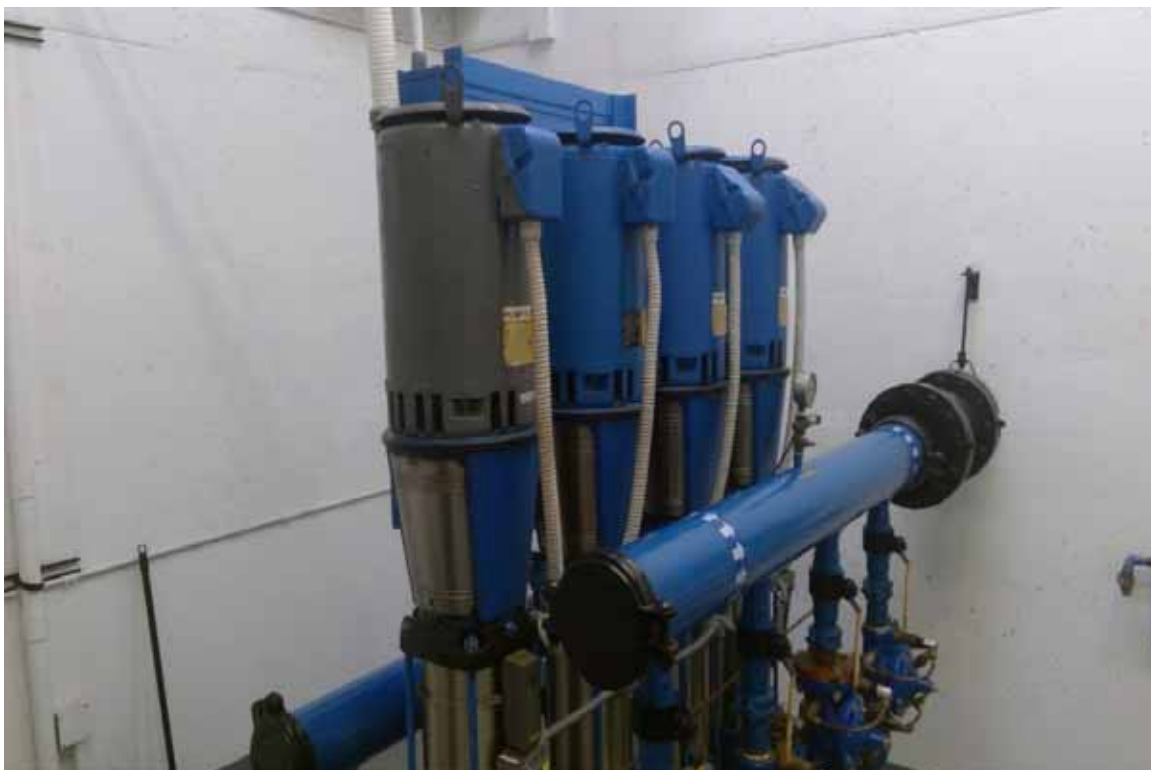
Domestic Water Booster Pump System
