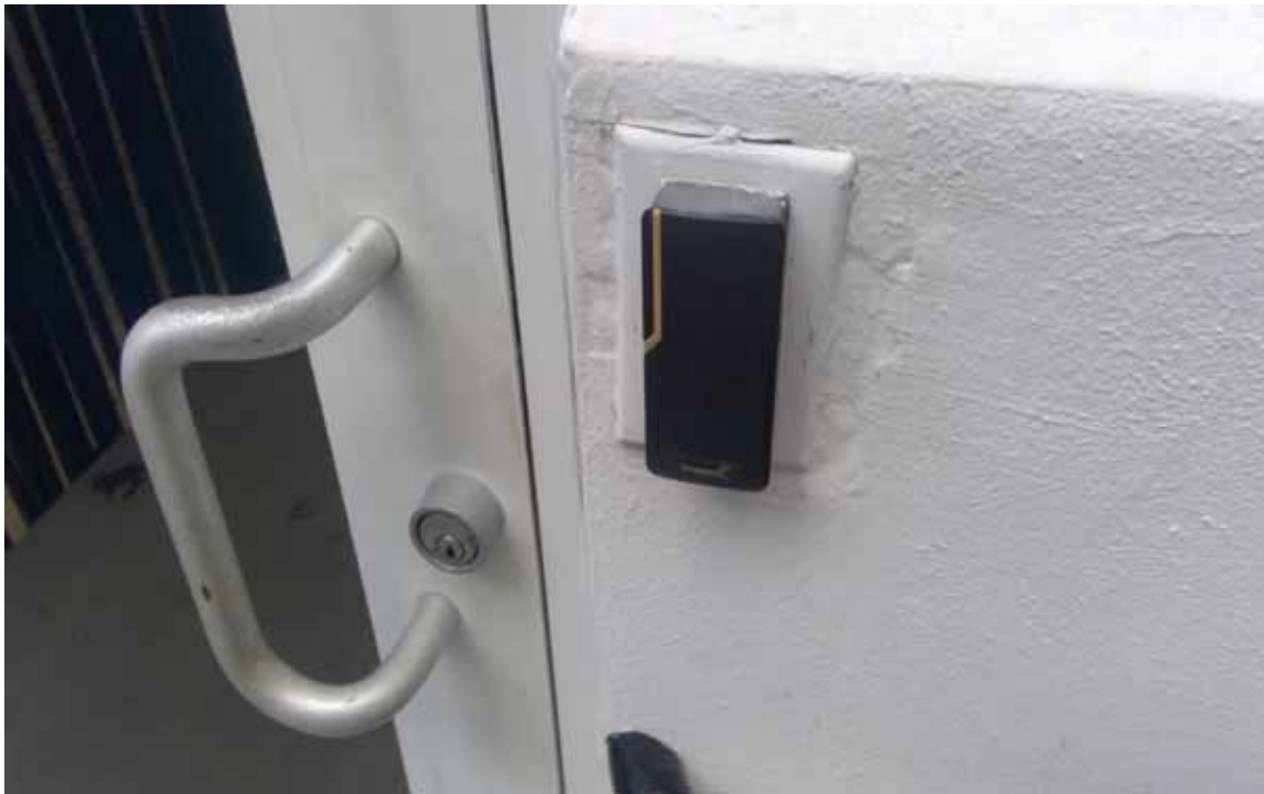
Access Control - FOB Reader
