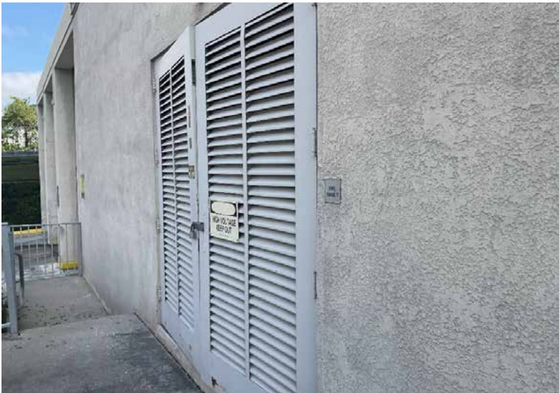
Doors - FPL Vault
