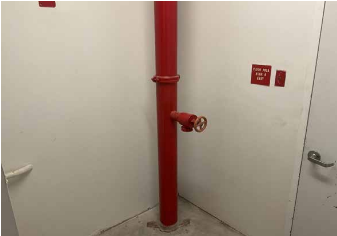
Fire Standpipe - Condo Bldg
