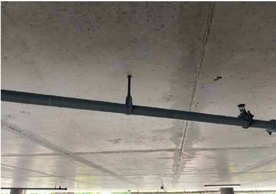
Fire Sprinkler Pipe Hanger - Garage
