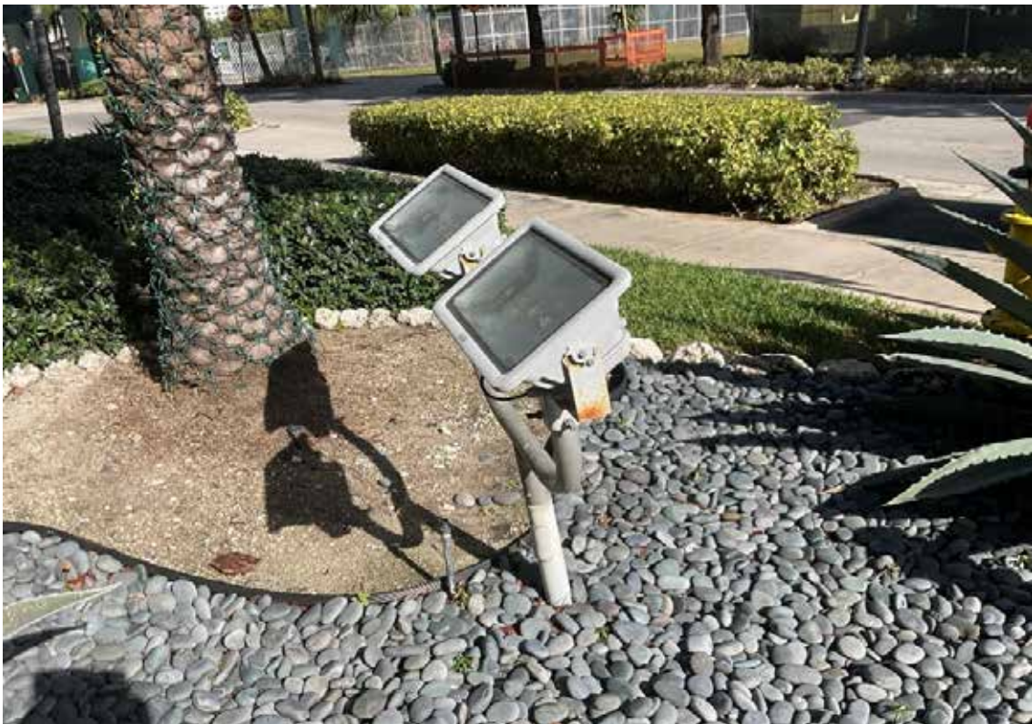
Light Fixtures, Spotlight - Condo Bldg
