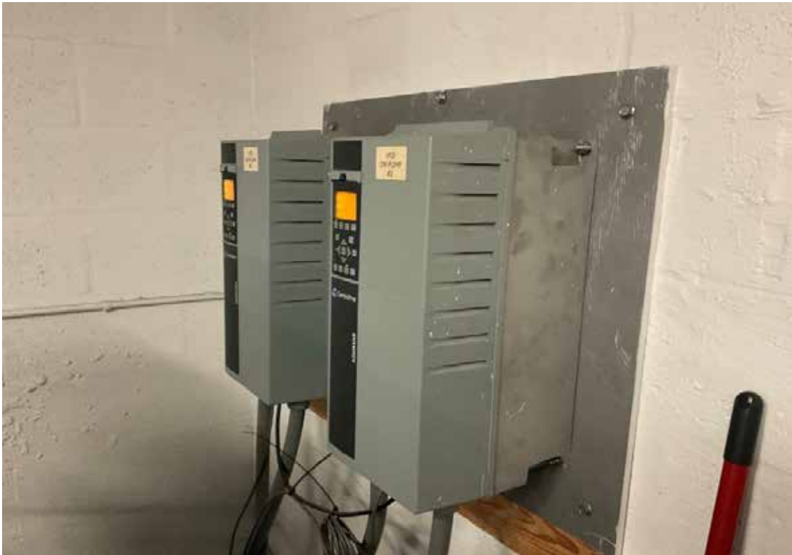
Variable Frequency Drives - Domestic Water System
