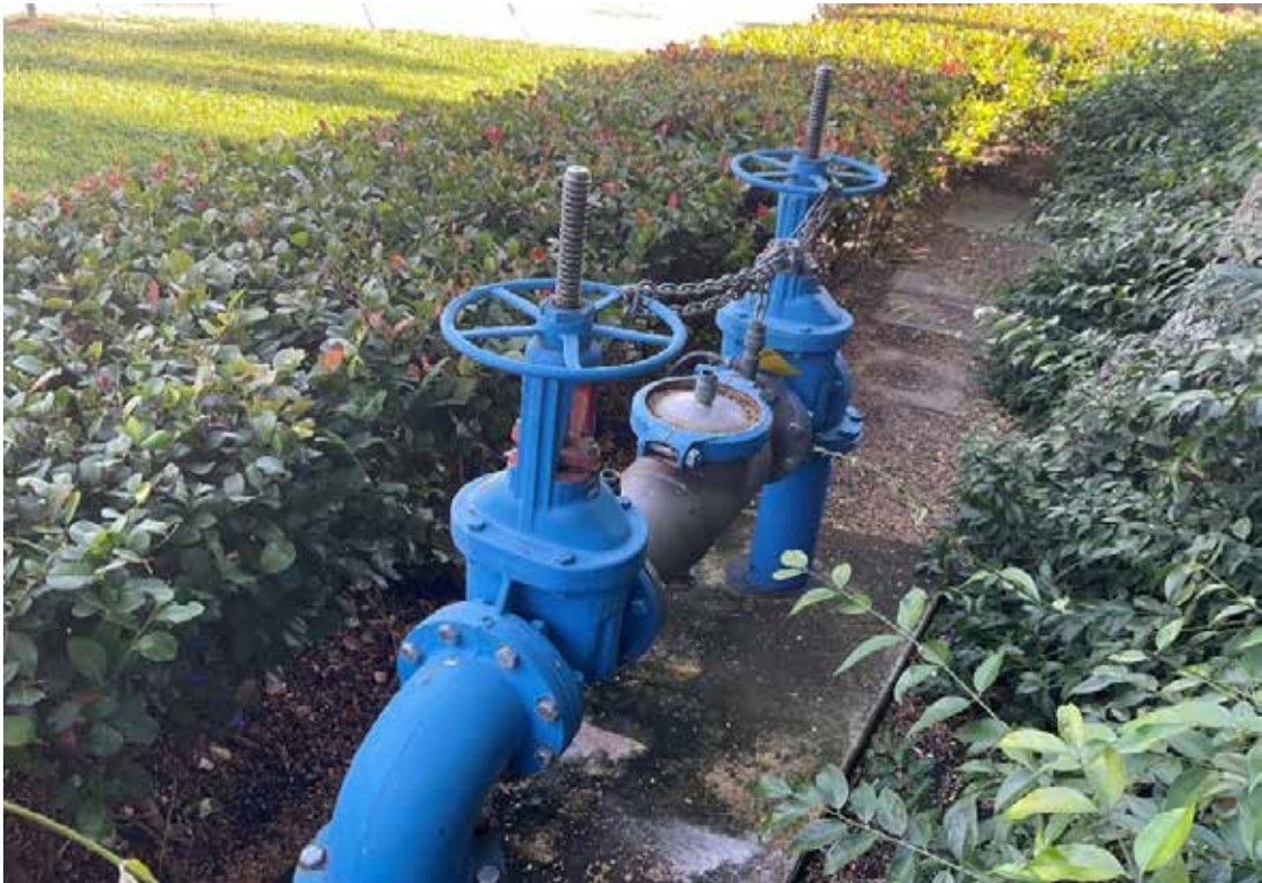
Backflow Preventer - Domestic Water
