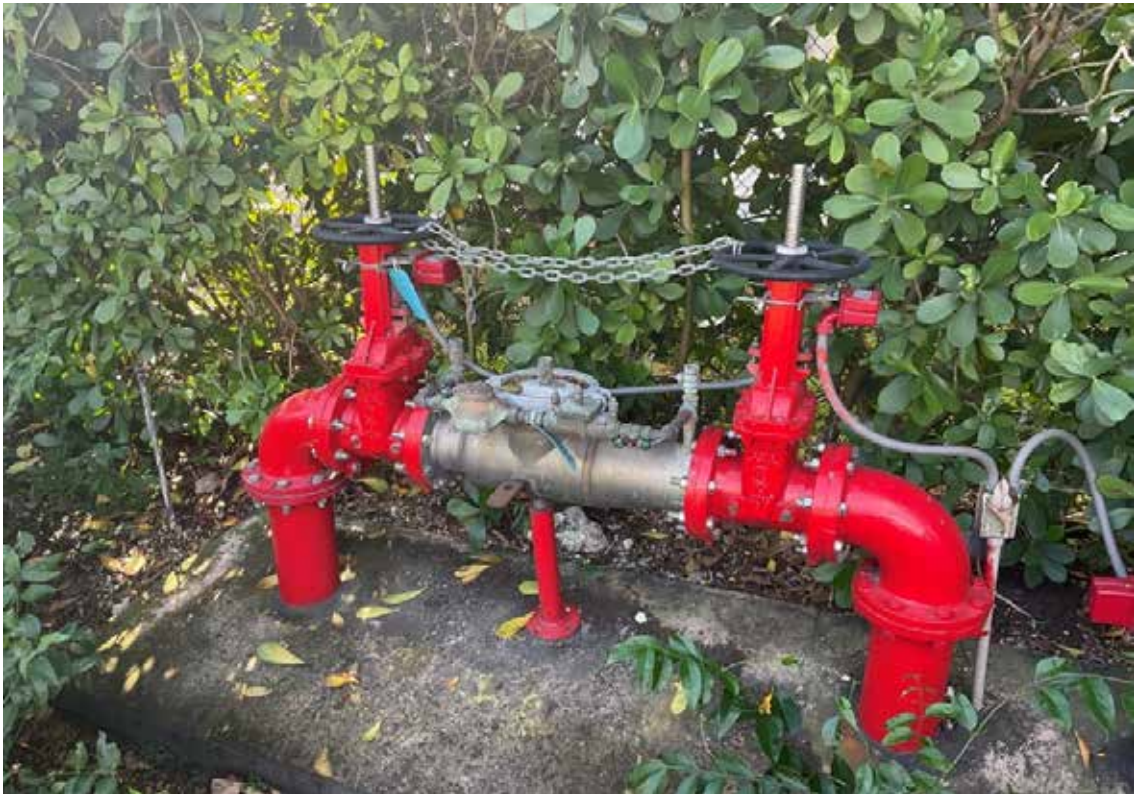
Backflow Preventer - Fire
