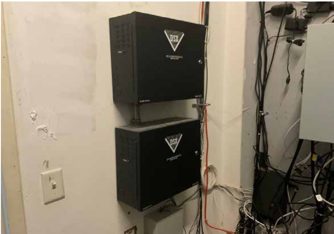
Access Control Equipment
