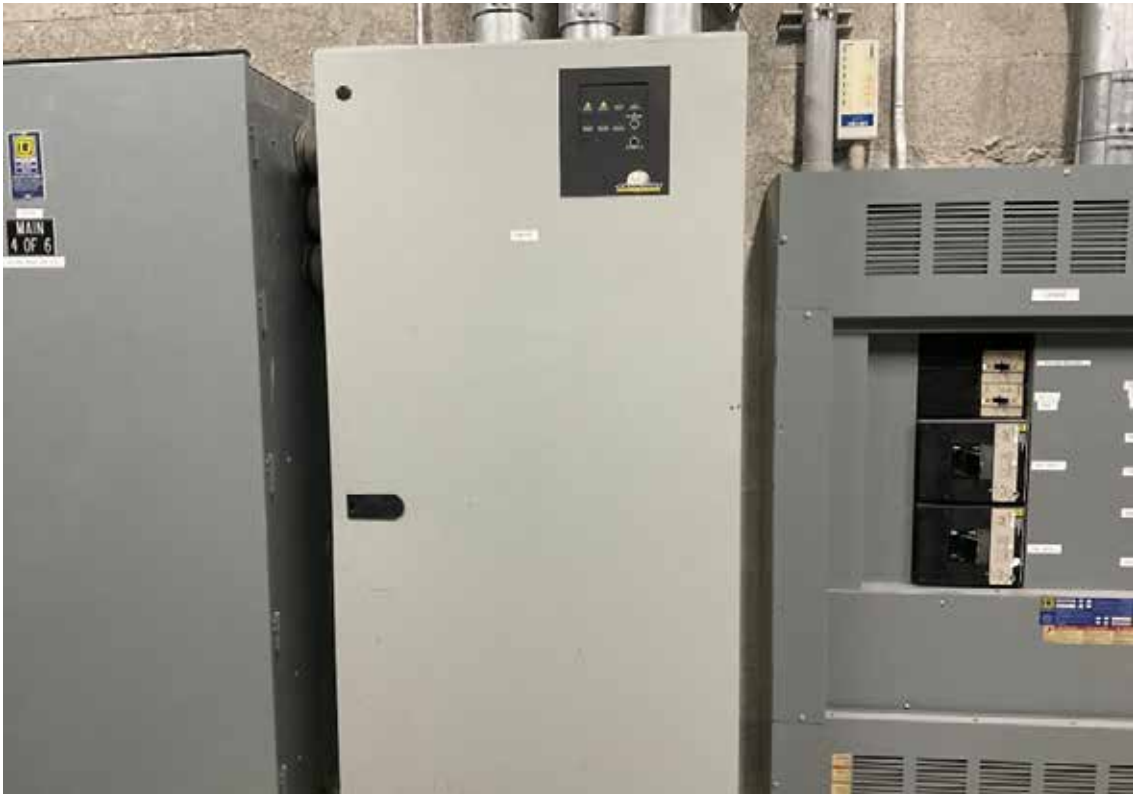
Generator Transfer Switch
