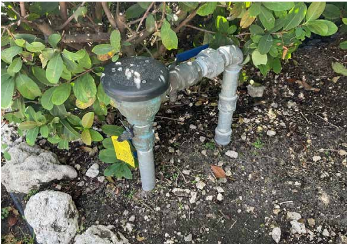
Backflow Preventer - Irrigation
