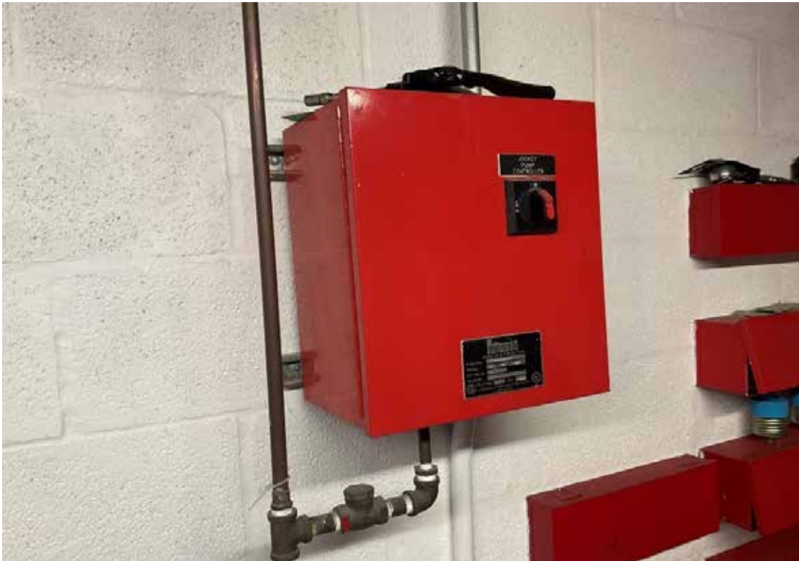
Fire Jockey Pump Controller
