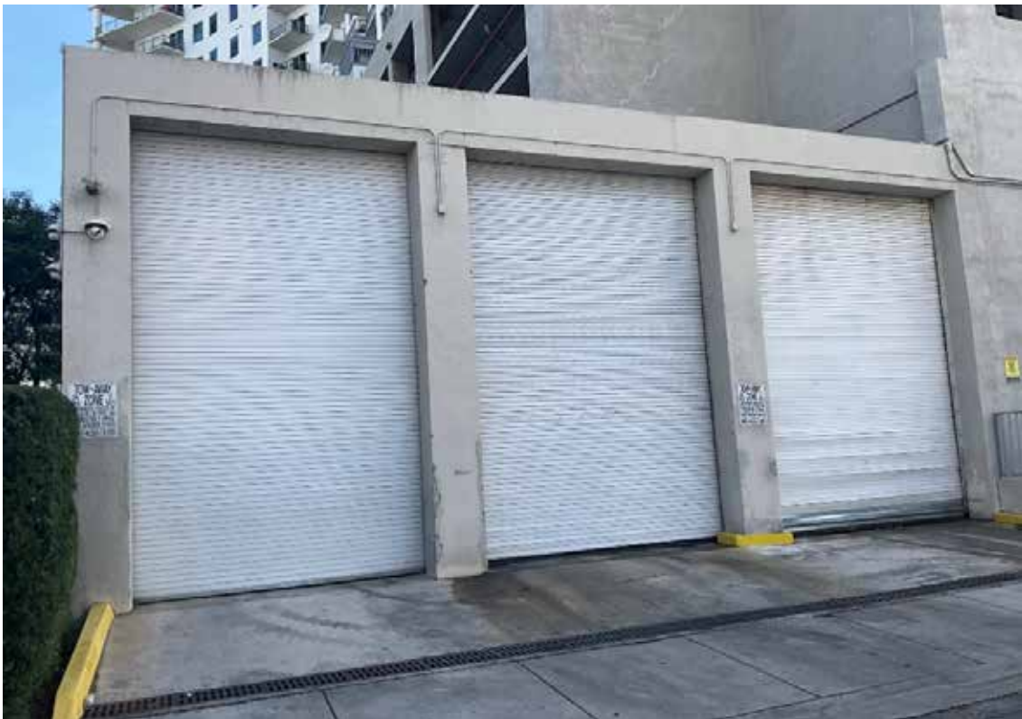
Doors, Roll-up - Service Area
