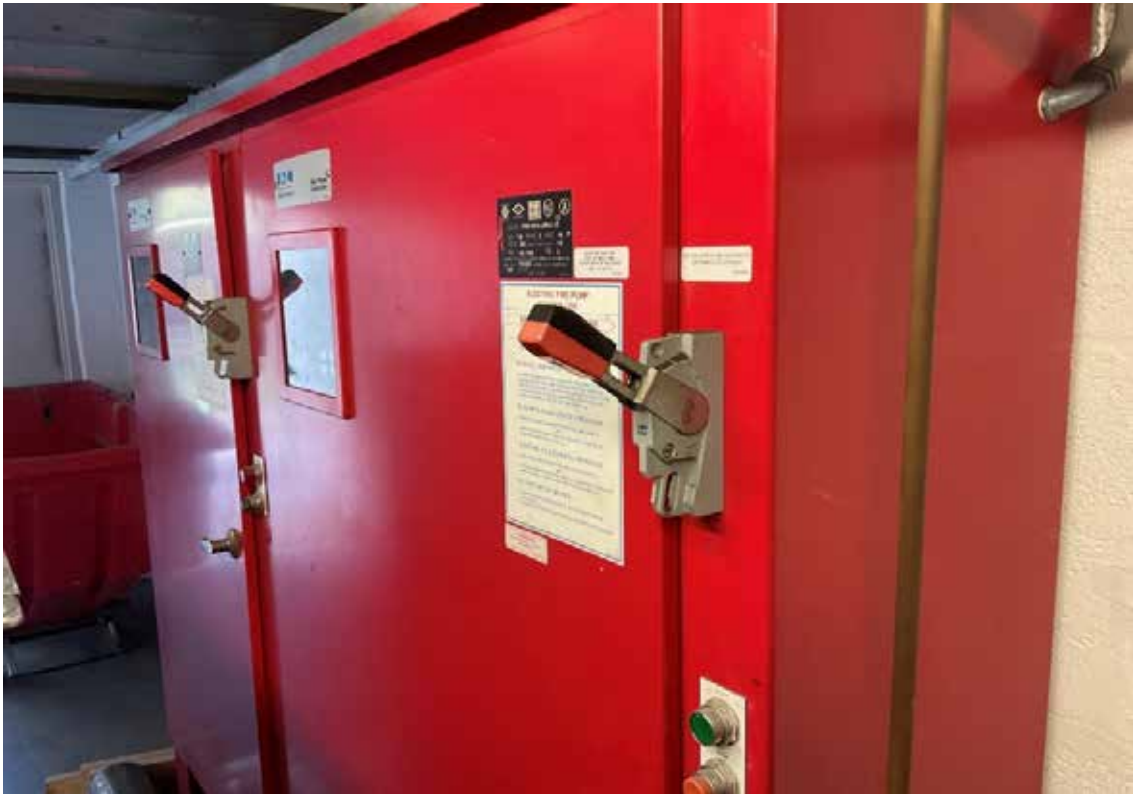
Fire Pump Controller
