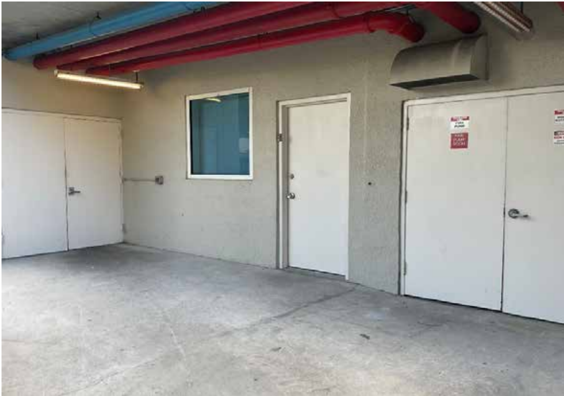
Doors - Maintenance Office & Fire Pump Room
