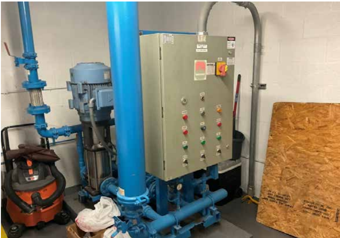
Domestic Water Booster Pump System
