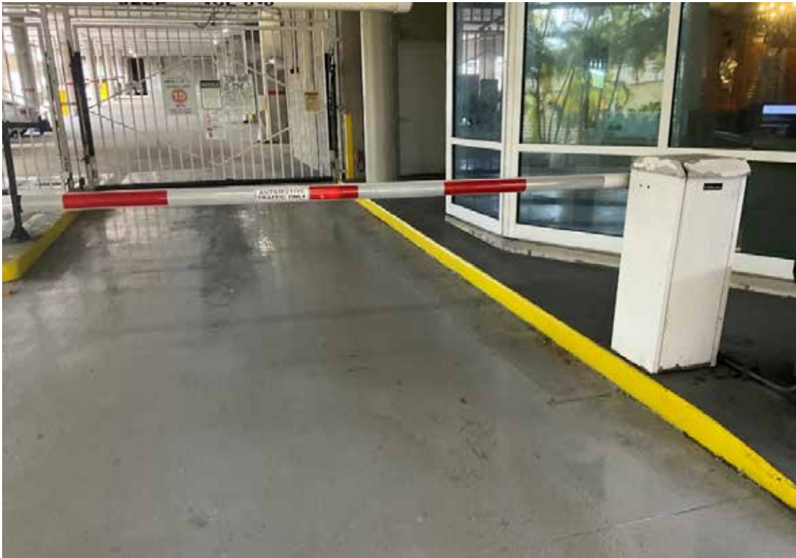
Gate Barrier Operator - Garage
