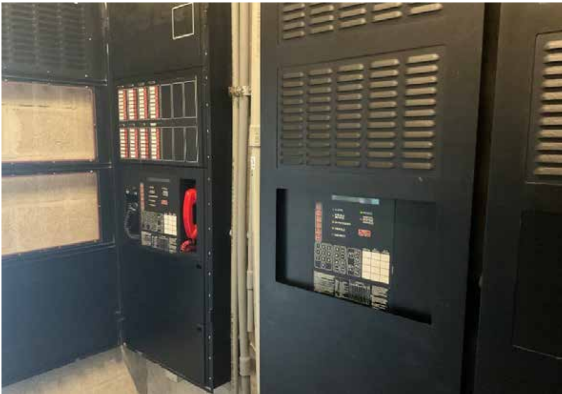
Fire Alarm Panels
