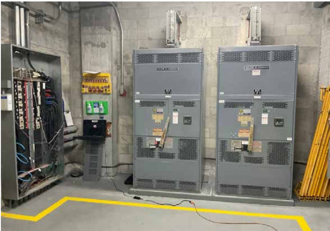
Main Electrical Room
