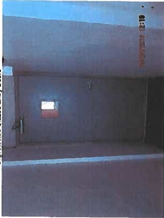
Unprotected Glazed Entry Door
