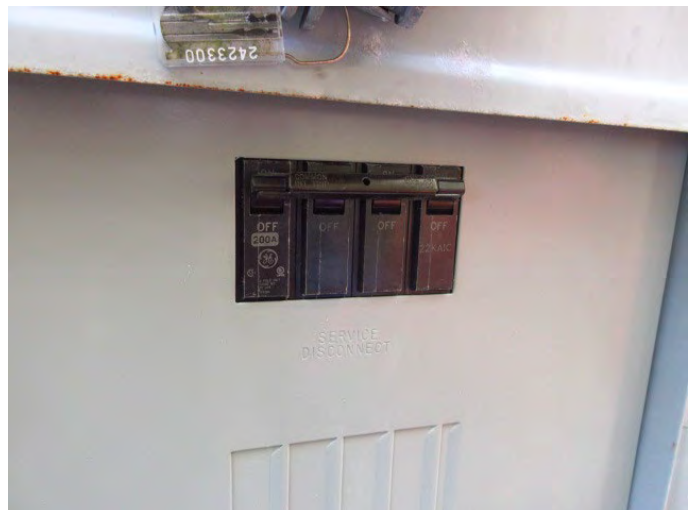
VIEW OF ELECTRICAL EQUIPMENT
