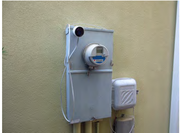
VIEW OF ELECTRICAL EQUIPMENT
