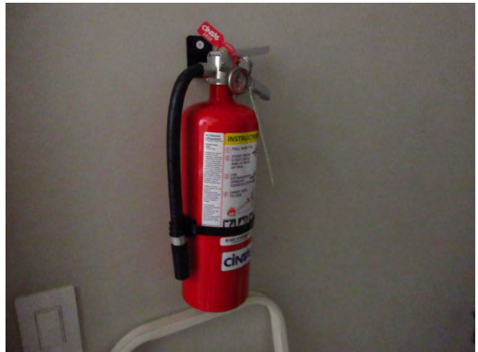
VIEW OF UNIT FIRE EXTINGUISHER
