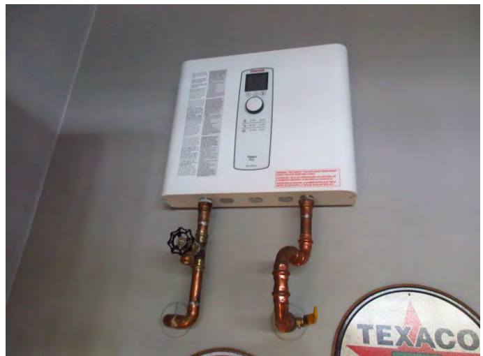
GENERAL VIEW OF UNIT WATER HEATER
