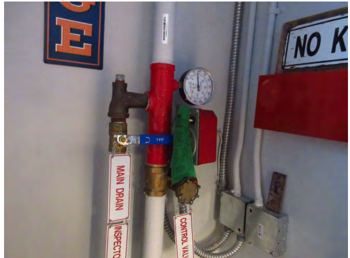
VIEW OF UNIT FIRE SUPPRESSION SYSTEM
