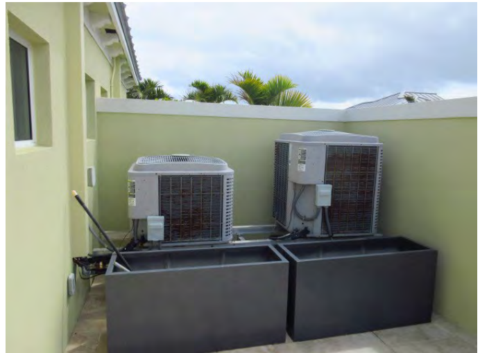
VIEW OF UNIT HVAC EQUIPMENT
