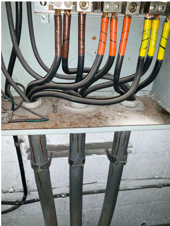
PHOTO-11 Service Conductors/Raceways
