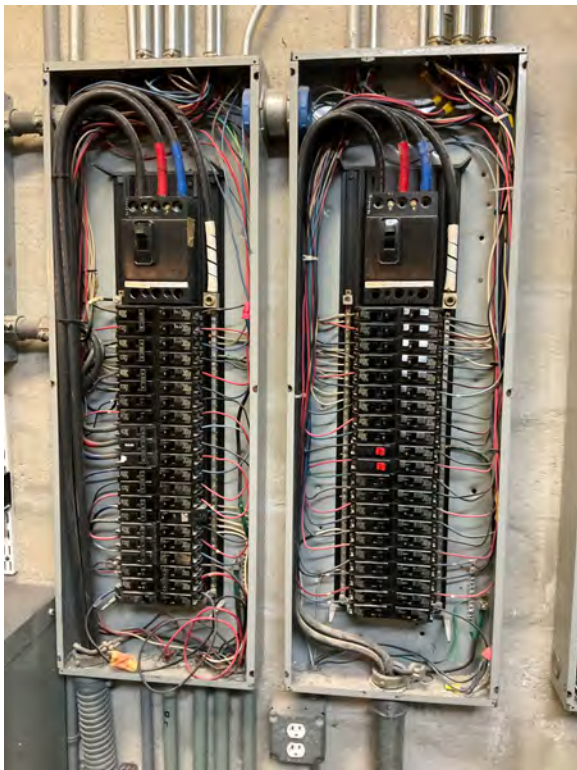
PHOTO-07 Electrical Panels
