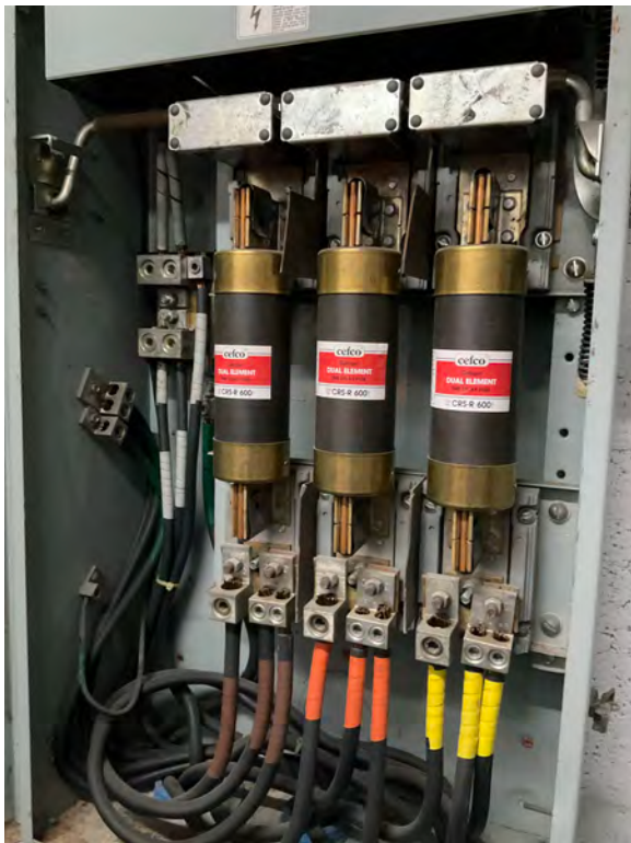
PHOTO-03 Electrical Service
