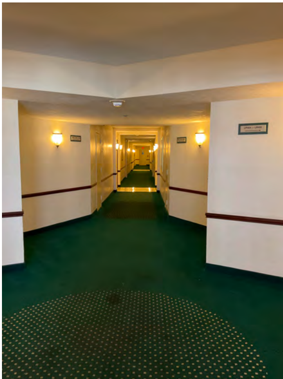
PHOTO-19 Existing Building Egress Lighting
