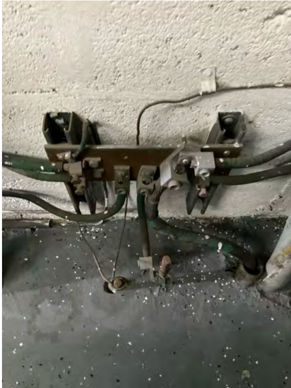
PHOTO-09 Grounding of Service
