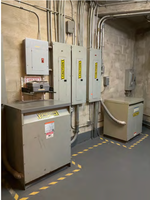
PHOTO-05 Electric Room
