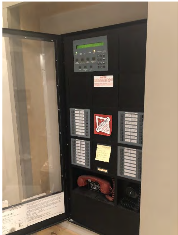
PHOTO-20 Existing Fire Alarm System
