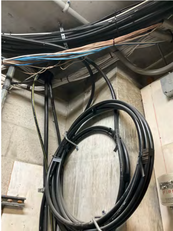
PHOTO-13 Wire and Cables
