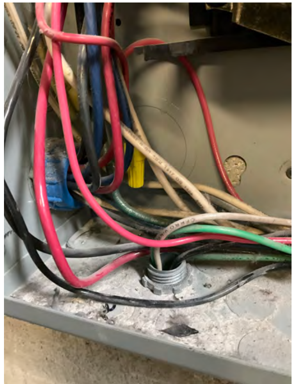
PHOTO-08 Branch Circuits
