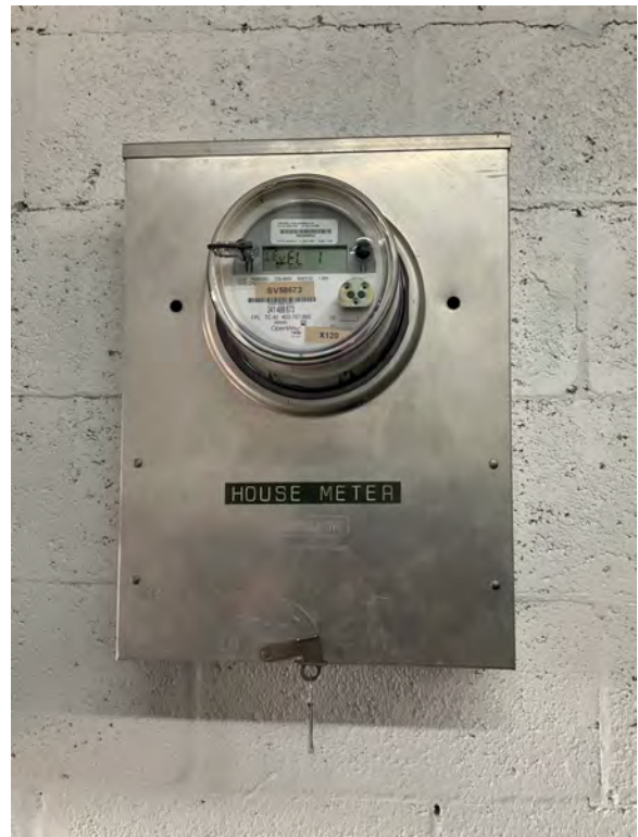
PHOTO-04 Metering Equipment
