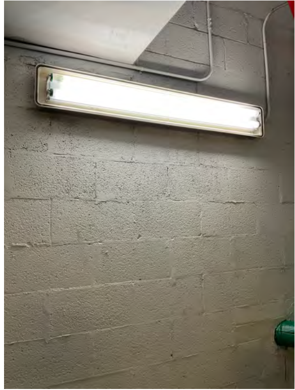
PHOTO-18 Existing Emergency Lighting
