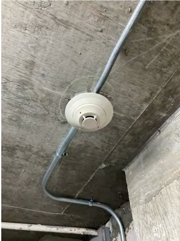
PHOTO-21 Existing Smoke Detectors
