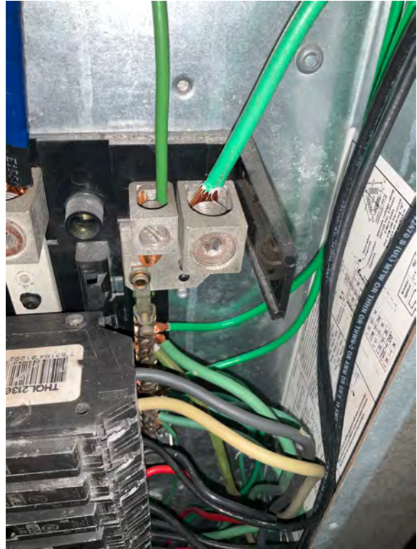
PHOTO-10 Branch Circuit Equipment Grounding System
