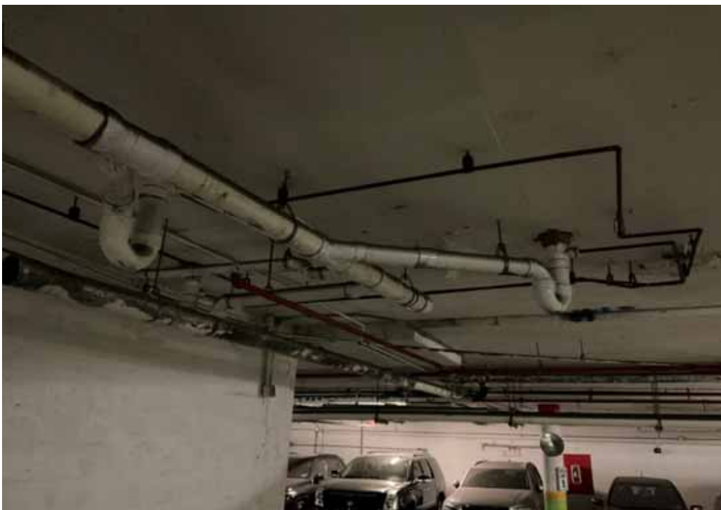
Plumbing Lines - Garage
