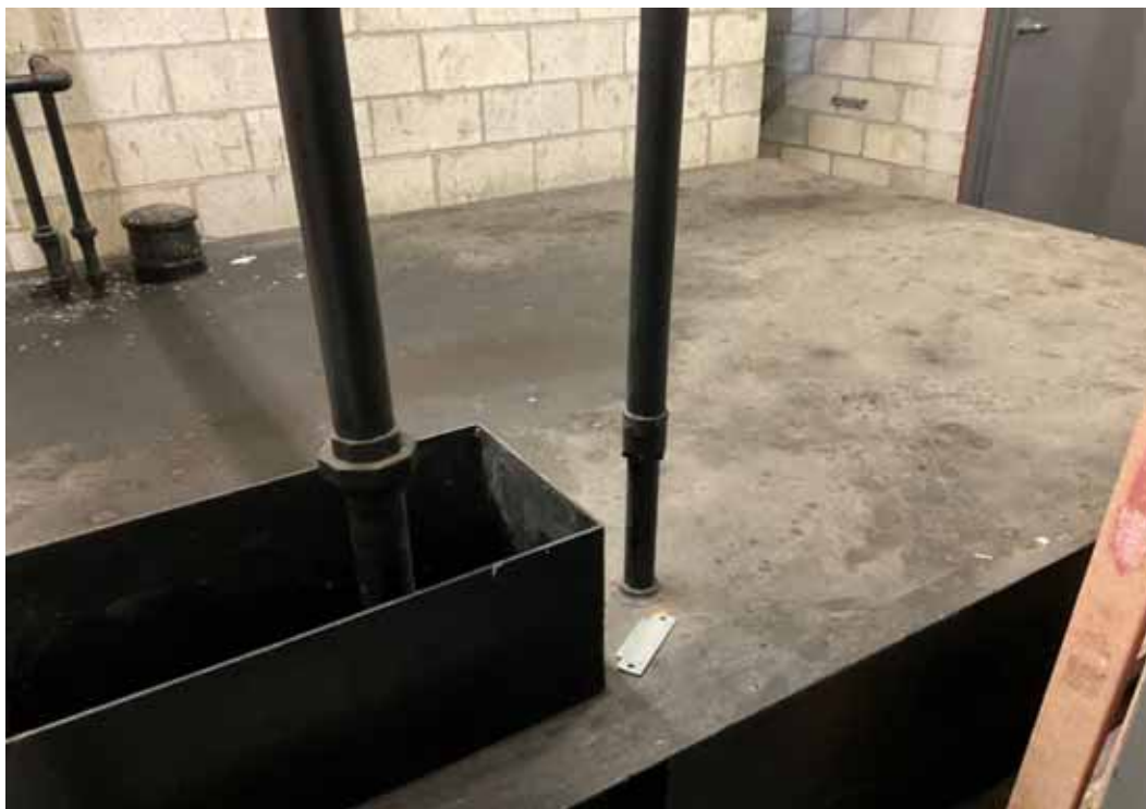
Generator Fuel Tank
