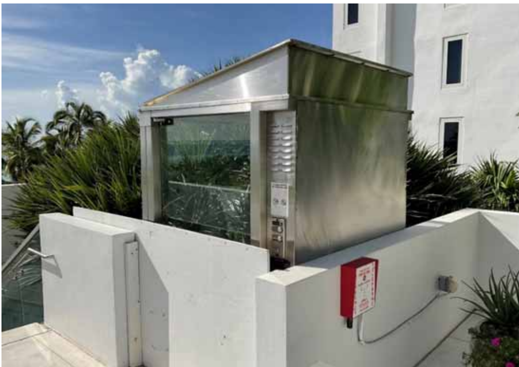
Main Pool Elevator
