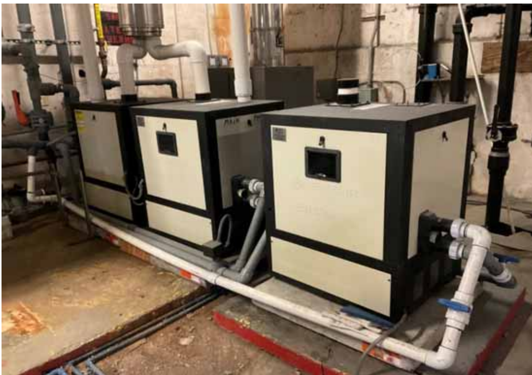
Main Pool Heater
