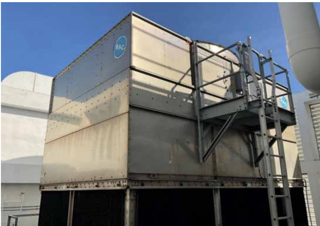
A/C Cooling Tower #4
