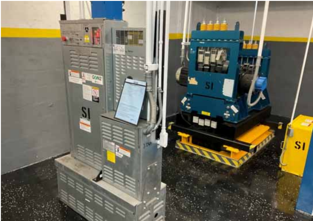
Elevator Equipment - South
