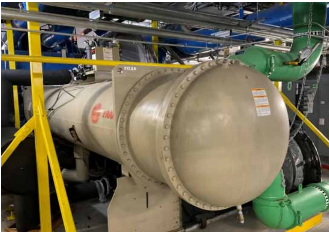
A/C Chiller Trane
