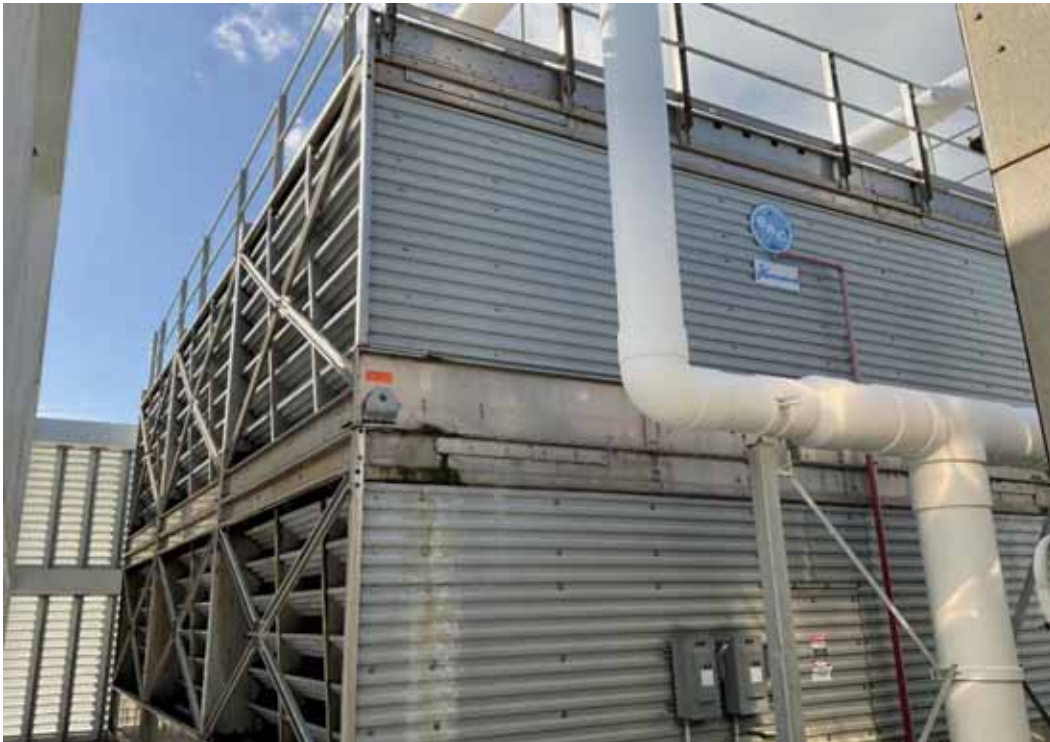
A/C Cooling Tower #1-3
