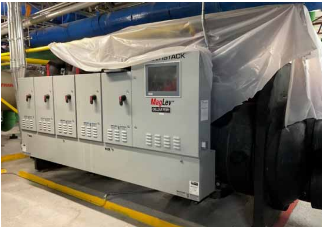
A/C Chiller 990 Tons
