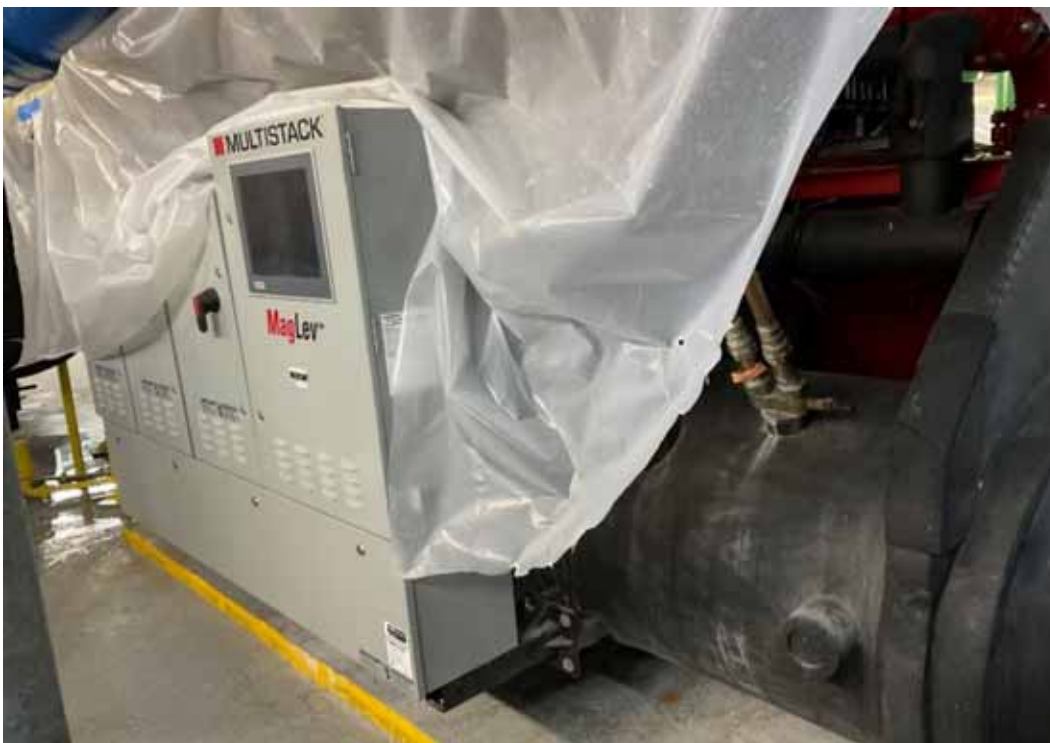
A/C Chiller 600 Tons
