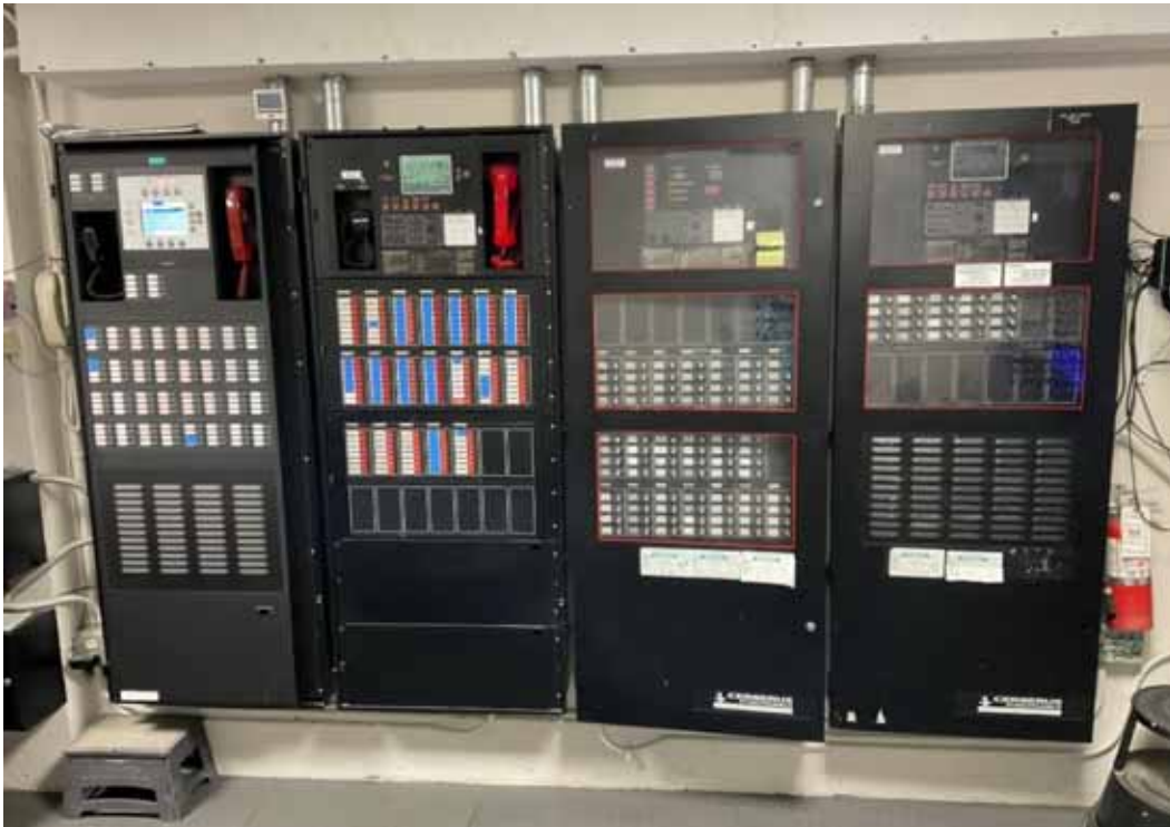
Fire Alarm Control Panel
