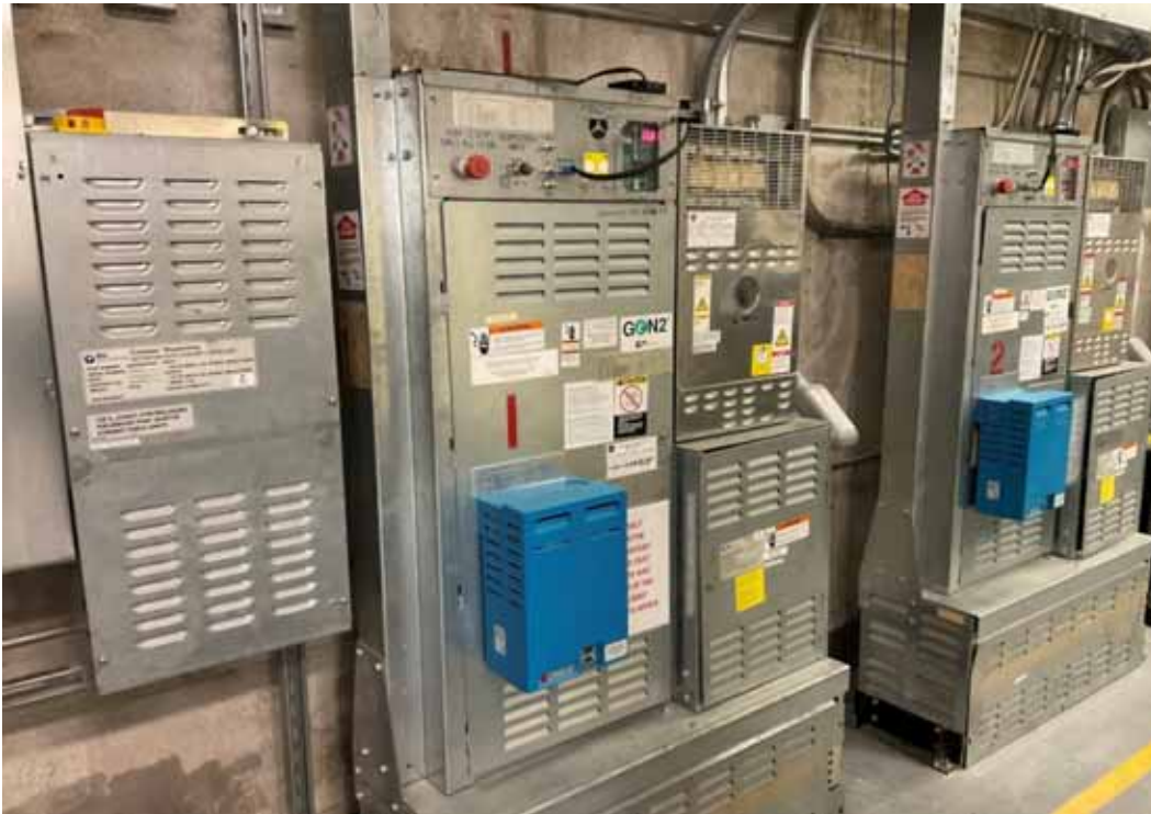
Elevator Equipment - North
