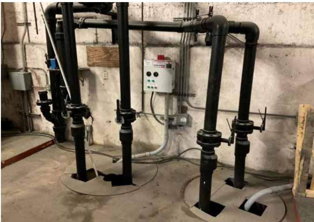
Sump Pumps - Garage
