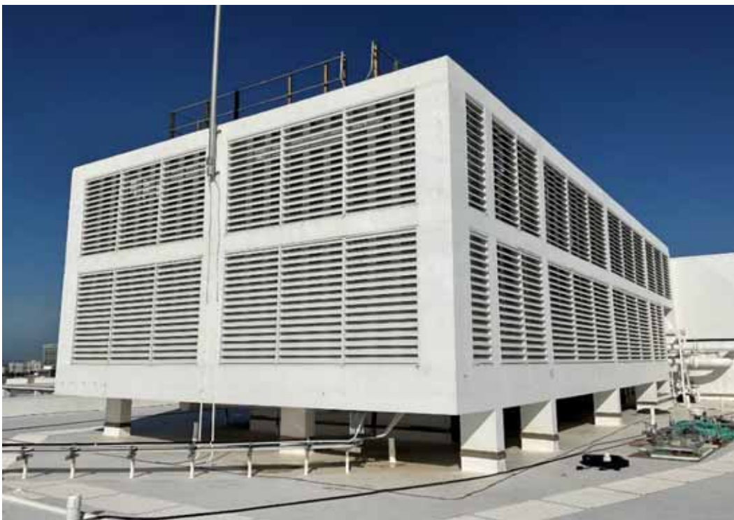
A/C Cooling Tower Surround
