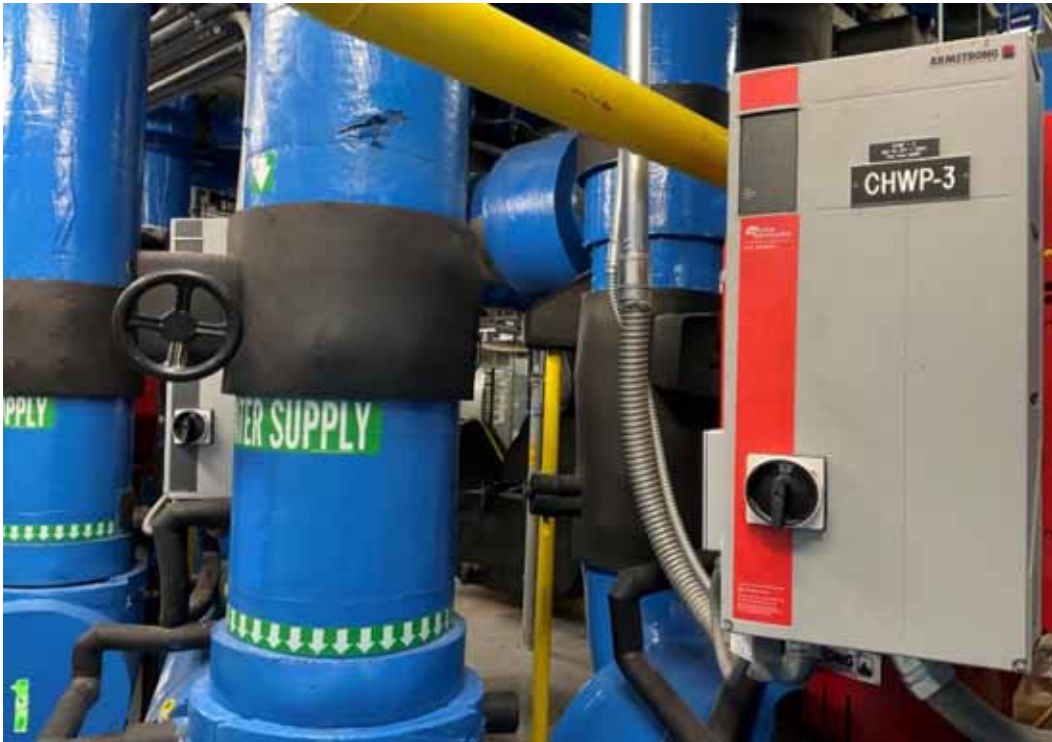
A/C - CHWP Pumps/Motors
