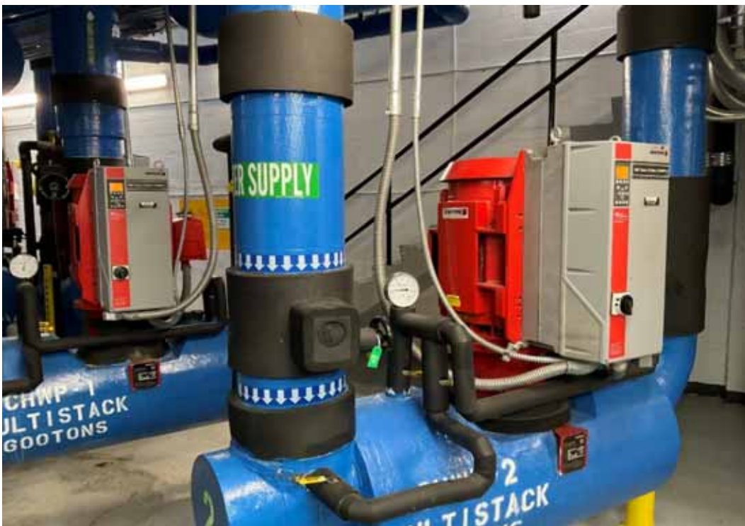
A/C - CHWP Pumps/Motors (Roney)
