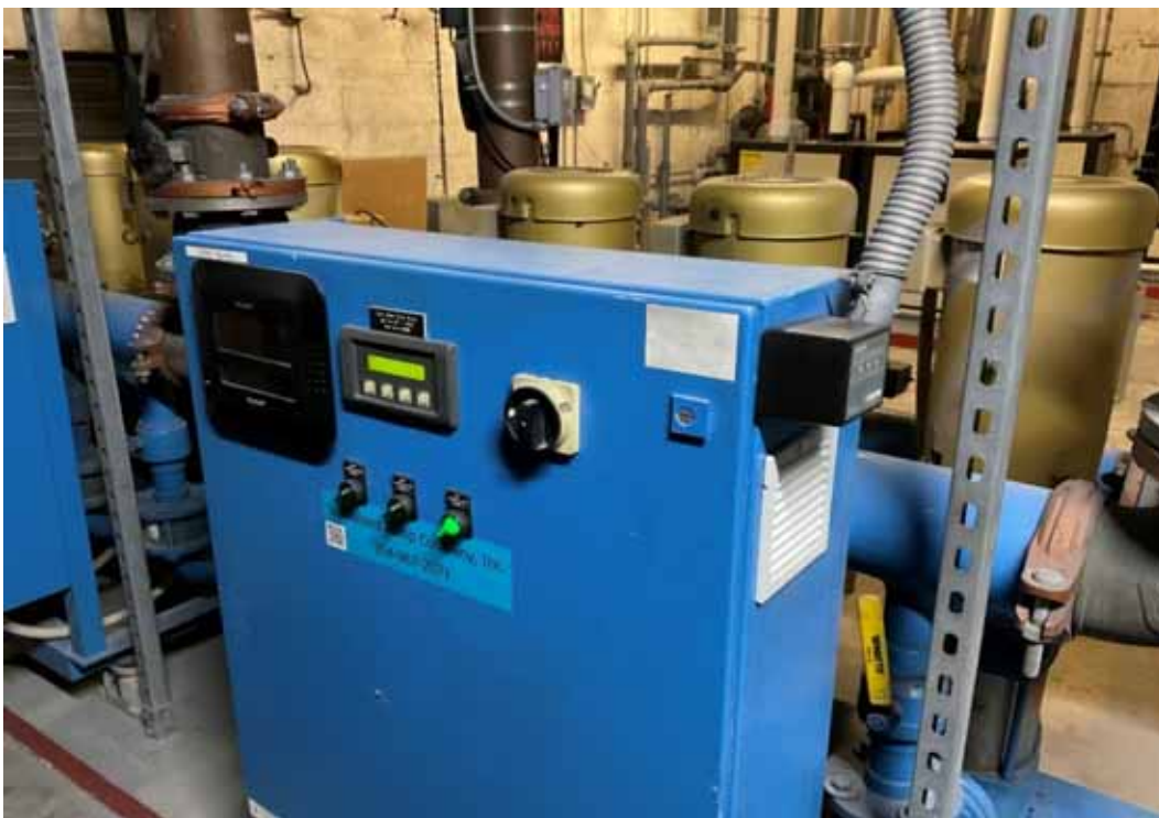
Domestic Water Pumps - Roney
