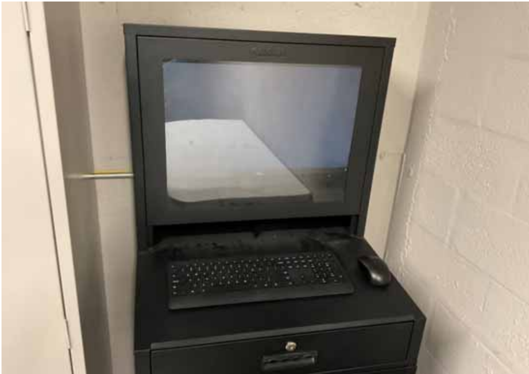
Building Management System
