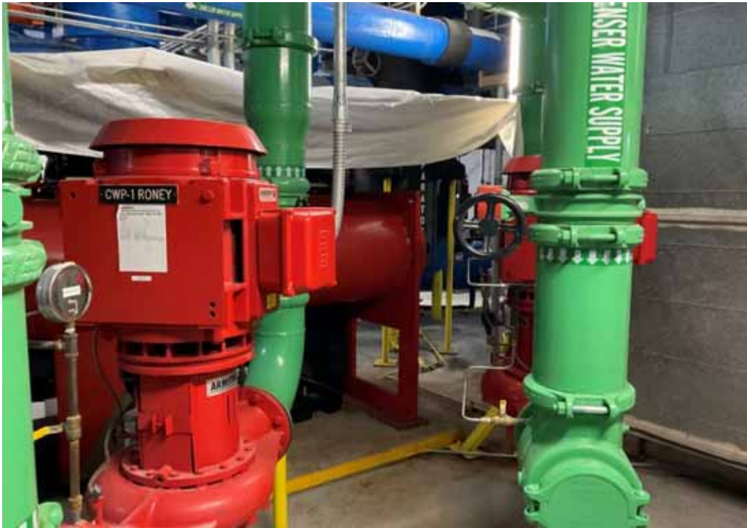
A/C - CWP Pumps/Motors (Roney)
