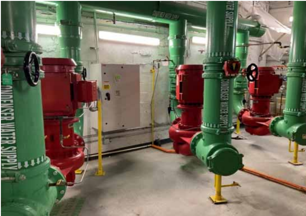
A/C - CWP Pumps/Motors
