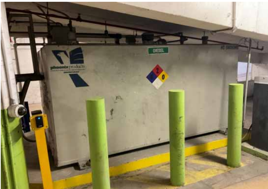
Generator Fuel Tank
