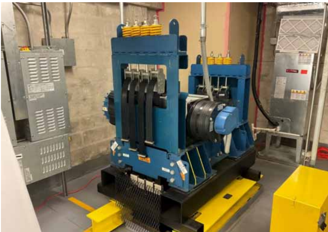
Elevator Equipment - North
