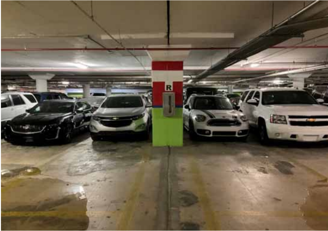
Expansion Joint - Garage
