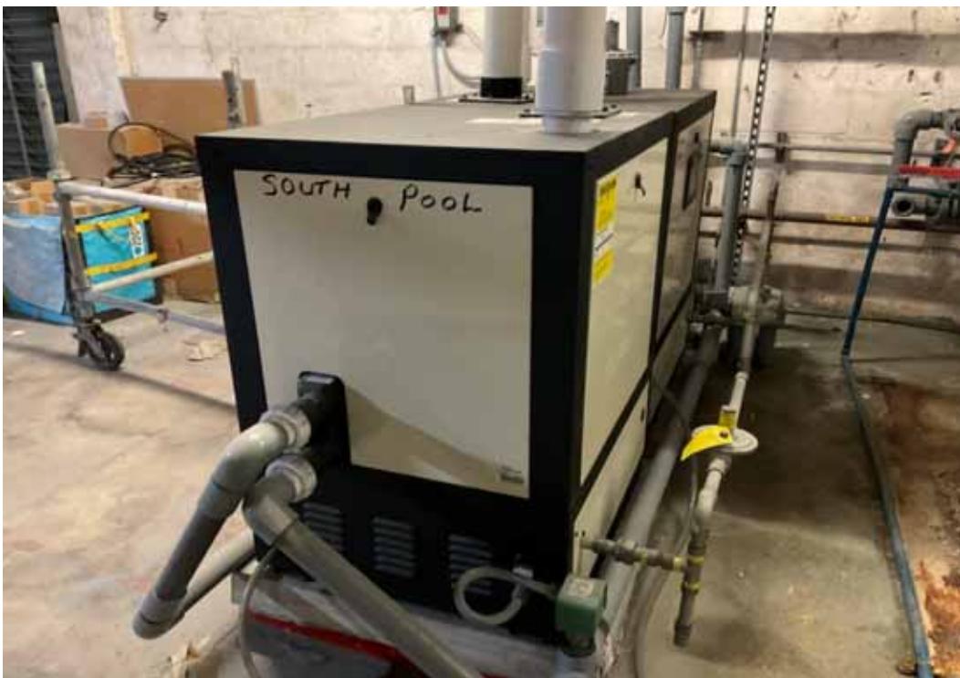
South Pool Heater
