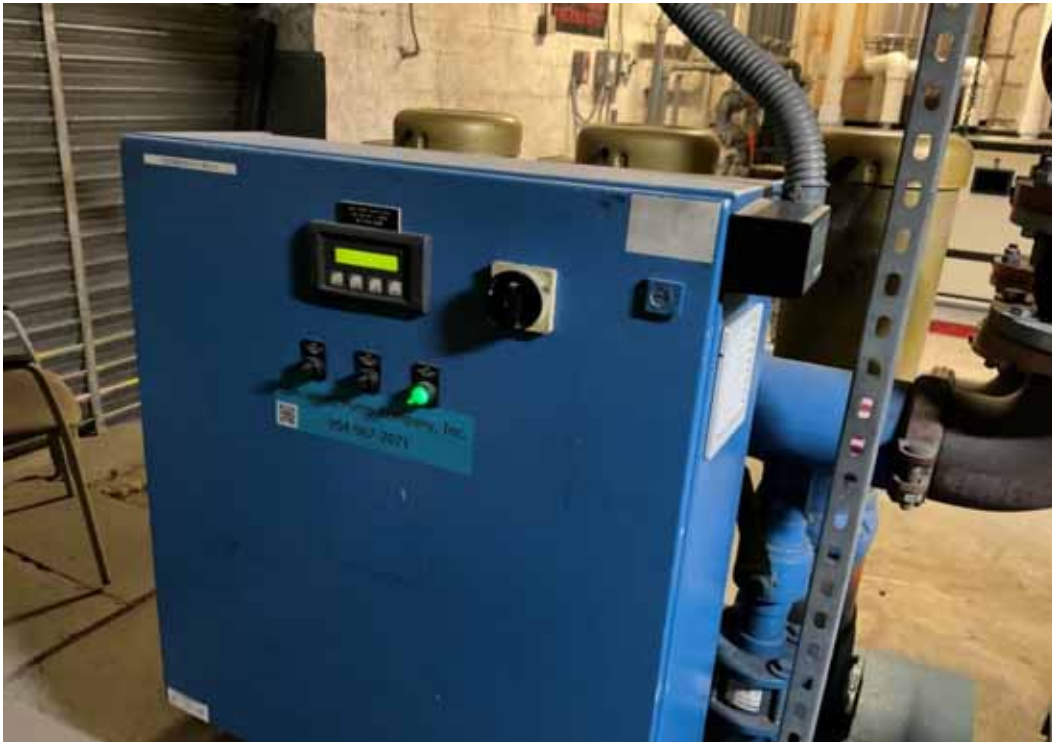
Domestic Water Pumps - Perry
